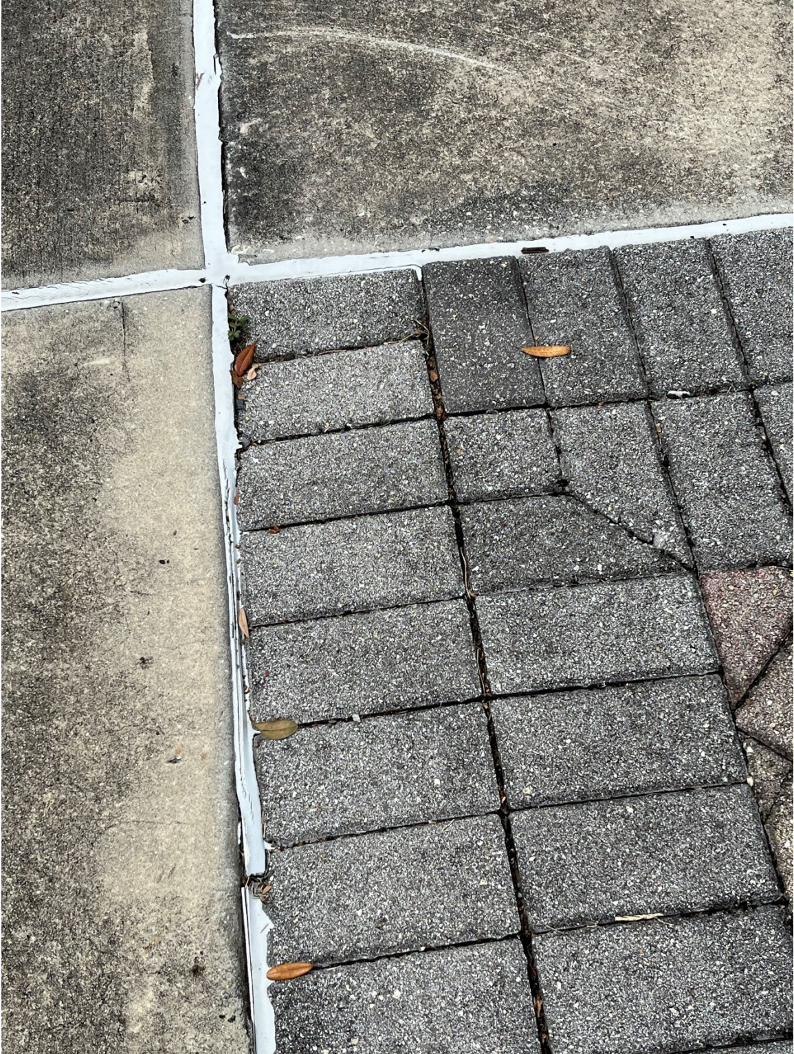
Photo 34 - Paver Base Failure
