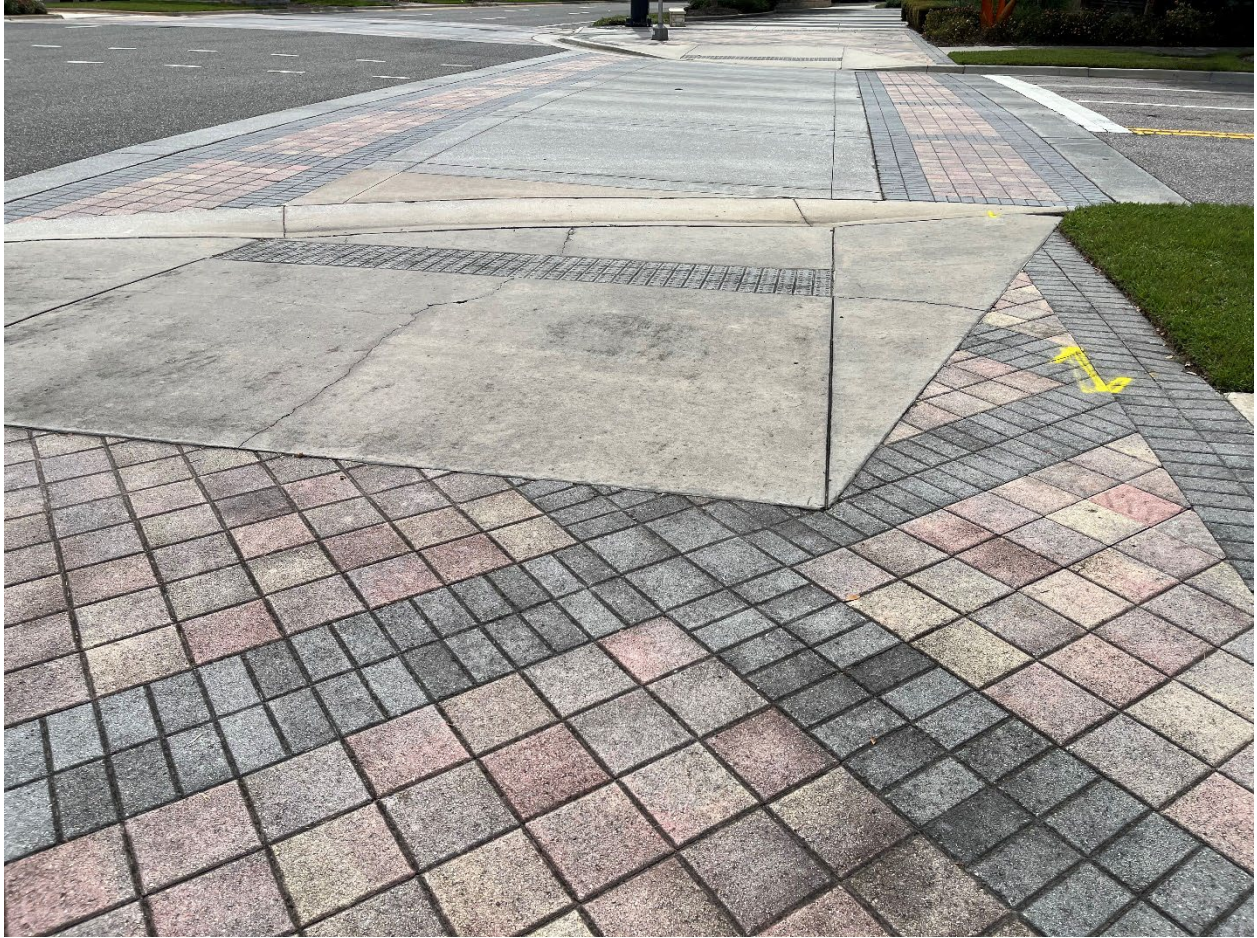
Photo 48 - Surficial Concrete Cracks in Handicap Ramp
