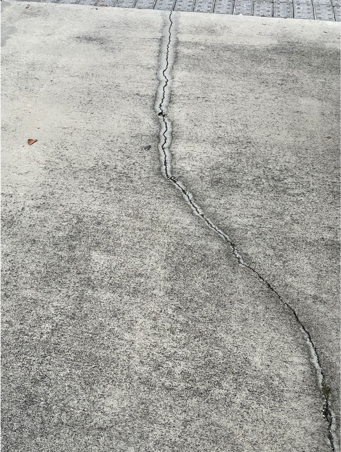
Photo 39 – Surficial Concrete Cracks in Median Strip
