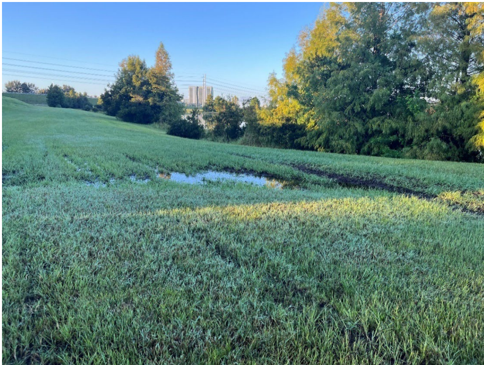
Photo 81 – Poor Drainage in NE Corner Berm
