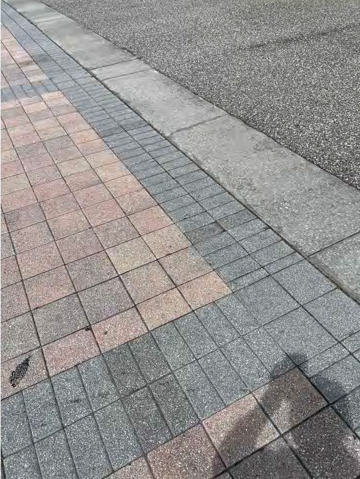
Photo 101 – Cracked Pavers – Minor Settling
