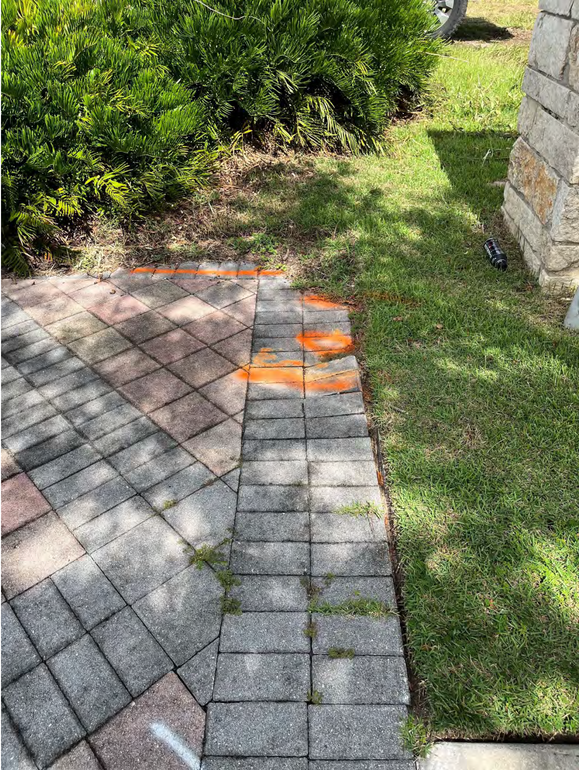
Photo 69 - Paver Base Failure
