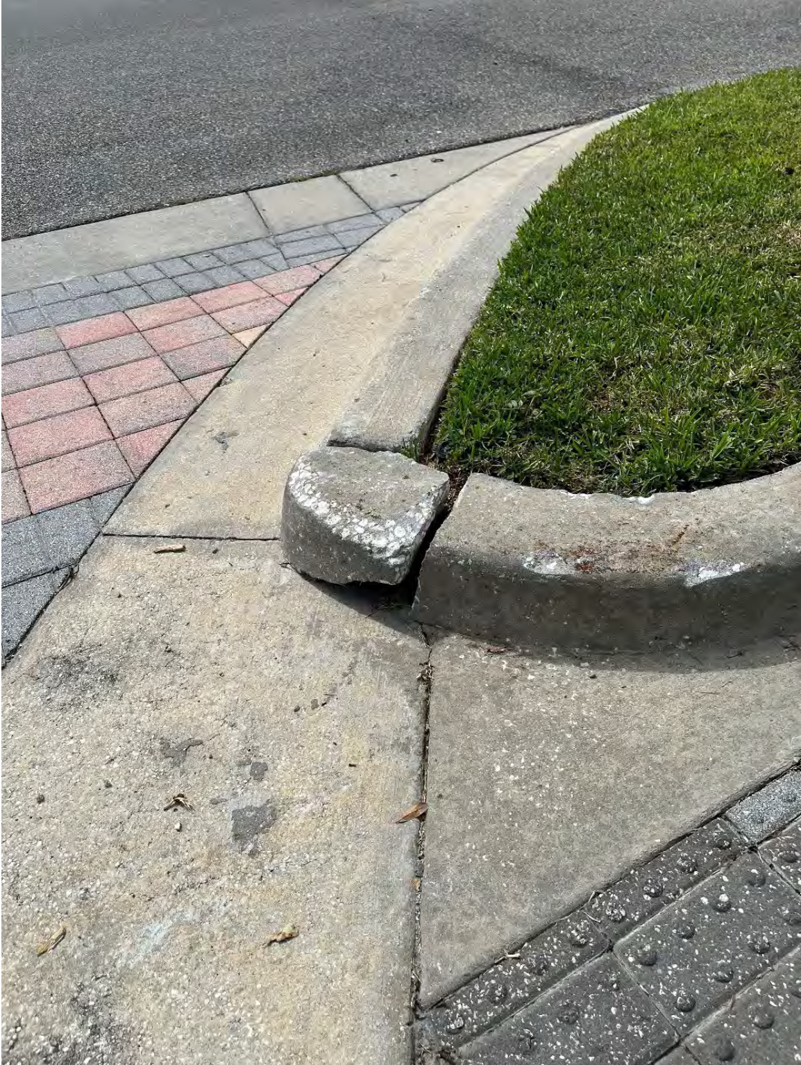
Photo 116 – Broken Concrete Curb
