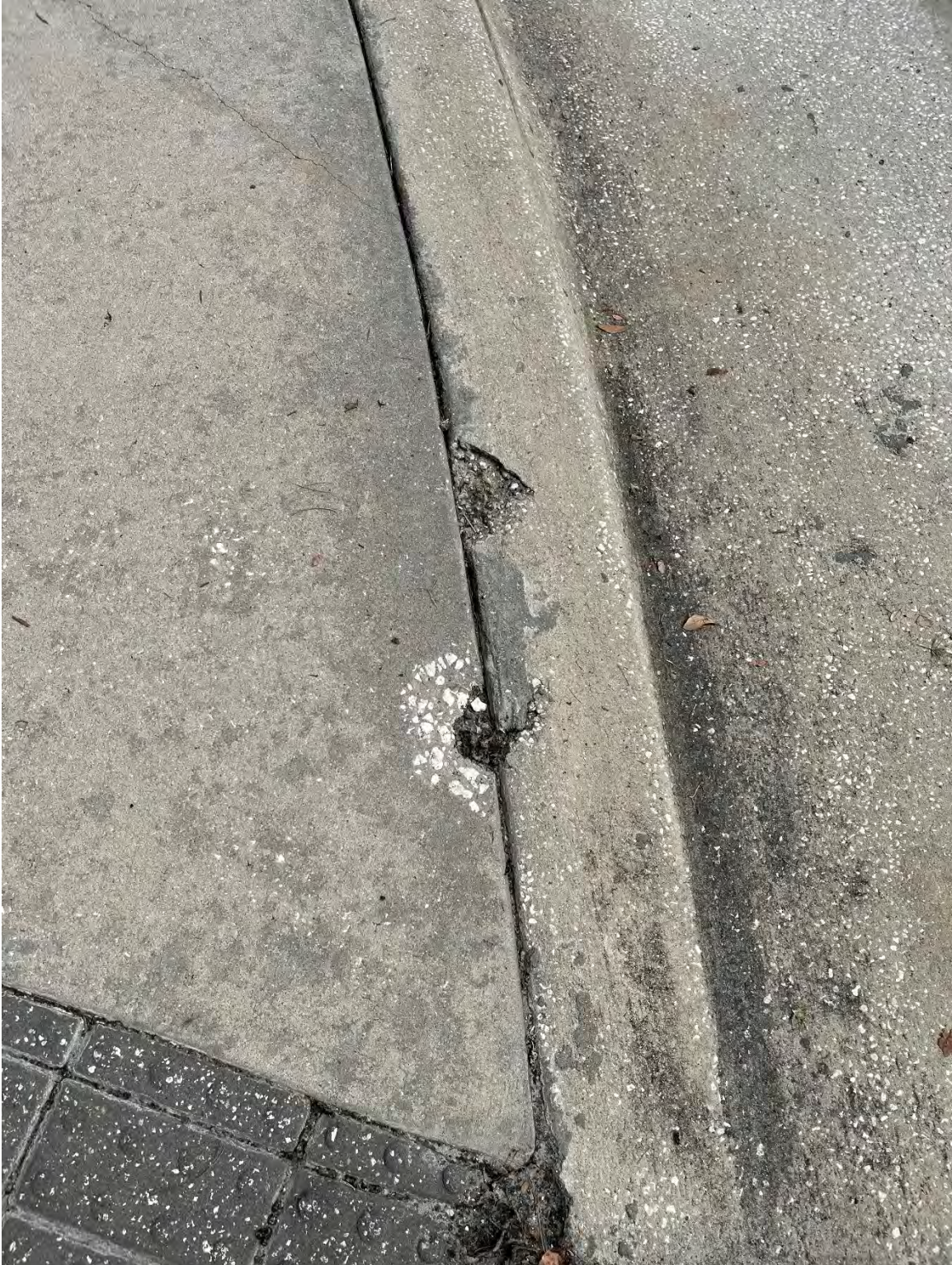
Photo 24 - Cracked Concrete in Handicap Ramp
