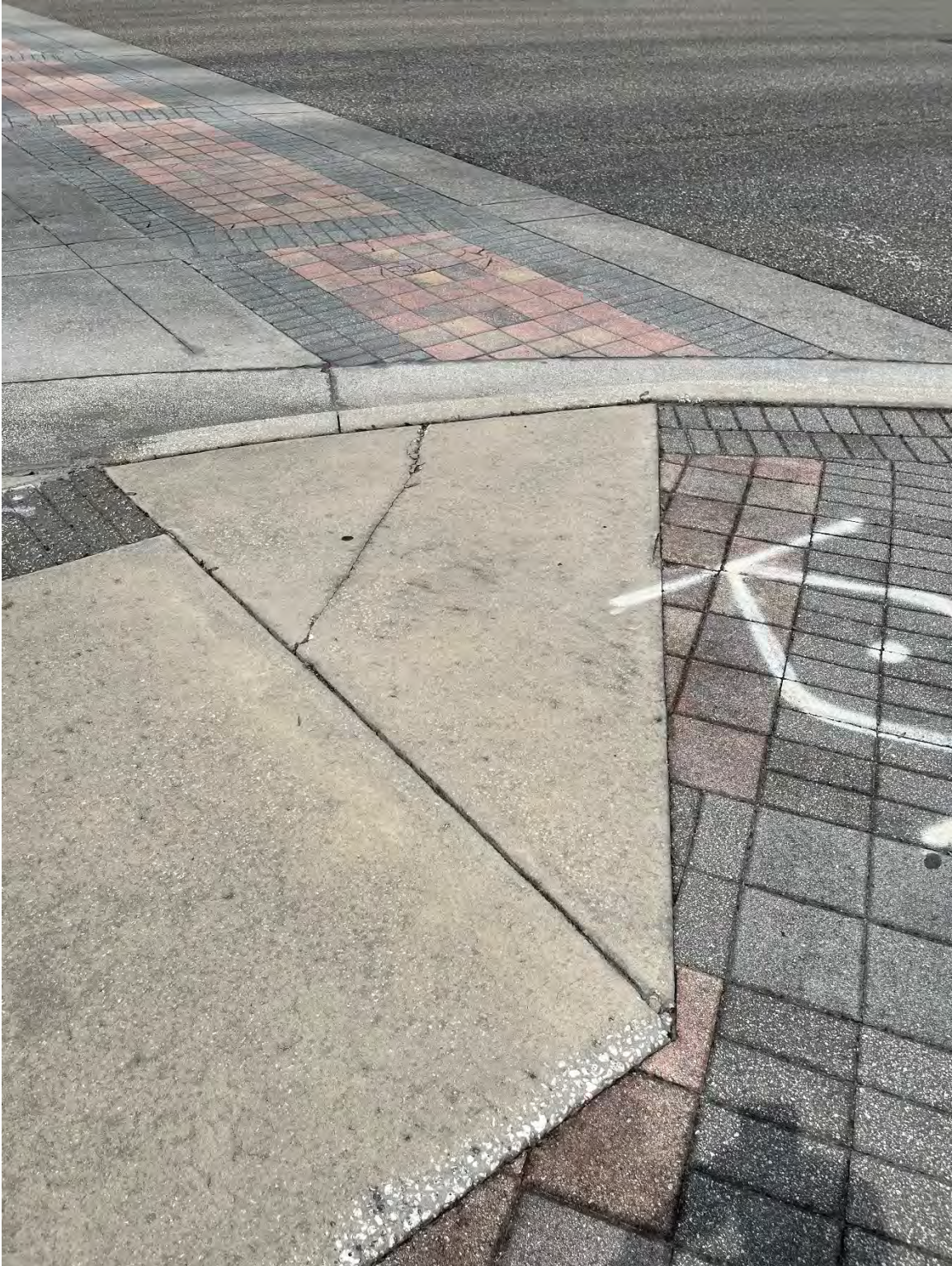
Photo 15 – Surficial Concrete Crack in Handicap Ramp
