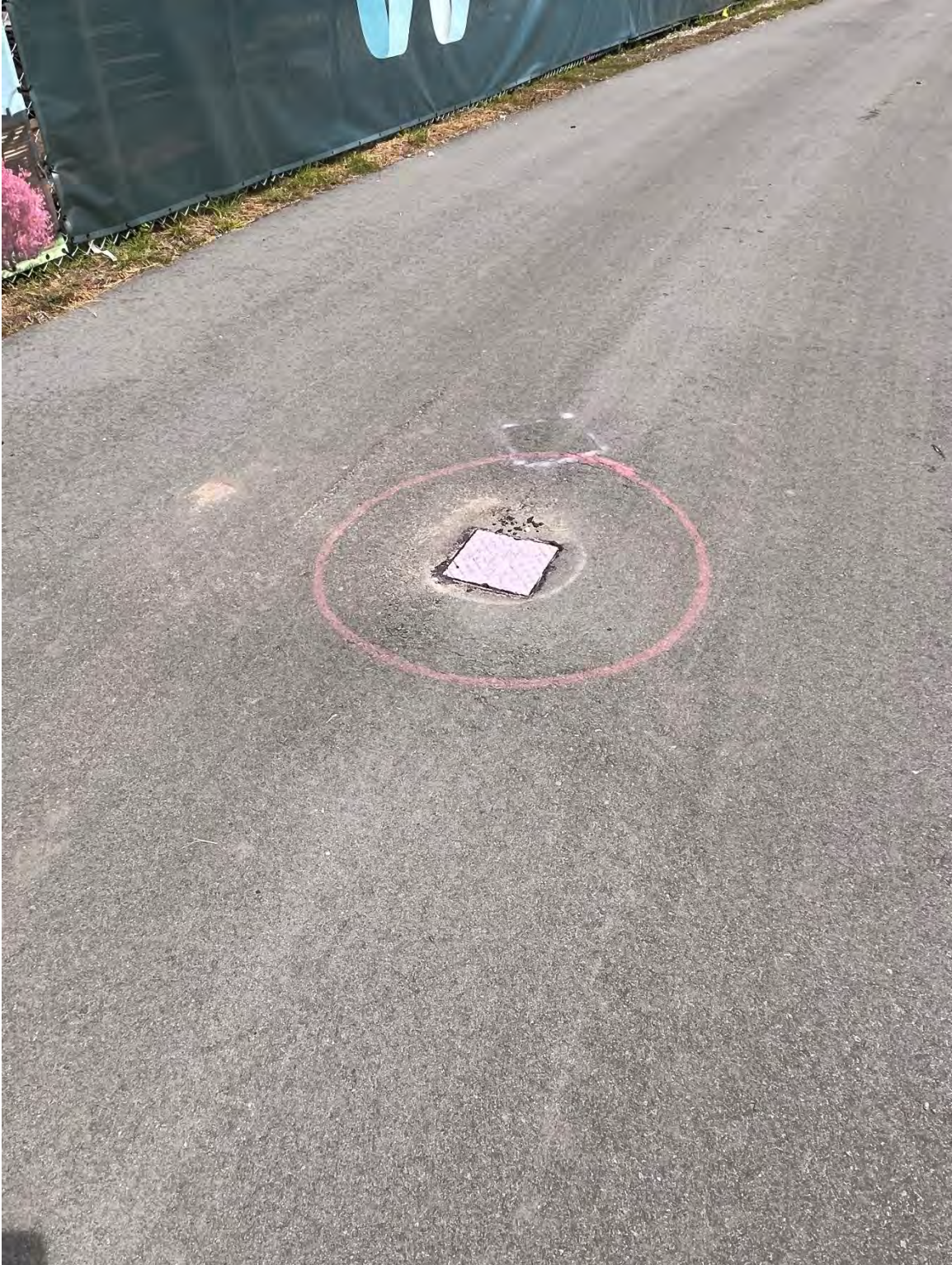
Photo 6 – Sunken Reclaim Water Meter
