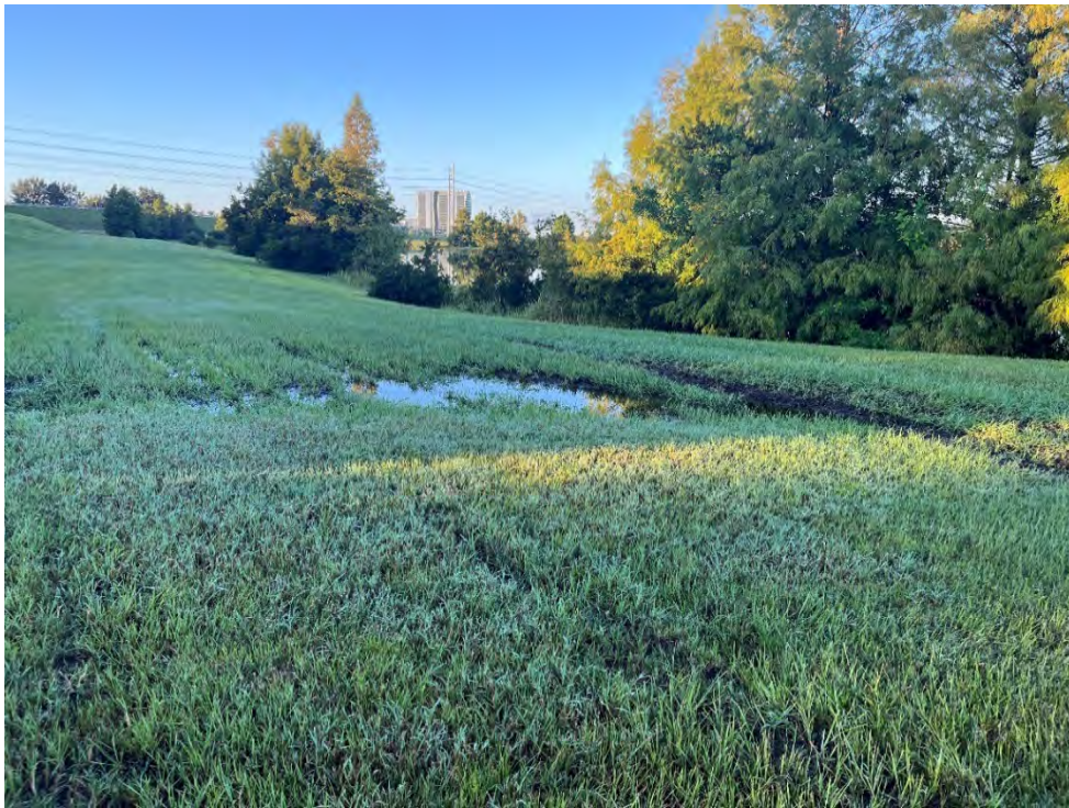
Photo 81 – Poor Drainage in NE Corner Berm
