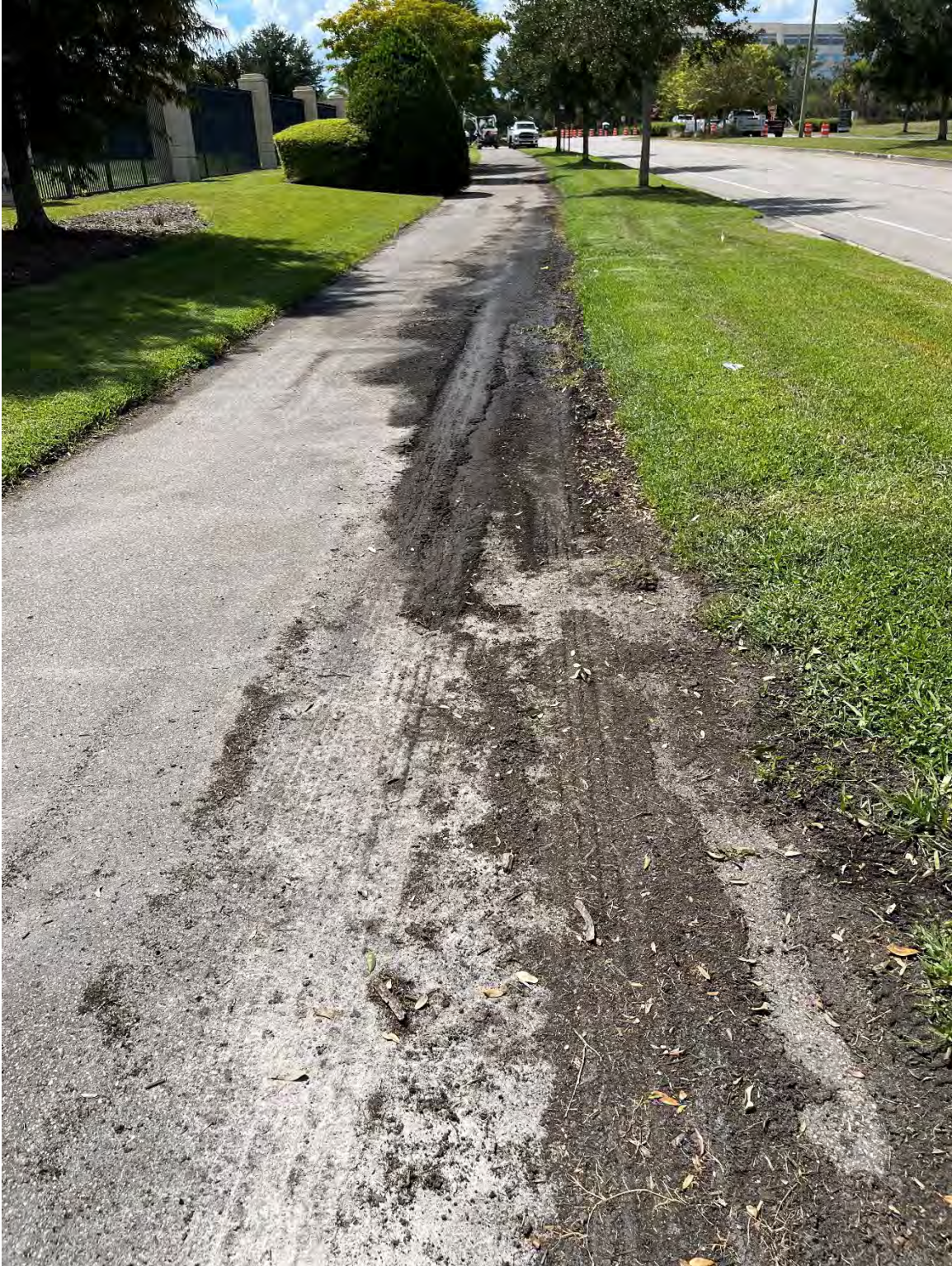
Photo 64 - Poor Drainage Area
