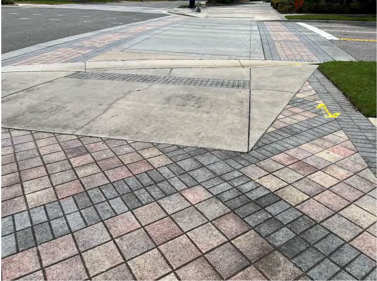
Photo 48 - Surficial Concrete Cracks in Handicap Ramp
