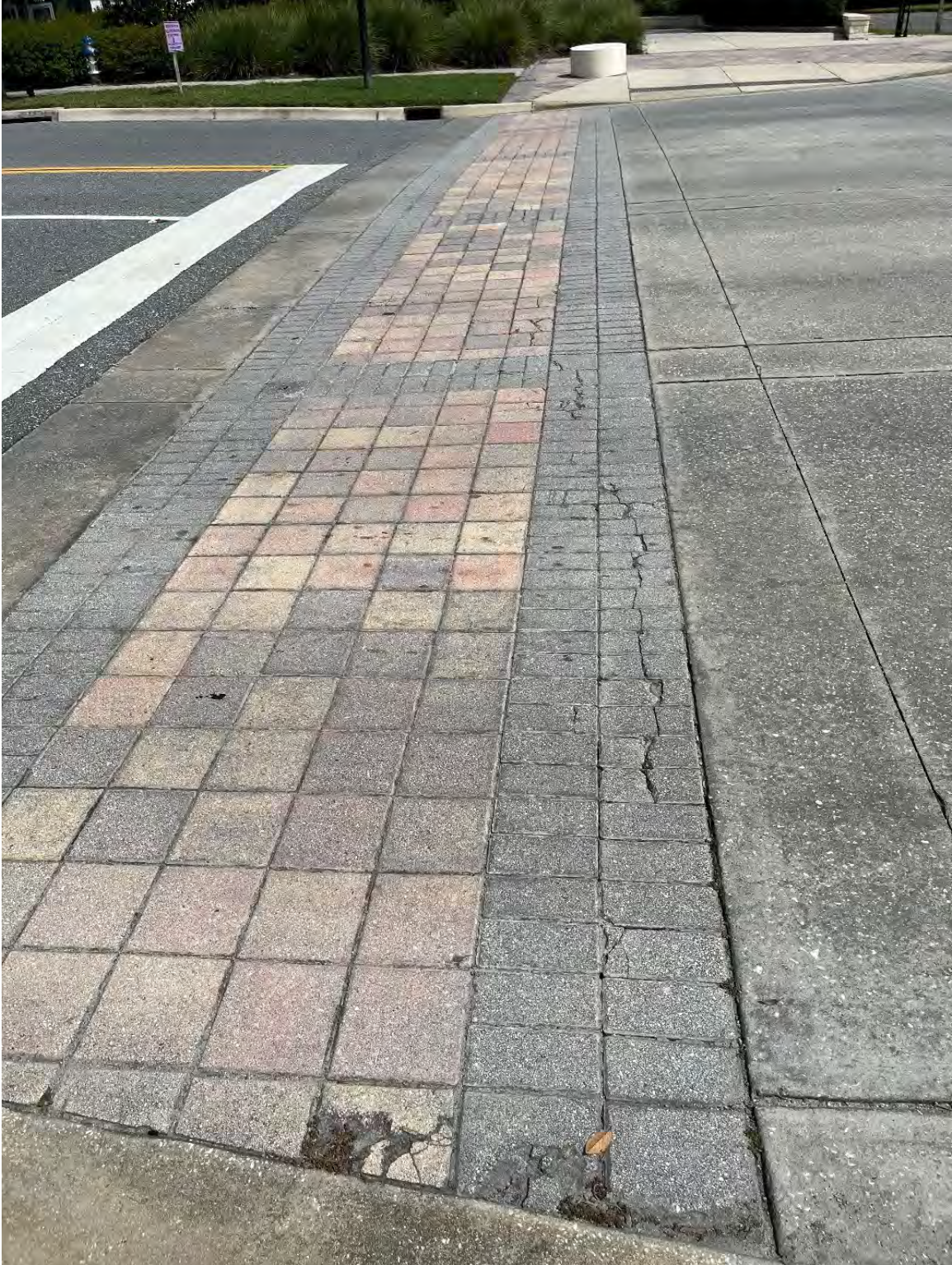
Photo 108 – Cracked and Broken Pavers – Some Settling
