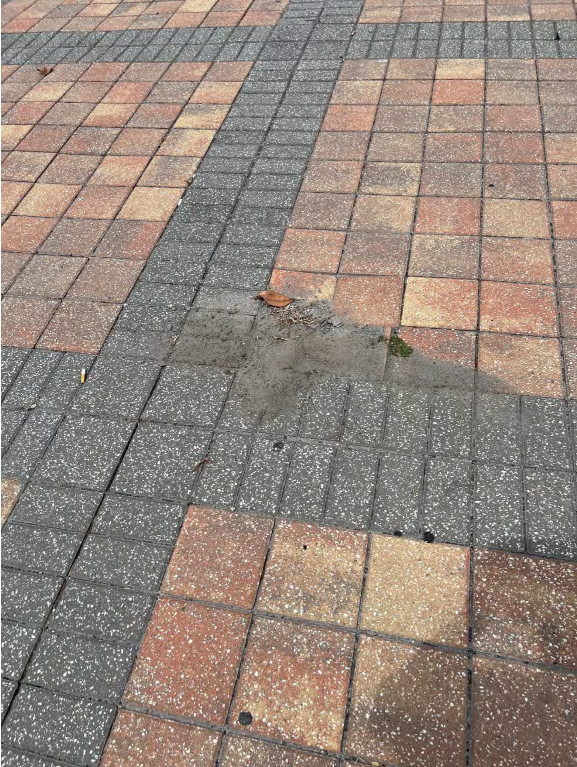
Photo 54 - Paver Base Failure in Median
