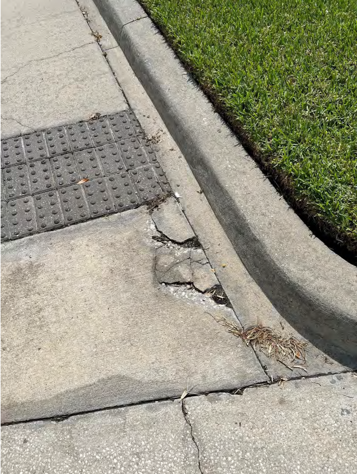
Photo 104 – Cracked Concrete – Some Settling
