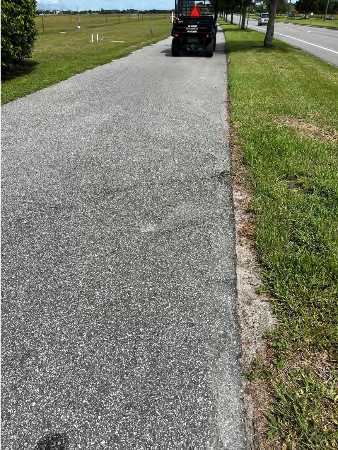
Photo 11 – Raveling Asphalt with Depression and Base Failure
