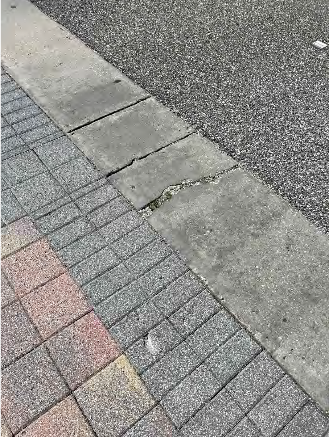
Photo 119 – Construction Entrance – Broken Concrete in Flush Curb
