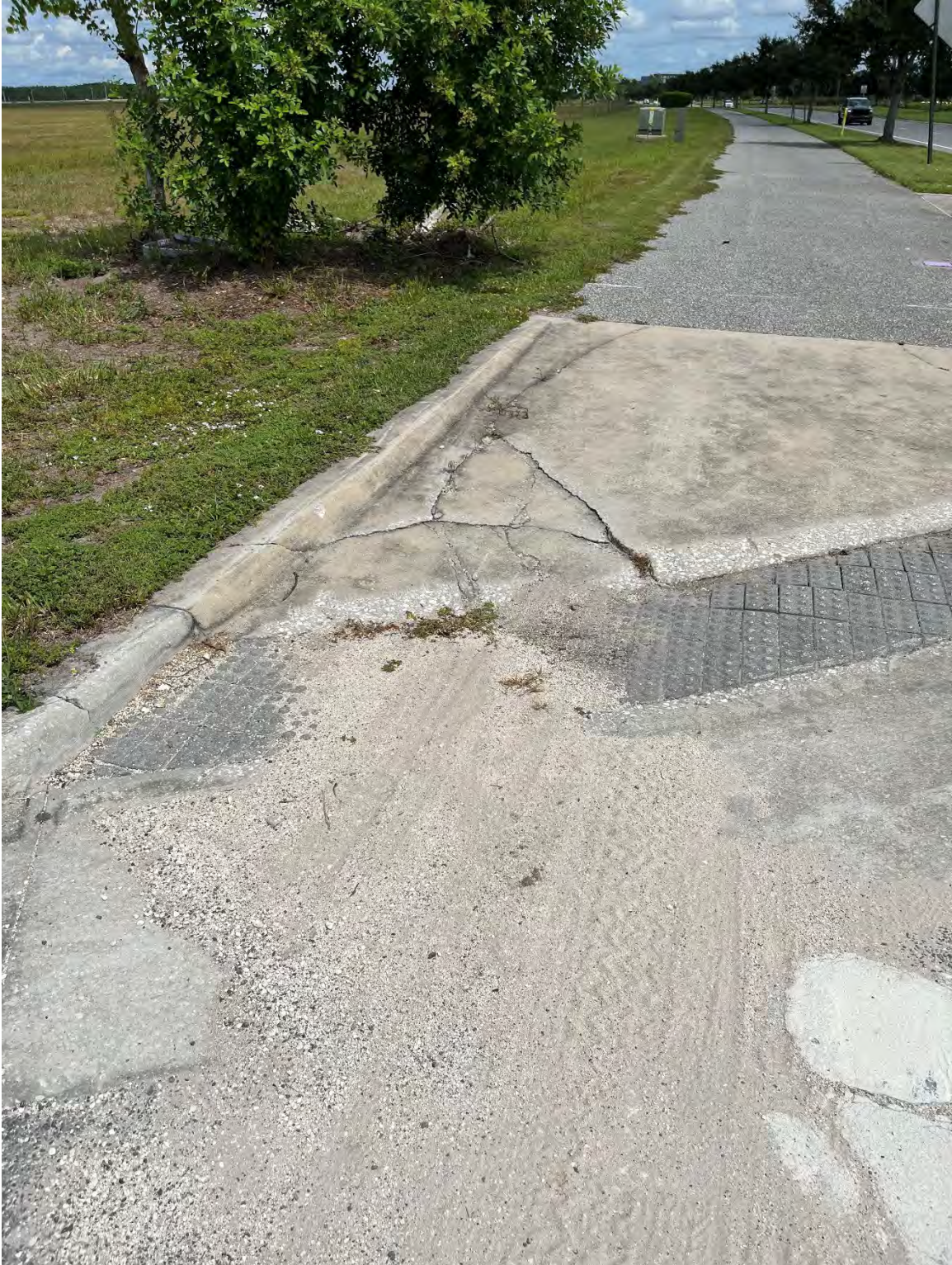
Photo 10 – Surficial Concrete Cracks in Handicap Ramp on East and West Side of Driveway Apron
