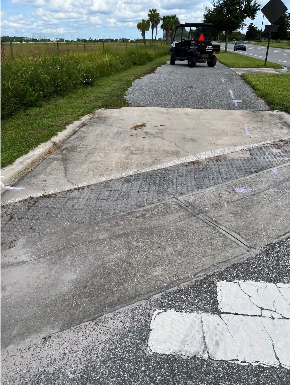
Photo 13 – Surficial Concrete Cracks in Handicap Ramp on East and West Side of Driveway Apron
