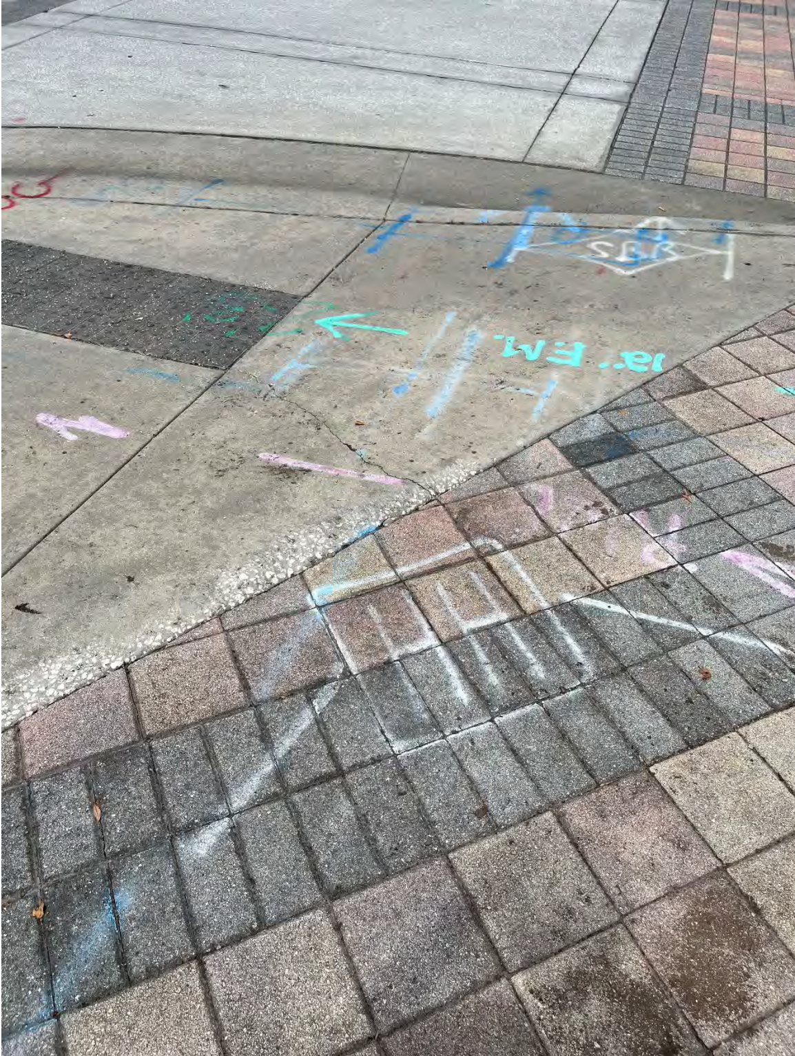
Photo 51 – Surficial Concrete Crack in Handicap Ramp
