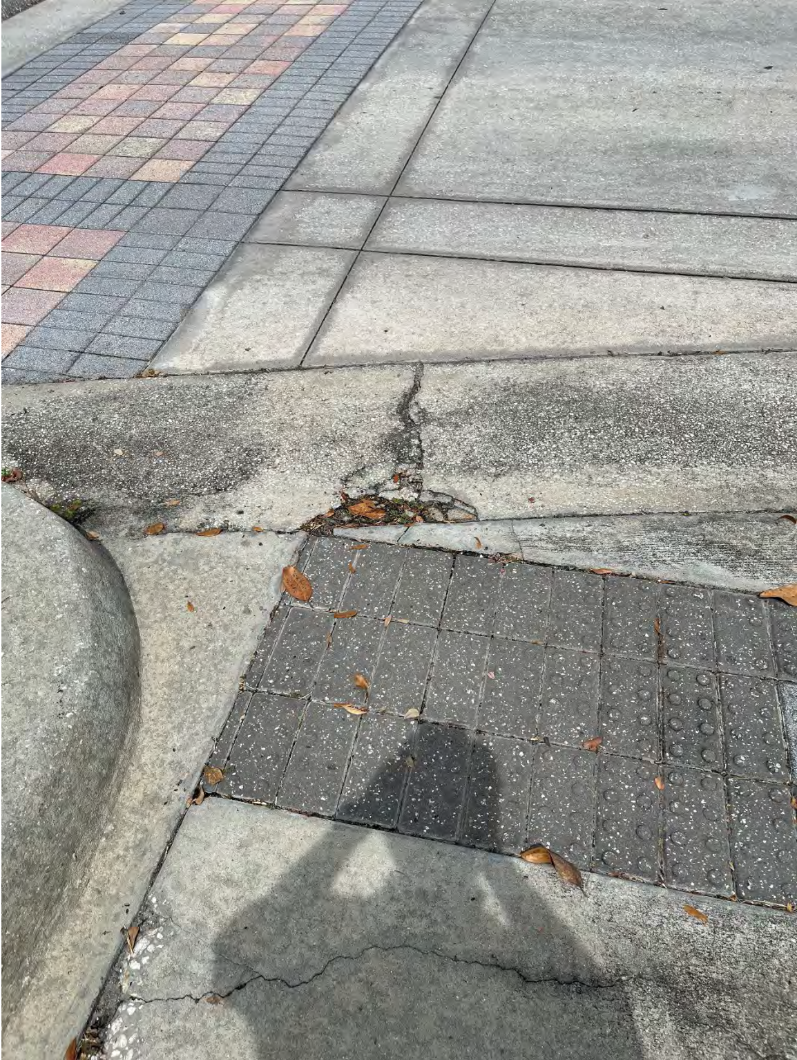
Photo 30 - Cracked Concrete in East Median
