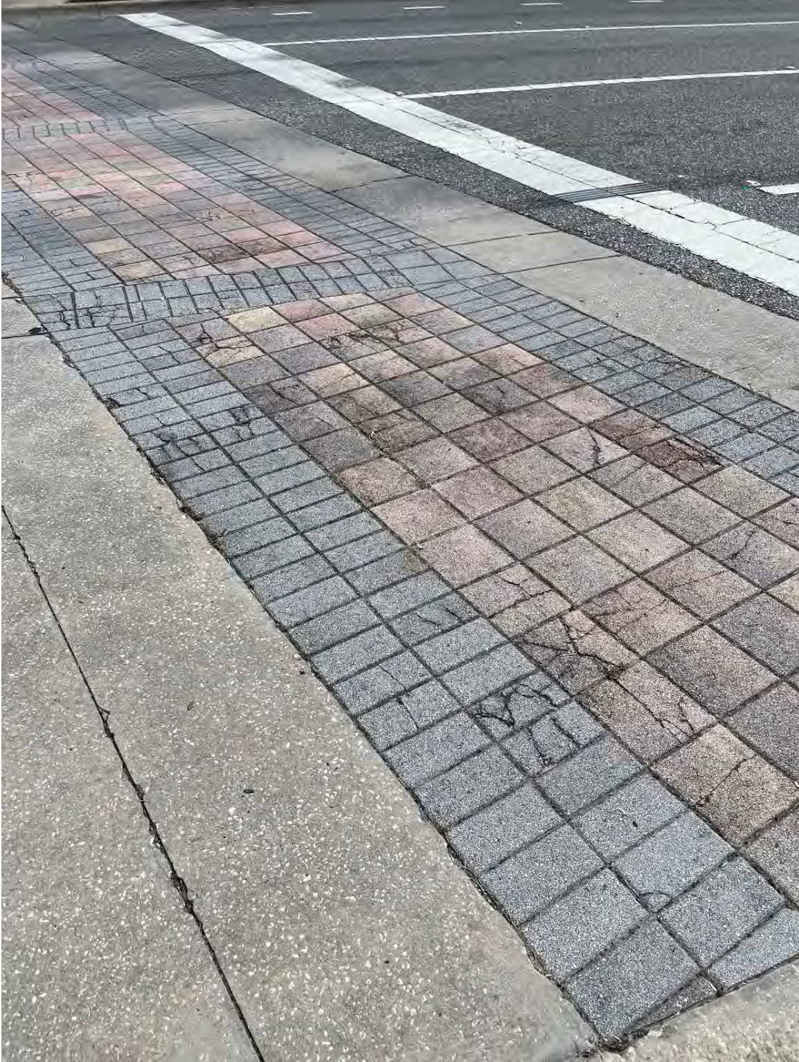
Photo 115 – Multiple Cracked Concrete – Pavers Settling – Broken Flush Curb
