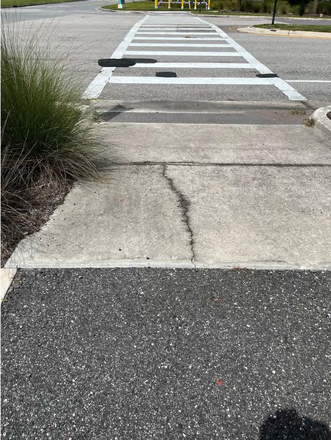
Photo 63 – Surficial Concrete Crack in Handicap Ramp
