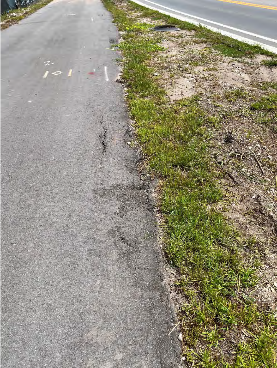
Photo 7 – Raveling Asphalt and Base Failure
