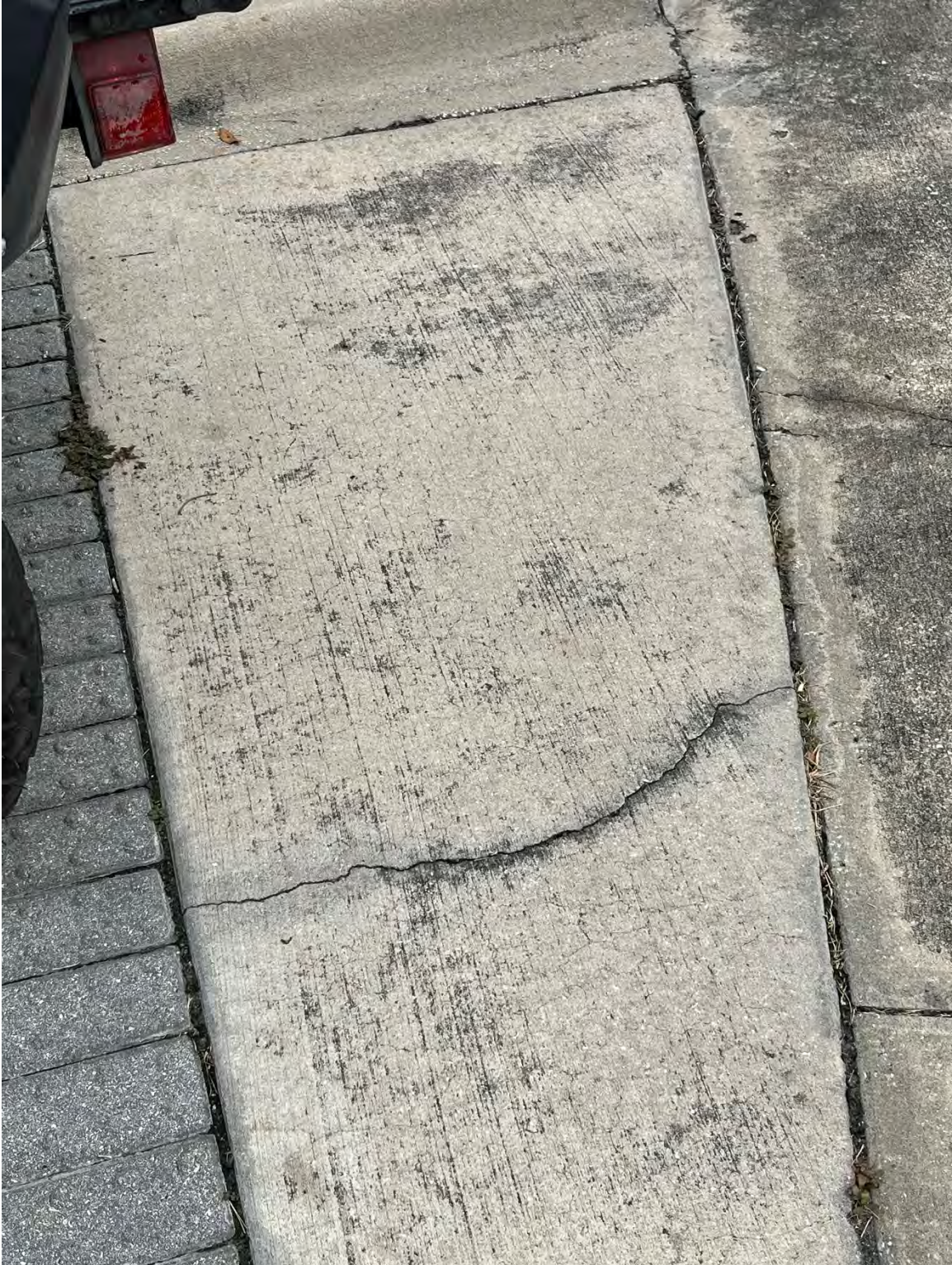
Photo 38 – Surficial Concrete Crack in Median Strip
