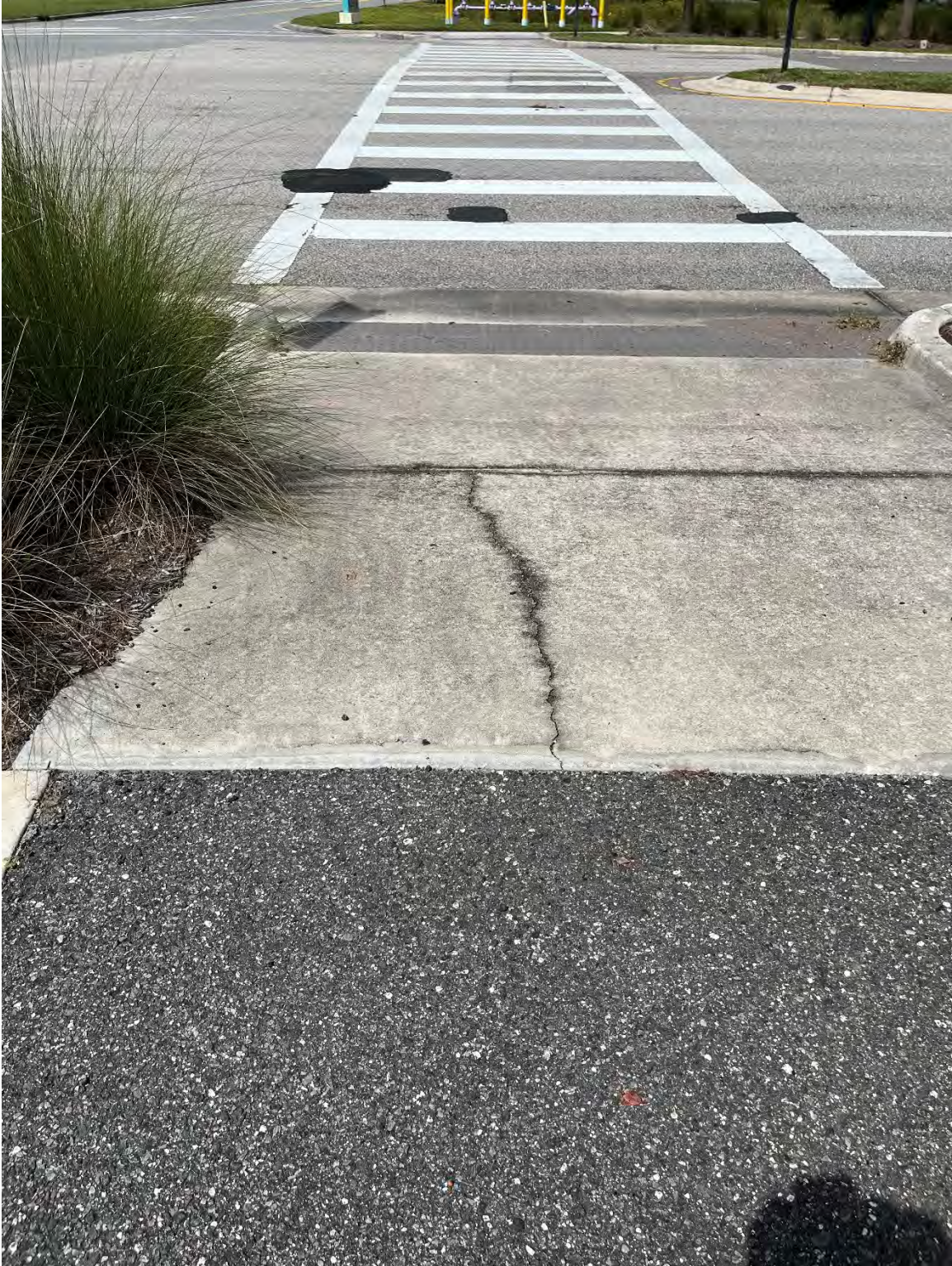
Photo 63 – Surficial Concrete Crack in Handicap Ramp
