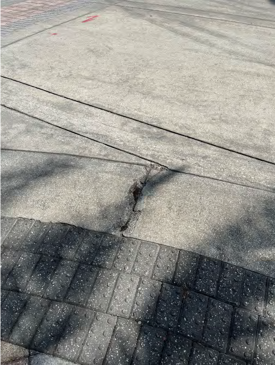
Photo 120 – Broken Concrete in Flush Curb
