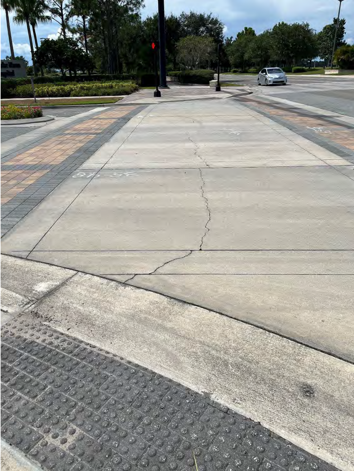
Photo 109 – Surficial Concrete Cracks - Multiple Cracked Pavers – Some Settling
