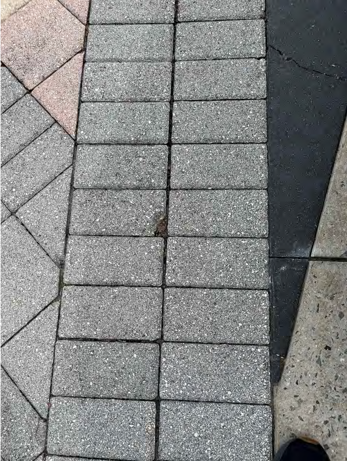
Photo 44 - Multiple Chipped Pavers
