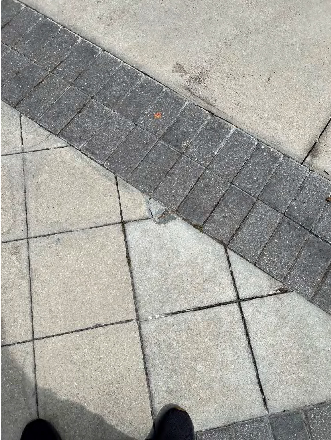
Photo 46 – Multiple Chipped Pavers
