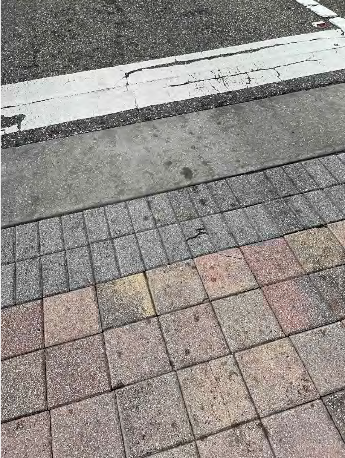
Photo 110 – Cracked Pavers – Some Settling
