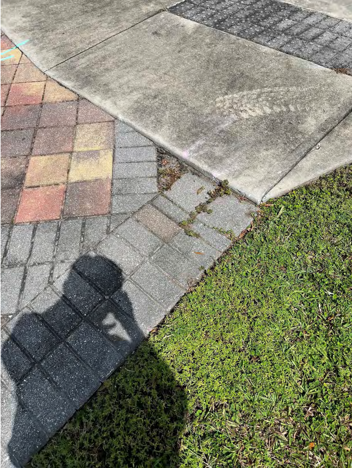
Photo 59 - Paver Base Failure
