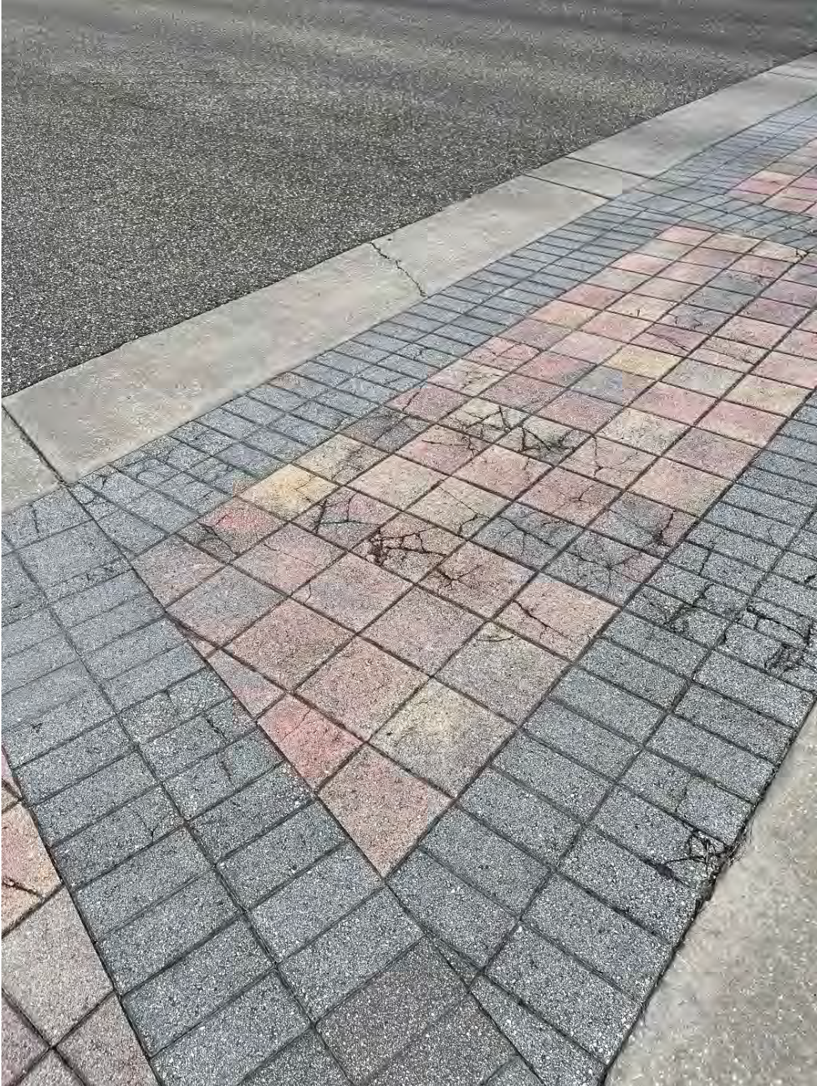
Photo 114 – Multiple Cracked Concrete – Pavers Settling – Broken Curb
