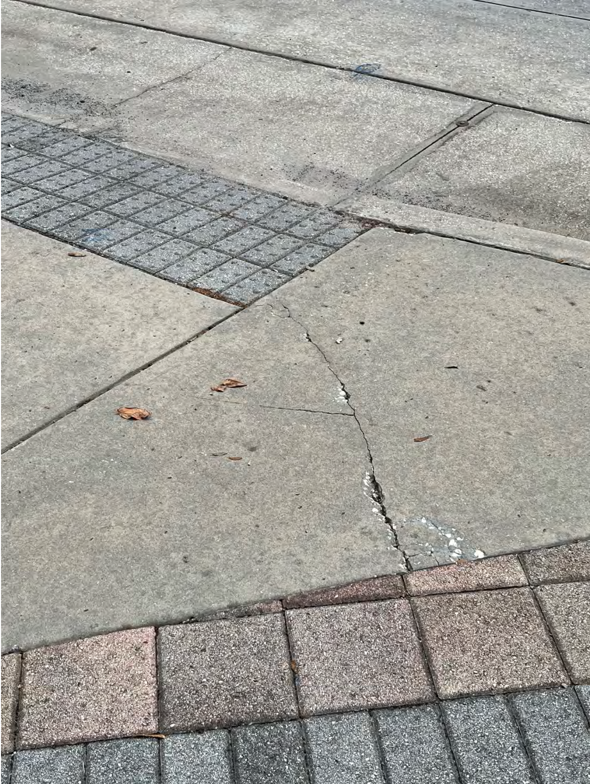
Photo 41 - Surficial Concrete Cracks in Handicap Ramp
