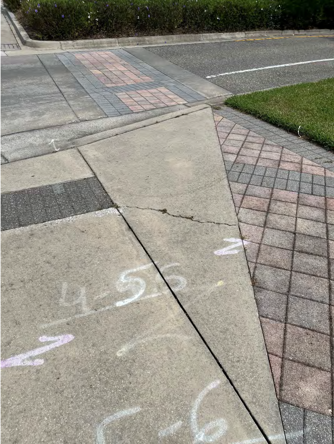
Photo 17 – Surficial Concrete Crack in Handicap Ramp
