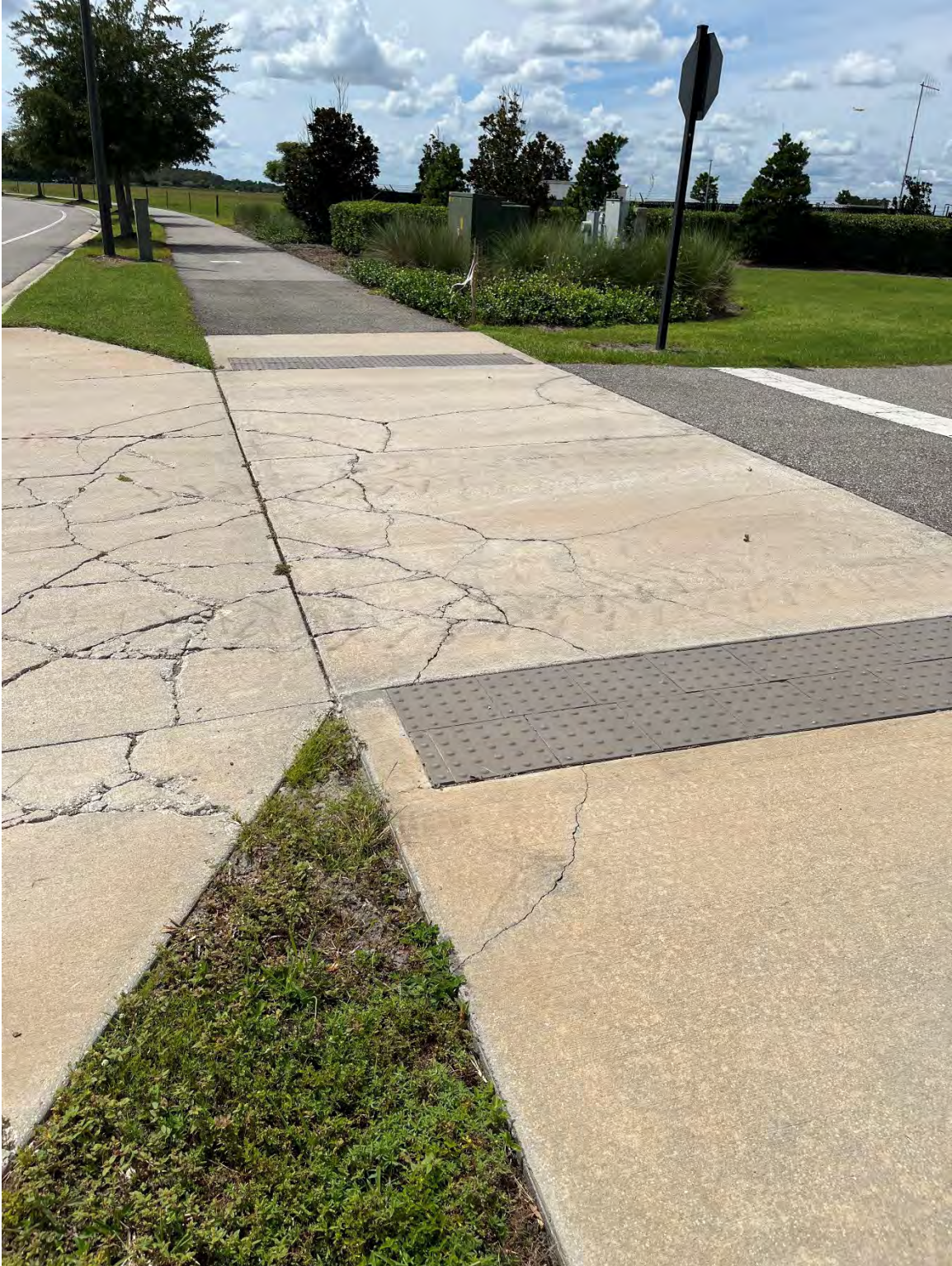
Photo 1 – Surficial Concrete Cracks in Trail and Driveway Apron
