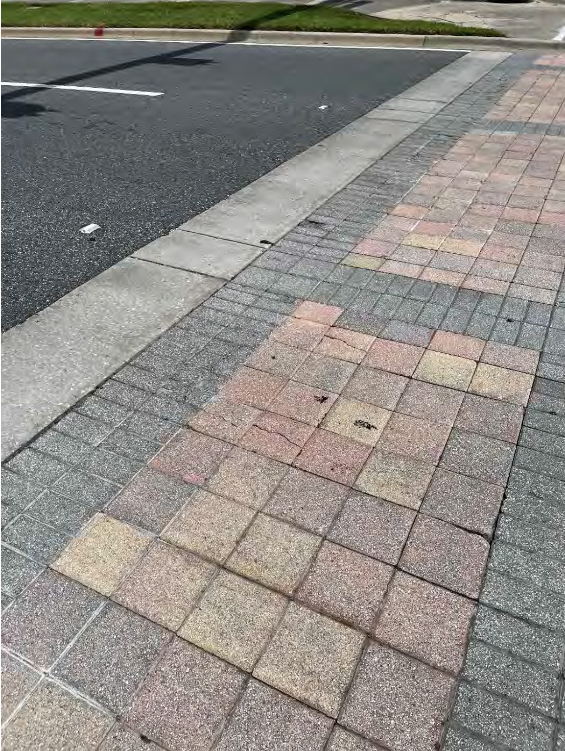
Photo 93 – Surficial Paver Cracks - Minor Settling
