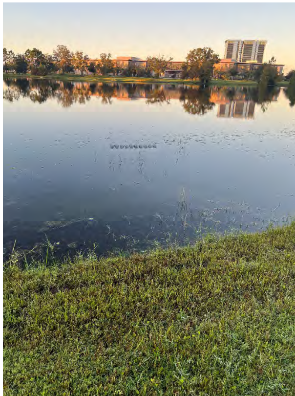
Photo 77 – NW Corner of Pond – Broken Pipe
