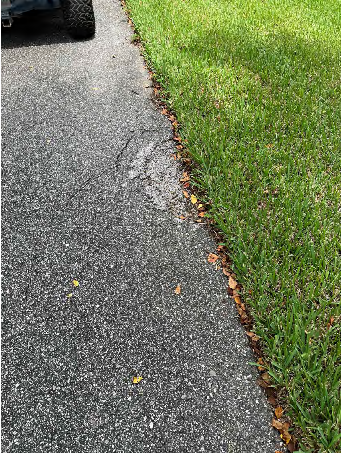
Photo 43 – Raveling Asphalt and Base Failure
