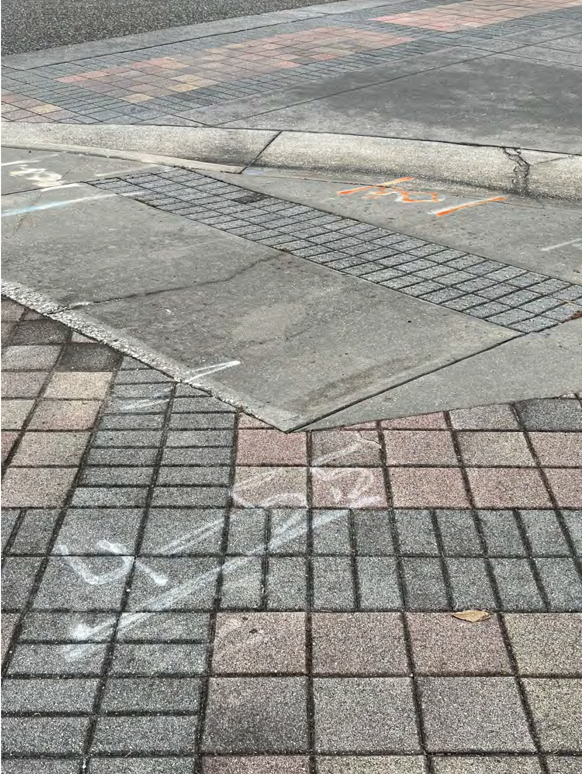
Photo 35 – Surficial Concrete Cracks in Handicap Ramp
