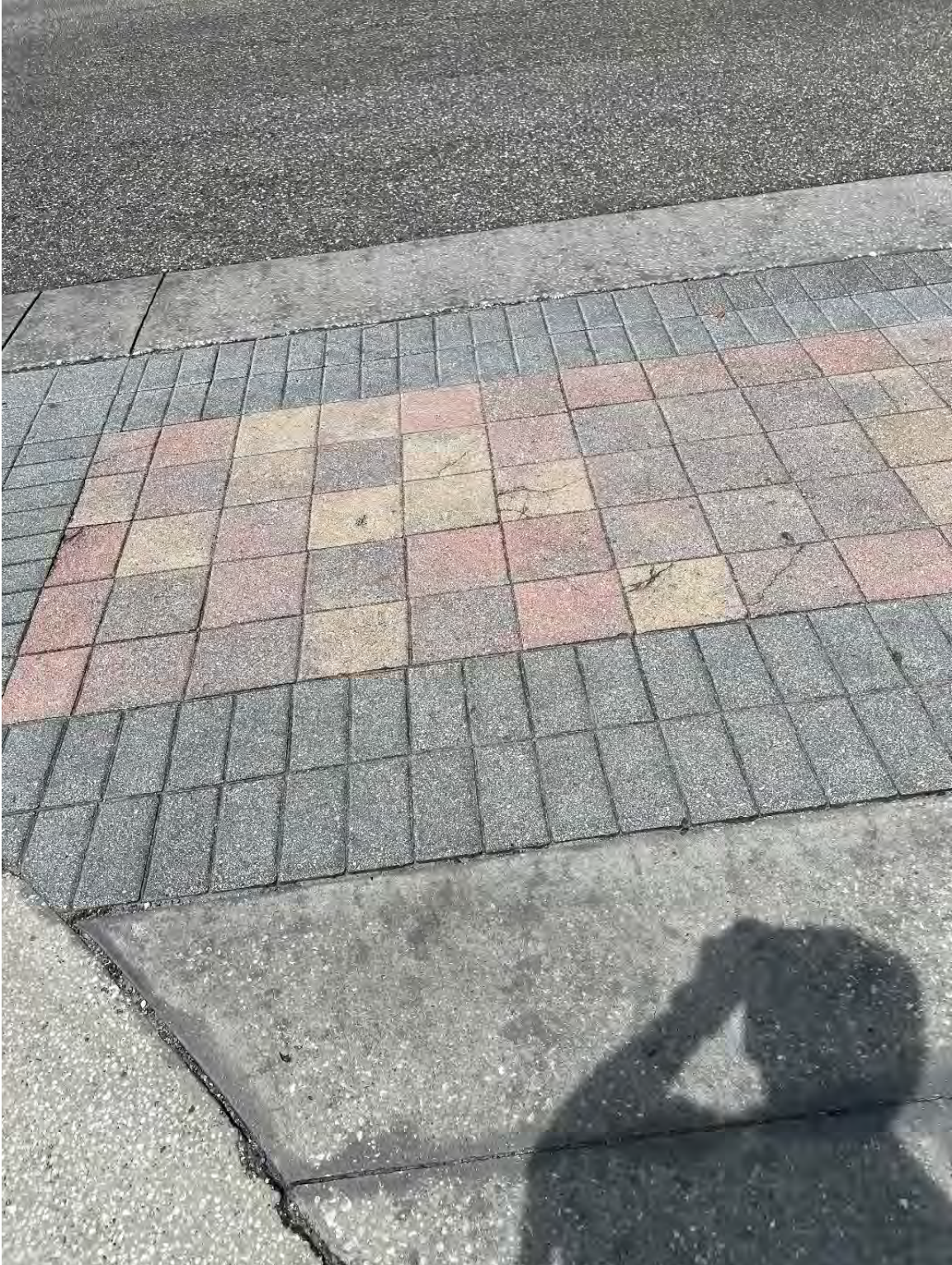
Photo 105 – Cracked Pavers – Some Settling
