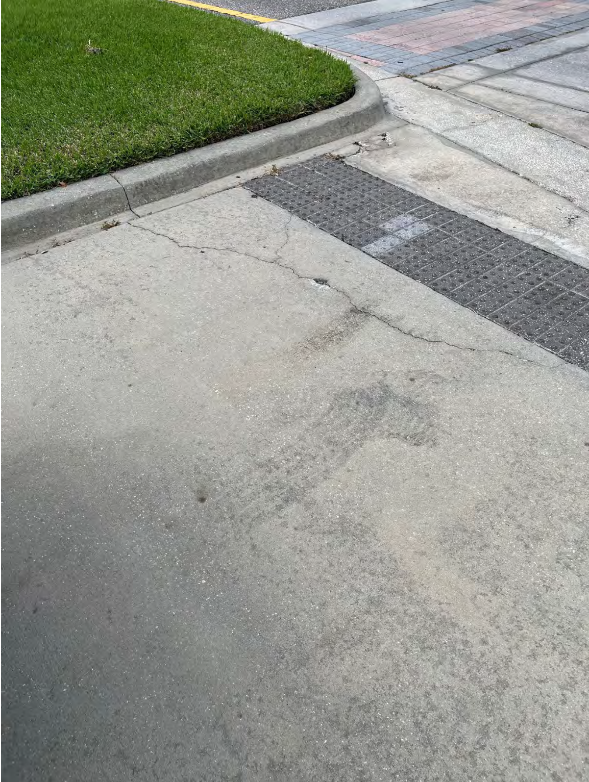
Photo 21 - Surficial Concrete Cracks in Handicap Ramp
