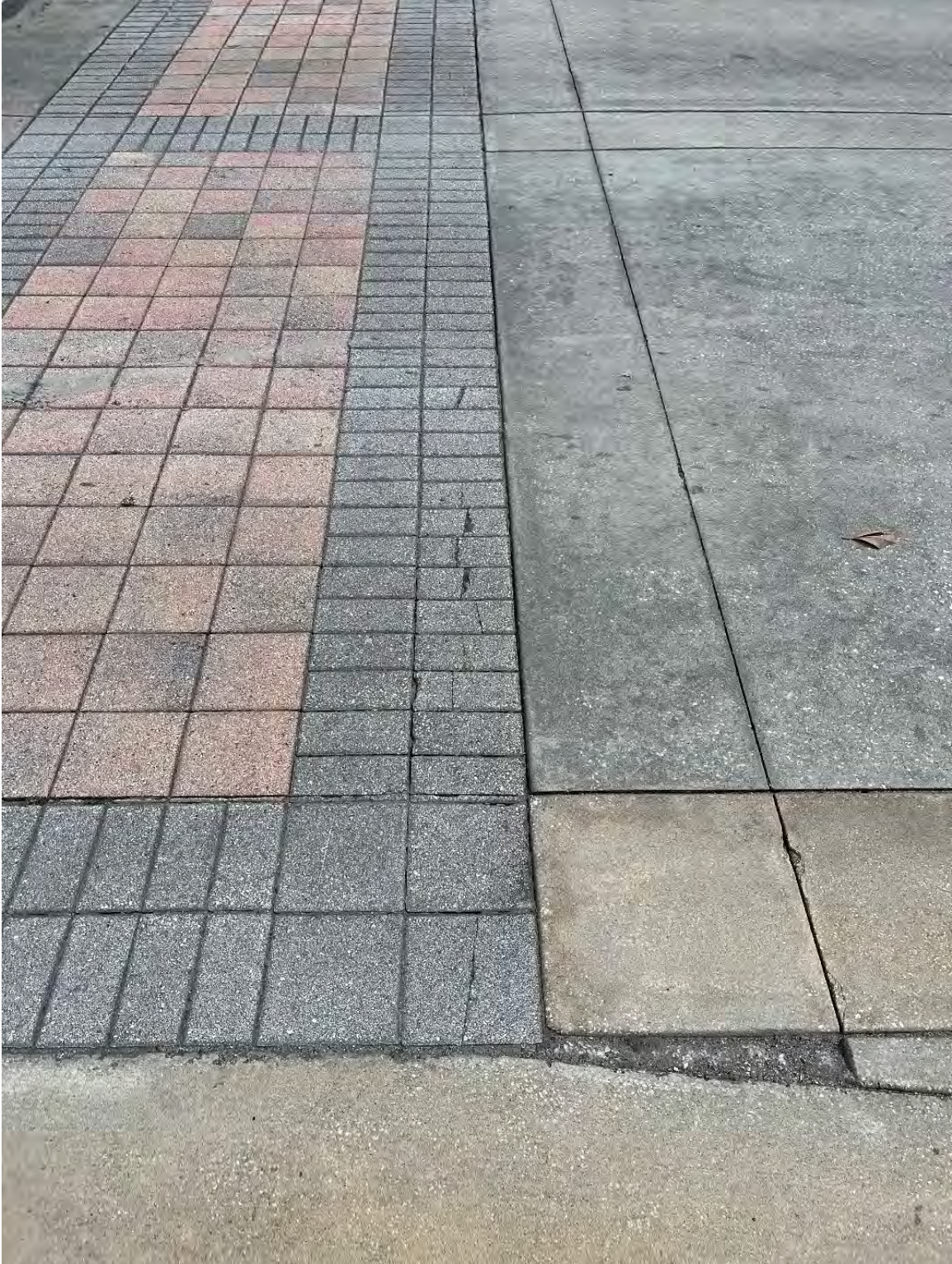
Photo 91 – Cracked Pavers - Minor Settling
