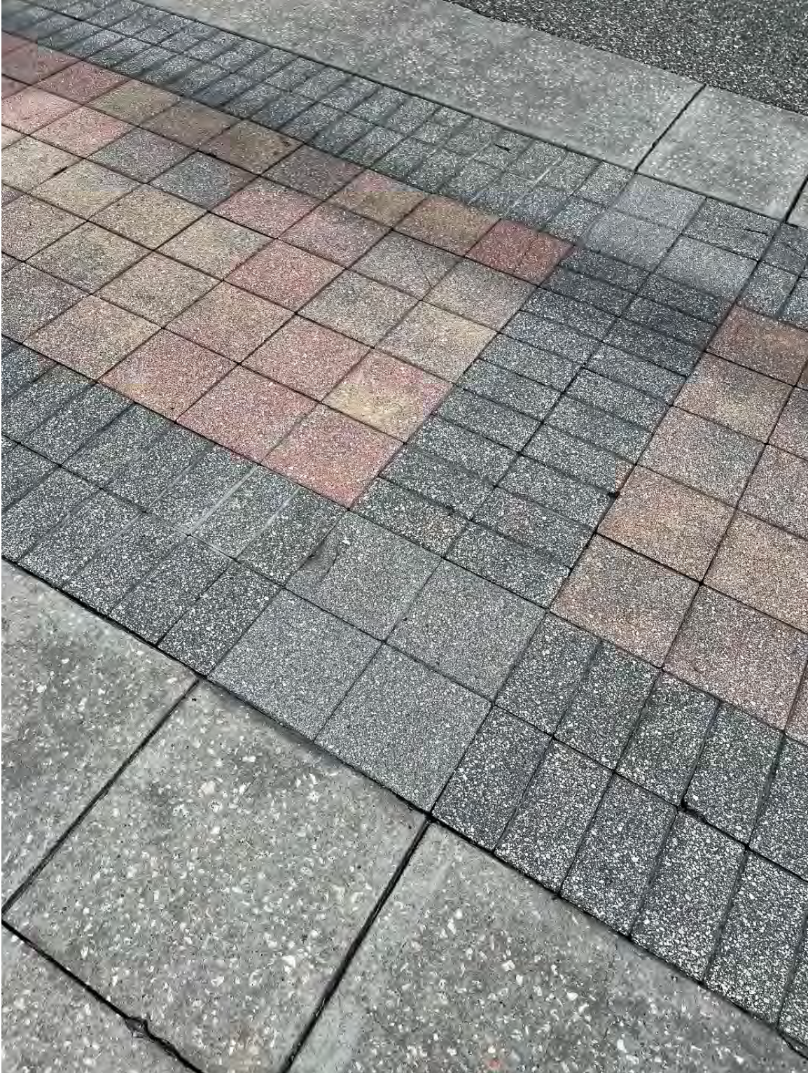
Photo 102– Cracked Pavers – Minor Settling
