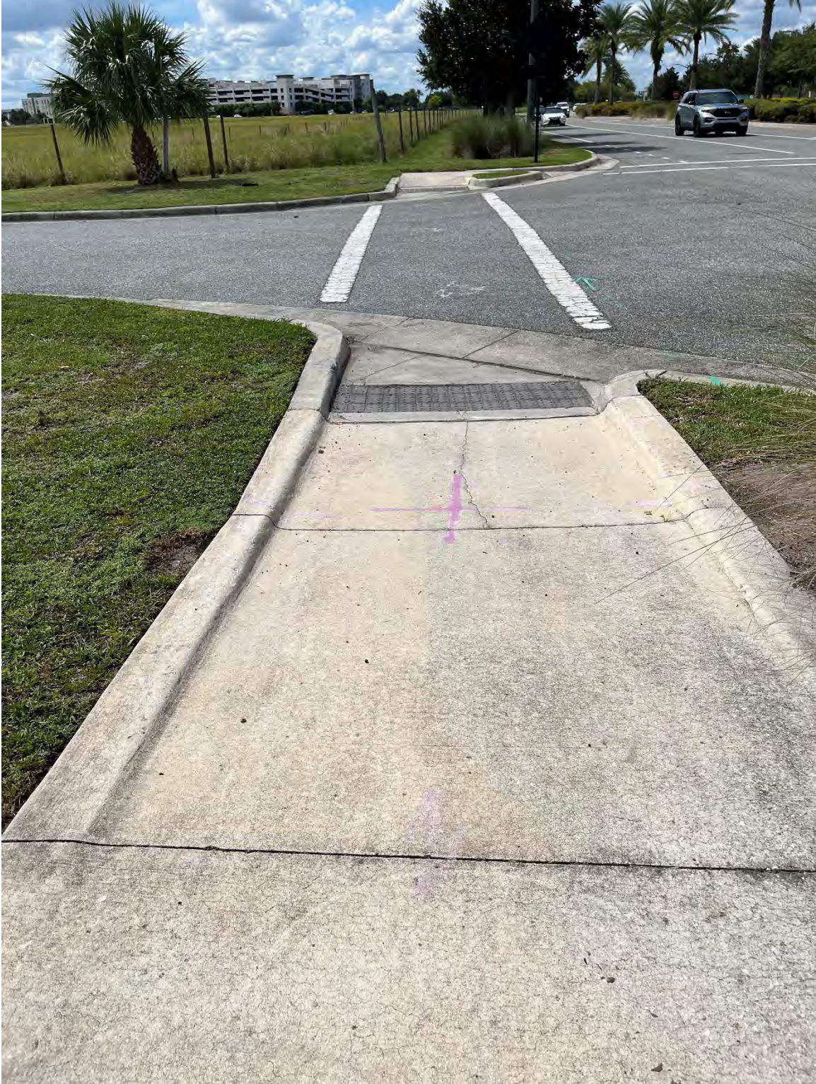
Photo 61 – Surficial Concrete Cracks in Handicap Ramp
