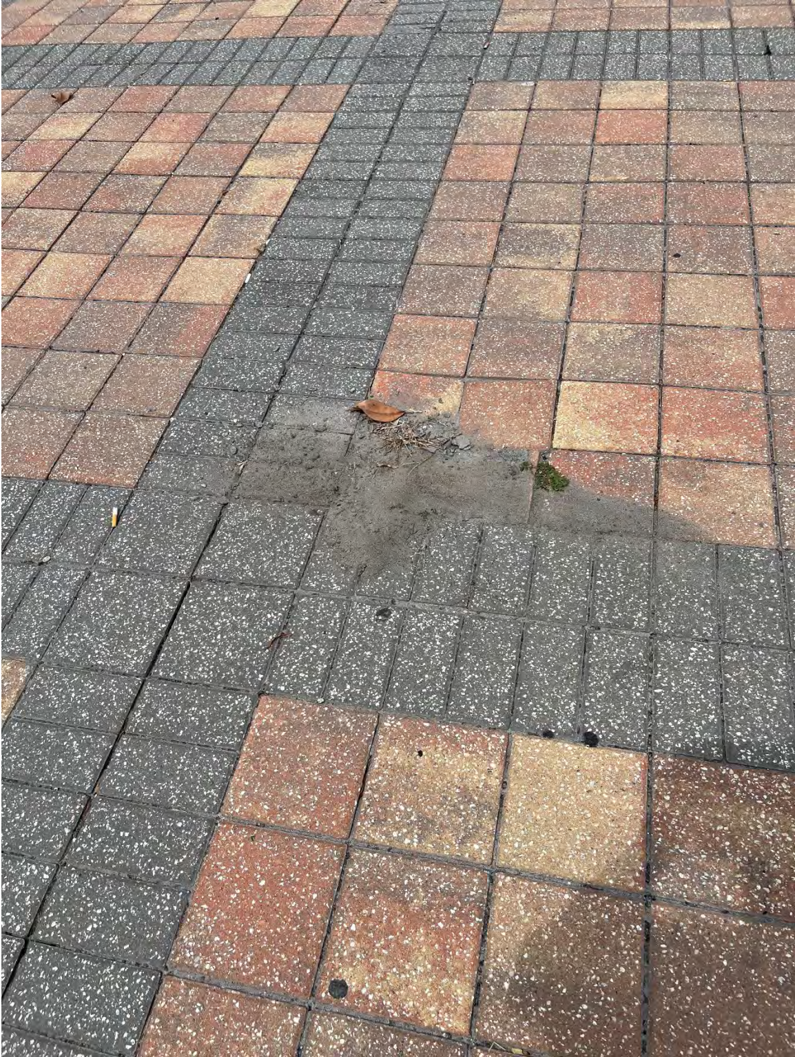
Photo 54 - Paver Base Failure in Median
