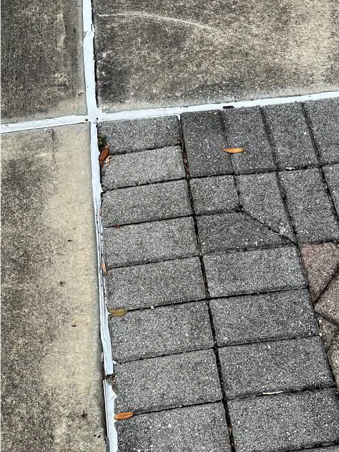
Photo 34 - Paver Base Failure
