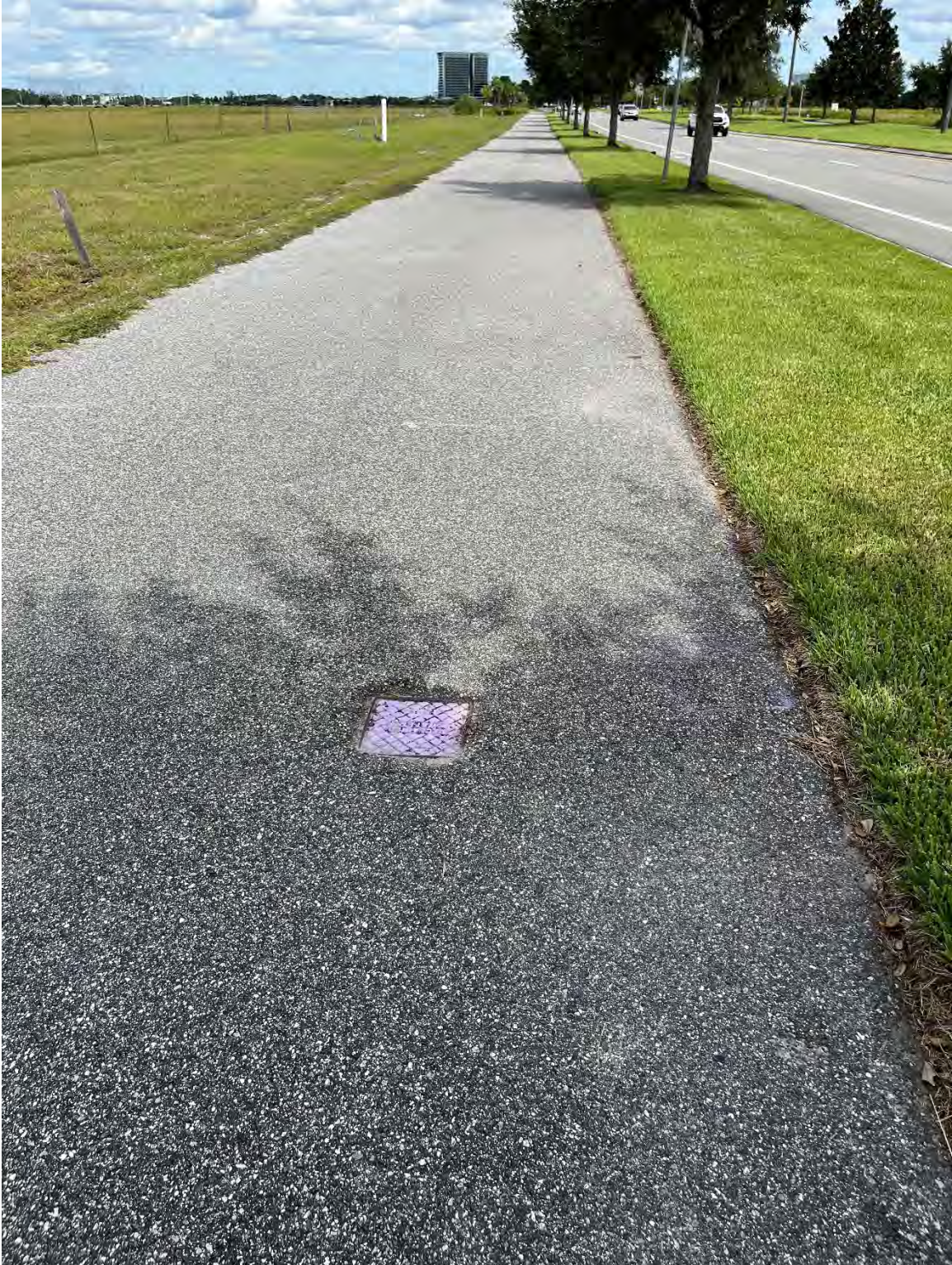
Photo 12 – Sunken Reclaim Water Meter
