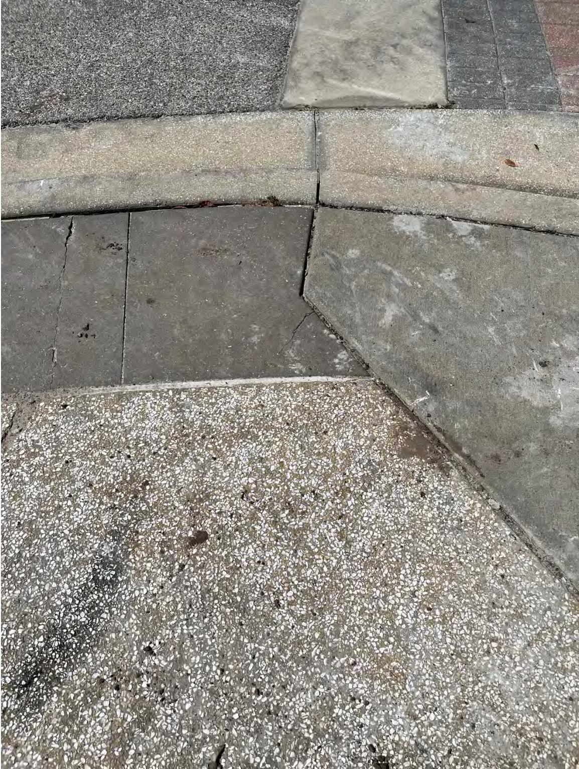
Photo 65 – Concrete Crack in Ribbon Curb (construction ongoing)
