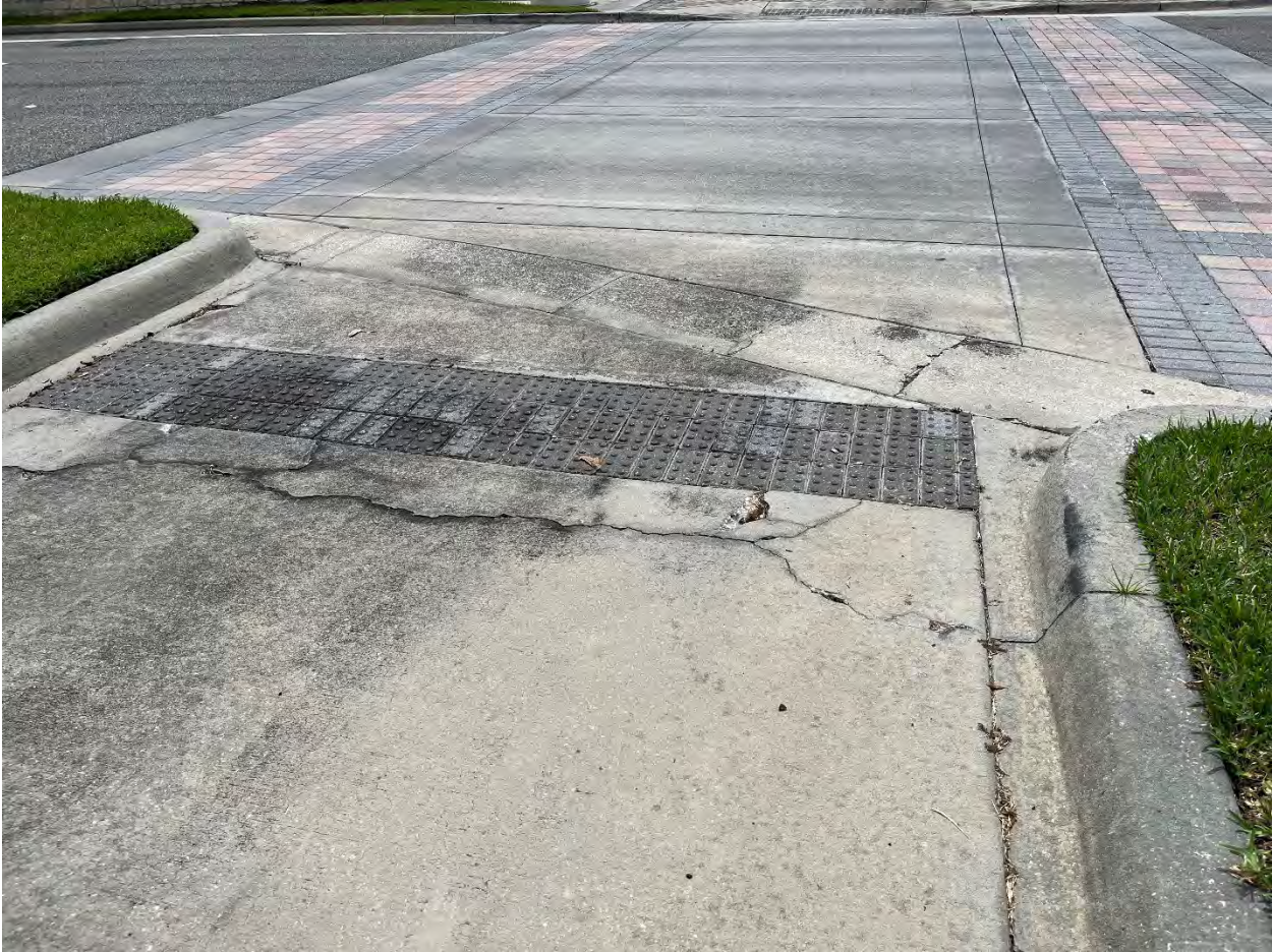
Photo 29 - Surficial Concrete Cracks
