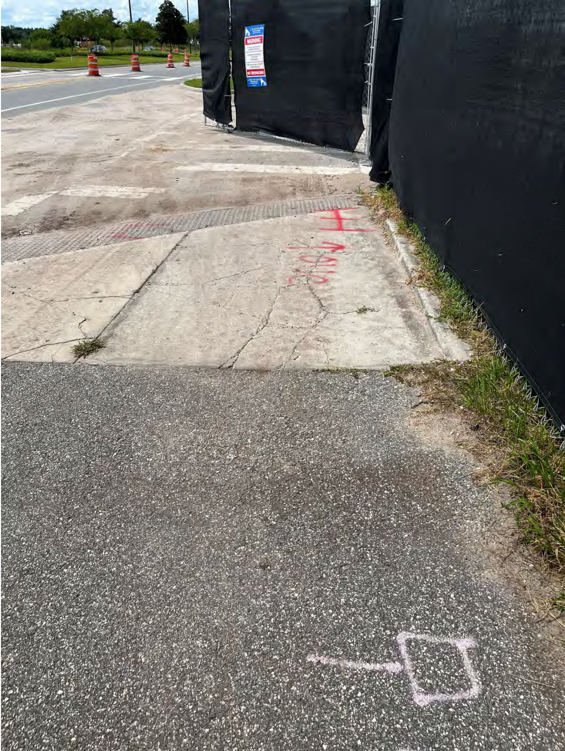
Photo 3 – Surficial Concrete Cracks in Curb Ramp (construction ongoing)
