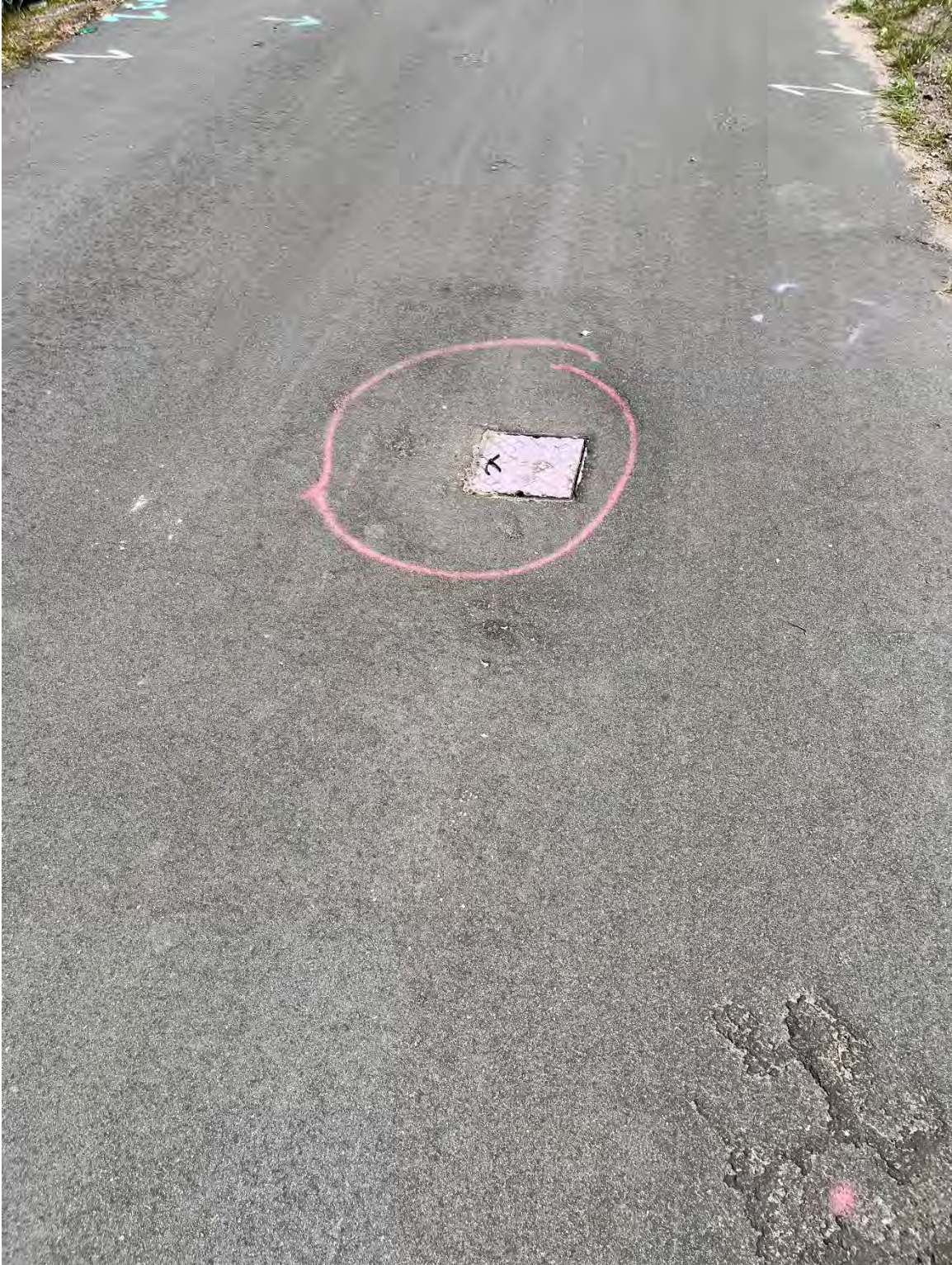
Photo 8 – Sunken Reclaim Water Meter
