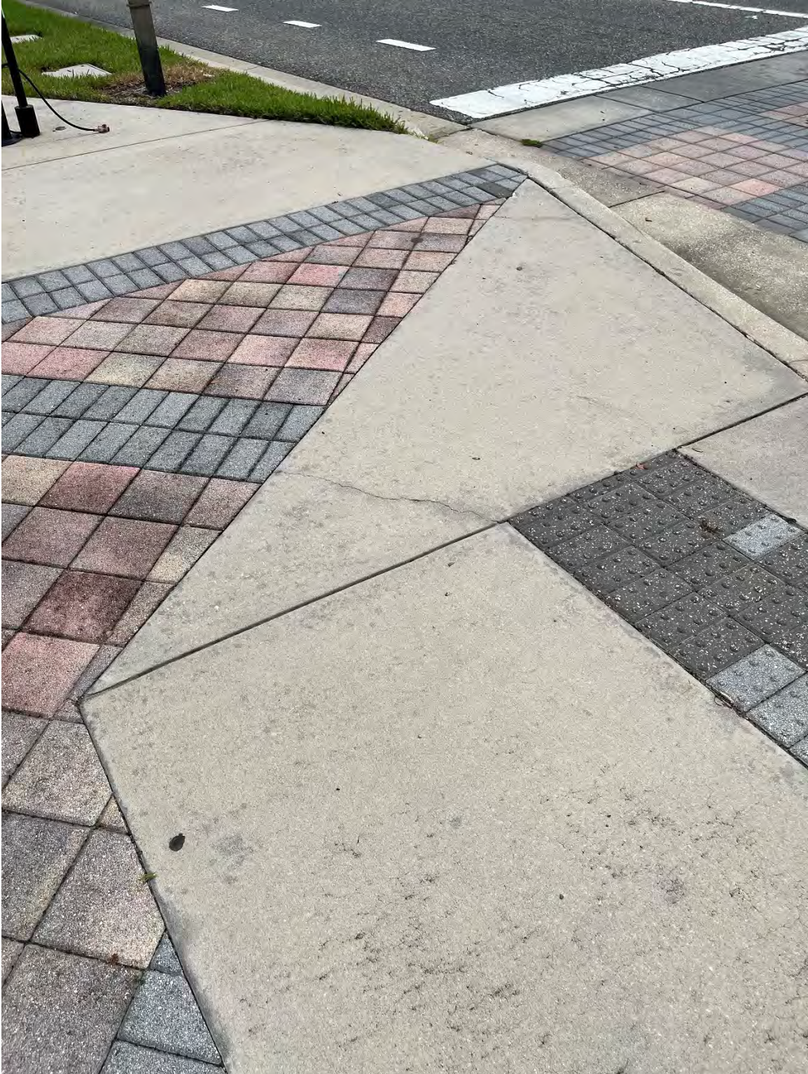
Photo 32 - Surficial Concrete Crack in Handicap Ramp
