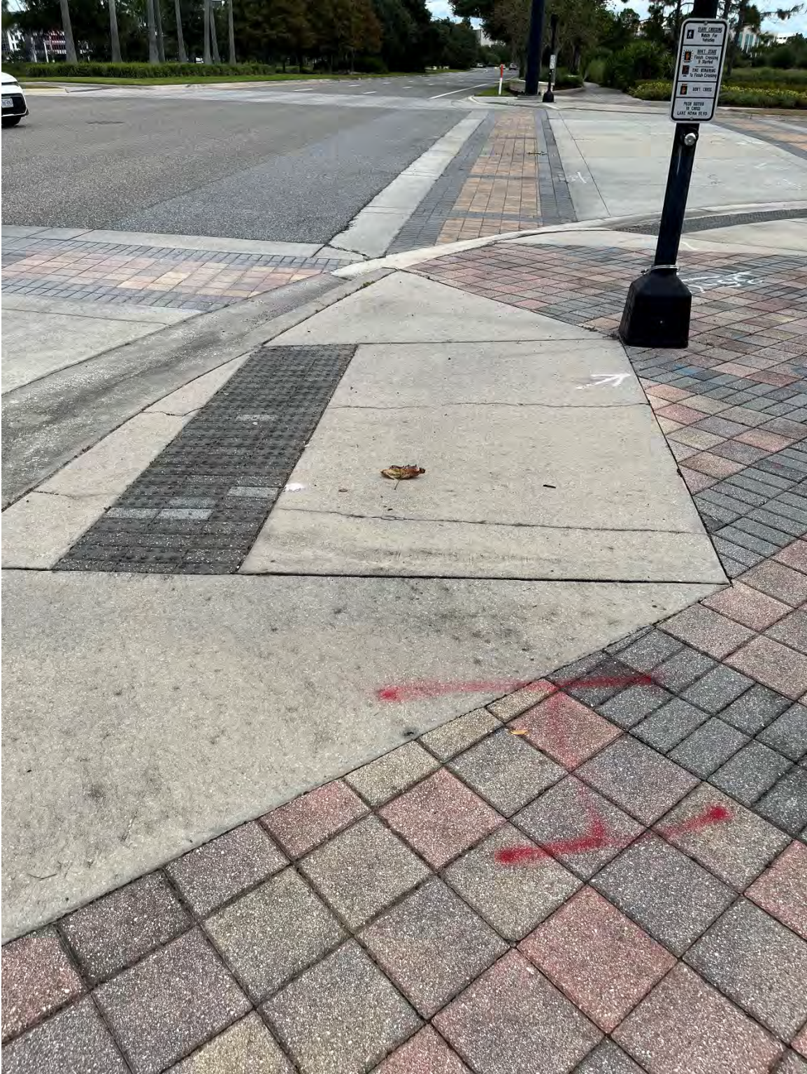
Photo 18 – Surficial Concrete Cracks in Handicap Ramp
