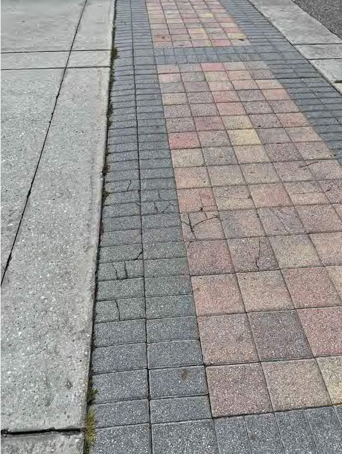
Photo 100 – Cracked Pavers - Sinking Pavers (Approximately ½")
