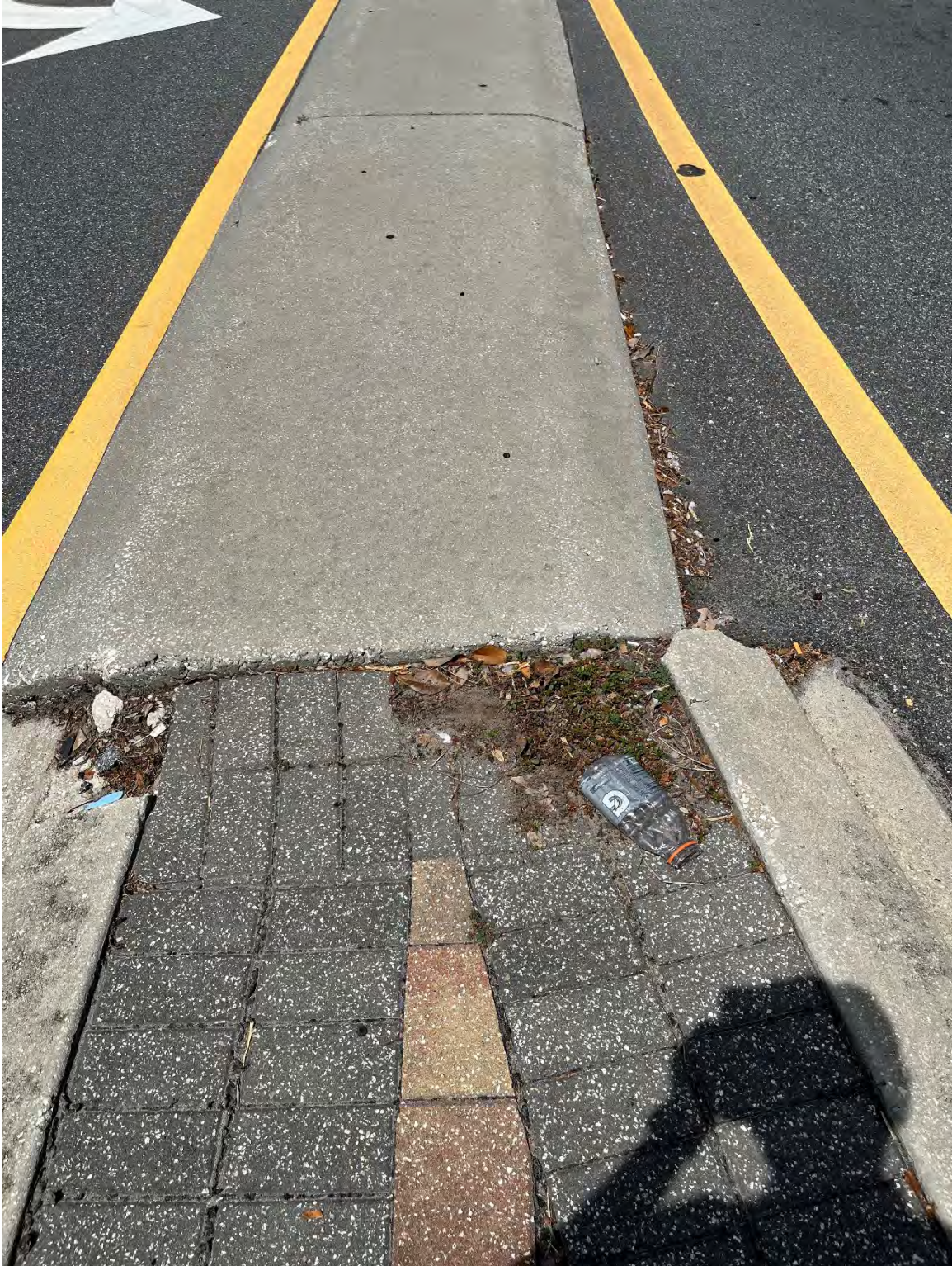
Photo 57 - Paver Base Failure in North Median Looking North
