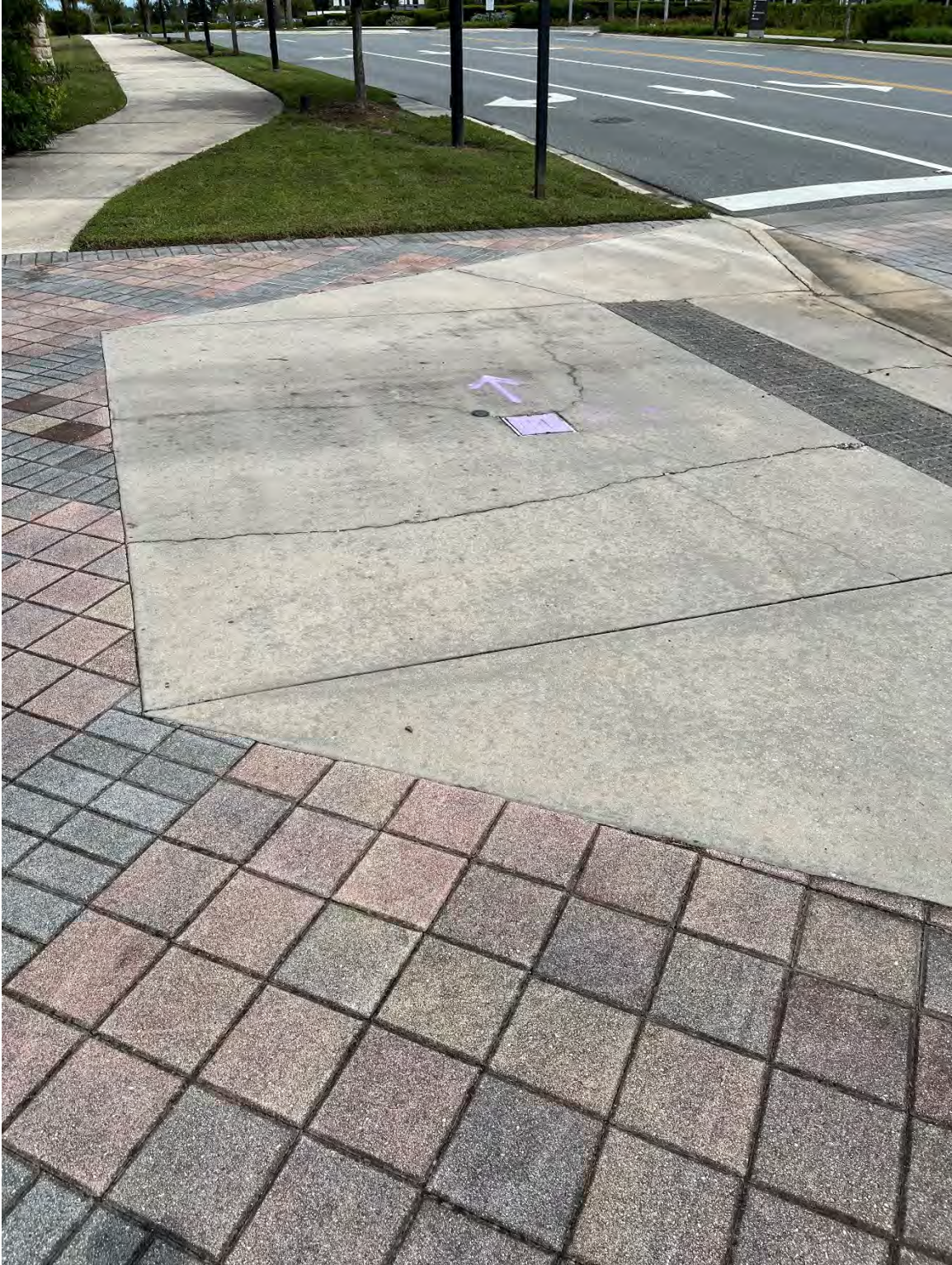
Photo 22 – Surficial Concrete Cracks in Handicap Ramp
