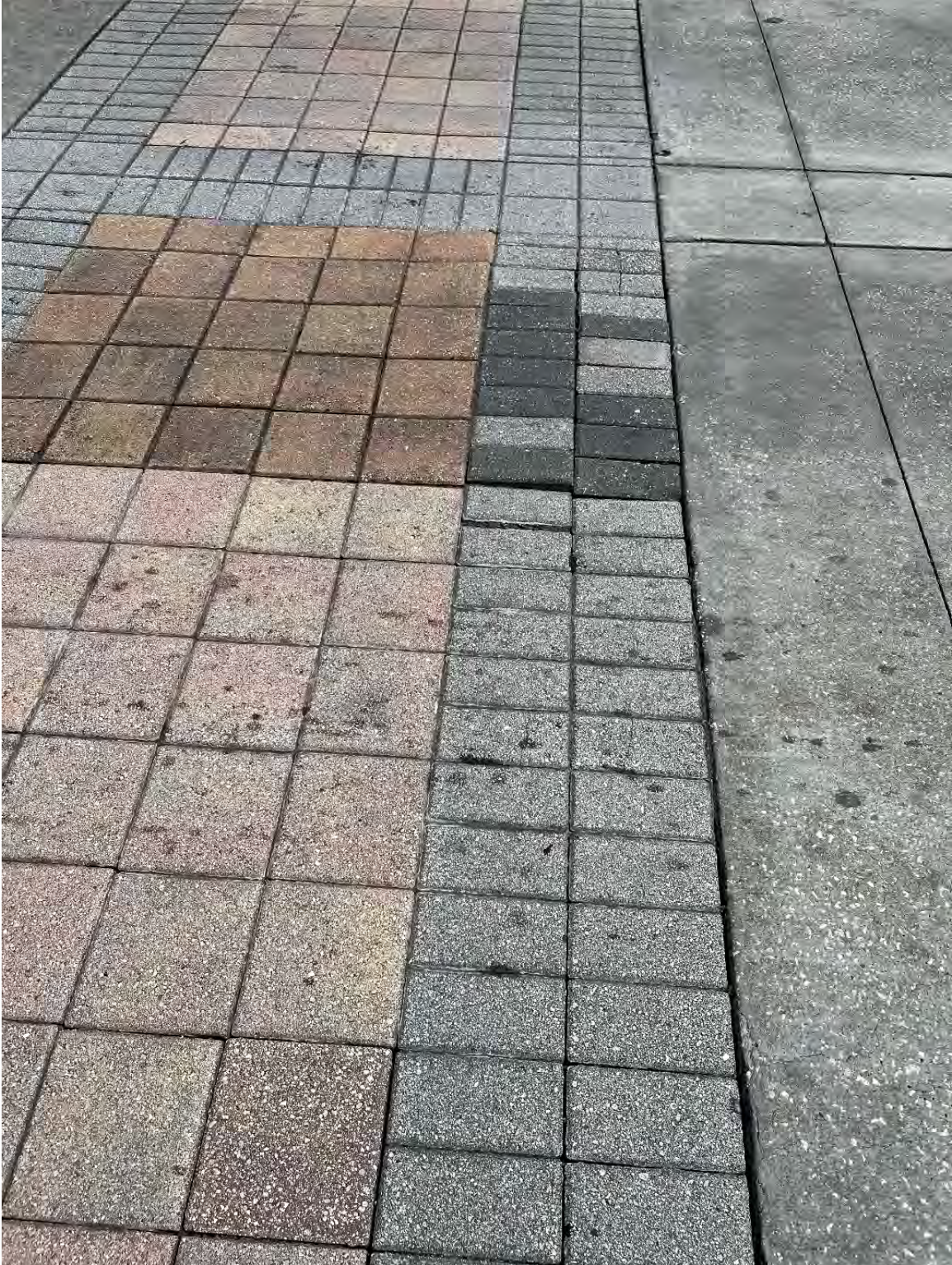
Photo 92 – Surficial Paver Cracks- Minor Settling
