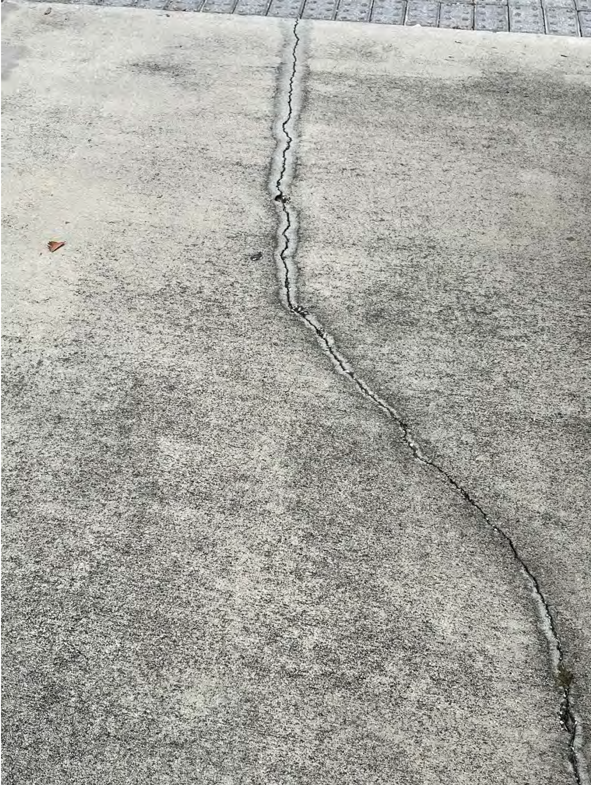
Photo 39 – Surficial Concrete Cracks in Median Strip
