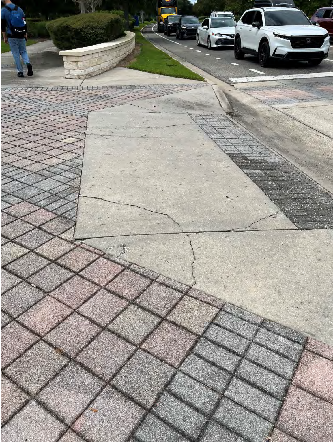
Photo 33 – Surficial Concrete Cracks in Handicap Ramp
