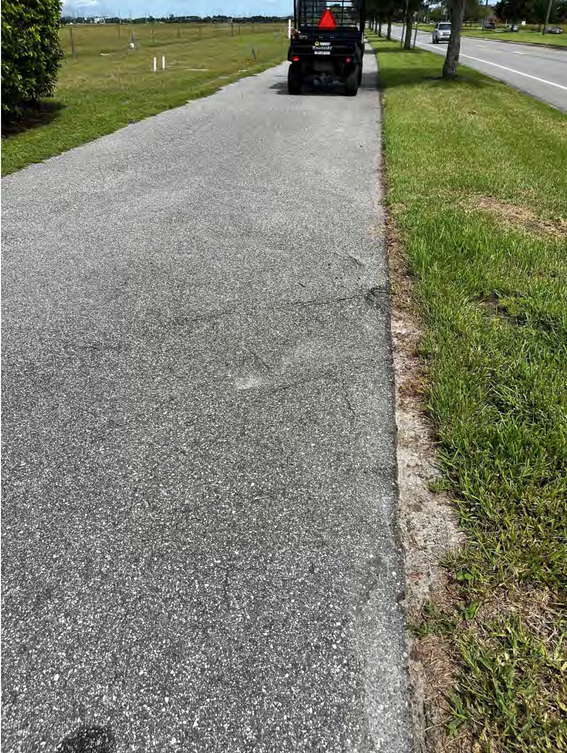
Photo 11 – Raveling Asphalt with Depression and Base Failure
