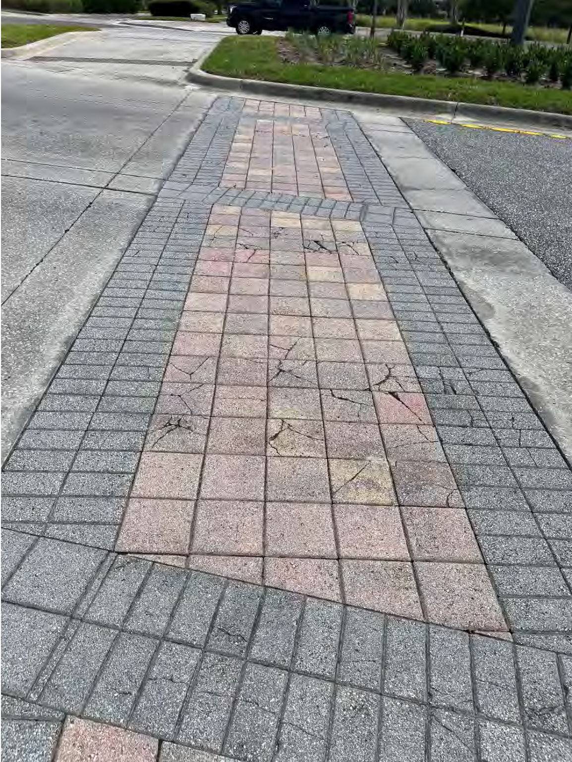
Photo 113 – Multiple Cracked Concrete – Pavers Settling – Broken Flush Curb
