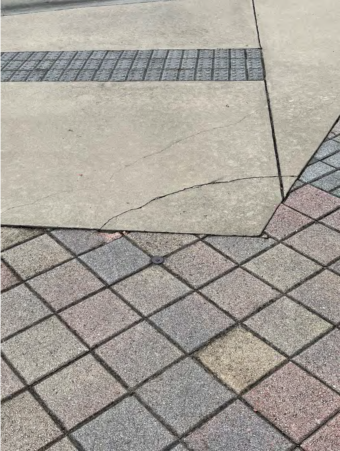
Photo 40 - Surficial Concrete Cracks in Handicap Ramp
