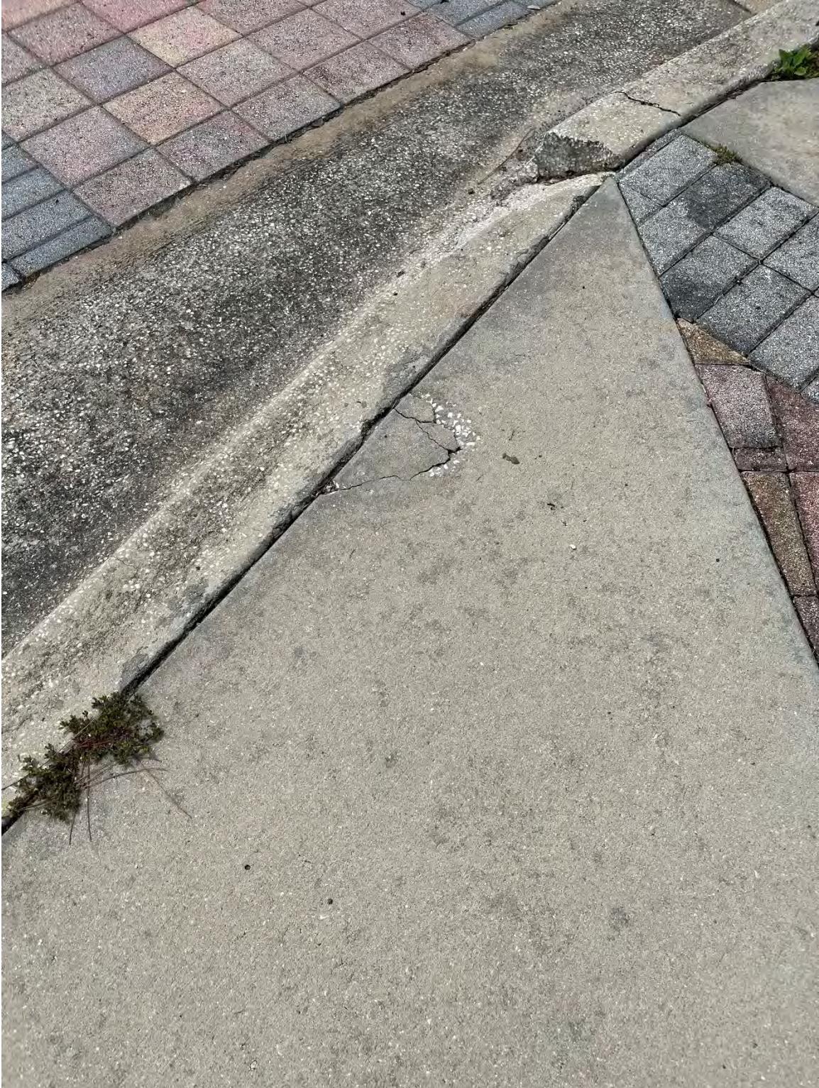
Photo 23 - Cracked Concrete in Handicap Ramp
