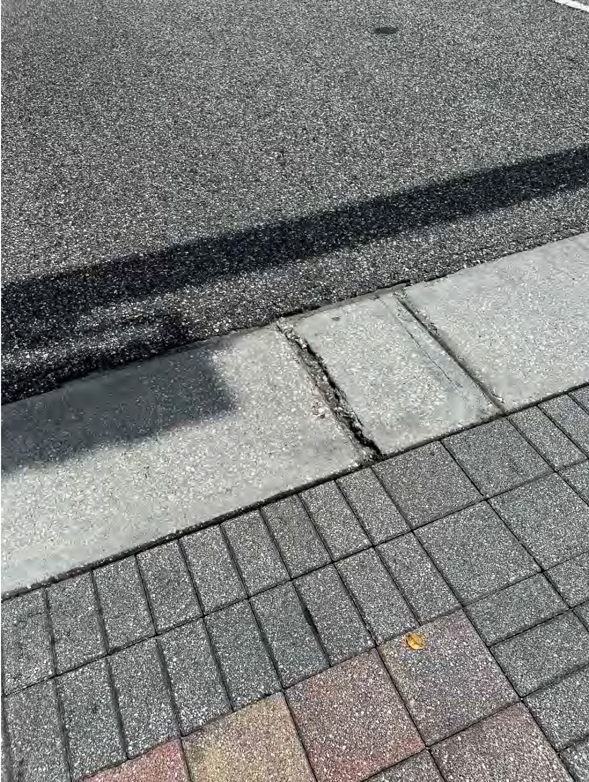
Photo 94 – Cracked Concrete - Minor Settling
