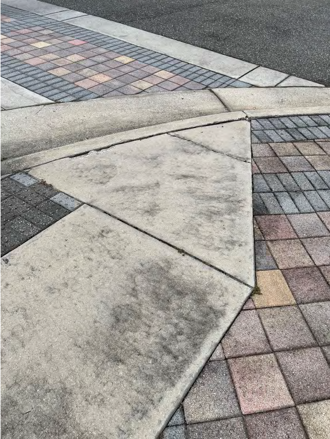
Photo 31 – Surficial Concrete Crack in Handicap Ramp
