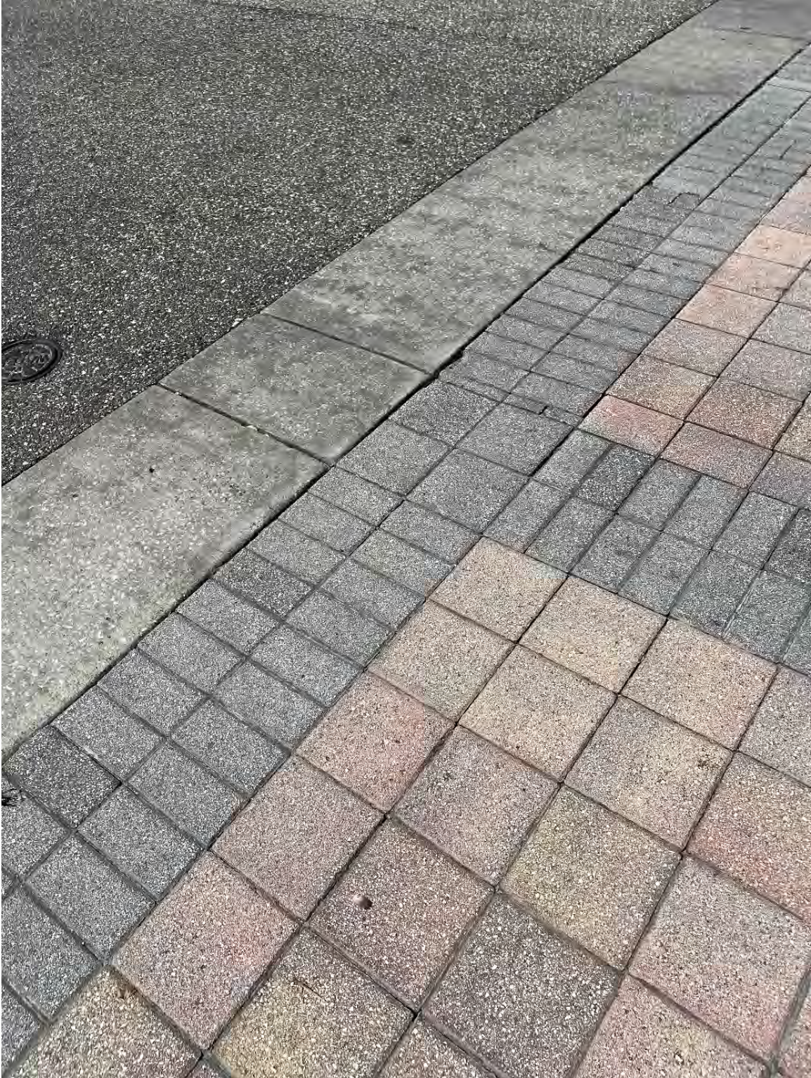
Photo 106 – Cracked Pavers – Settling Pavers
