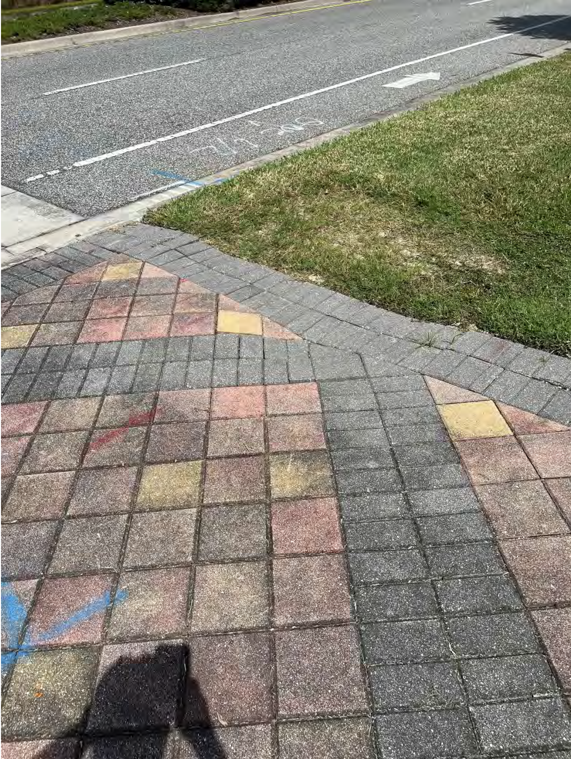
Photo 60 - Paver Base Failure
