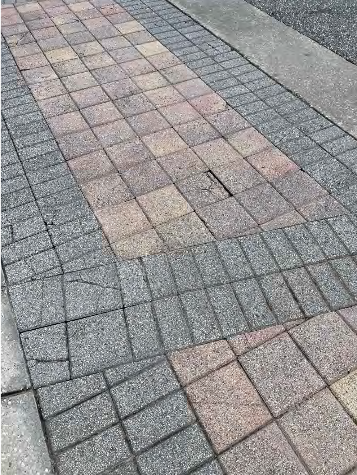
Photo 112 – Cracked Concrete – Pavers Settling
