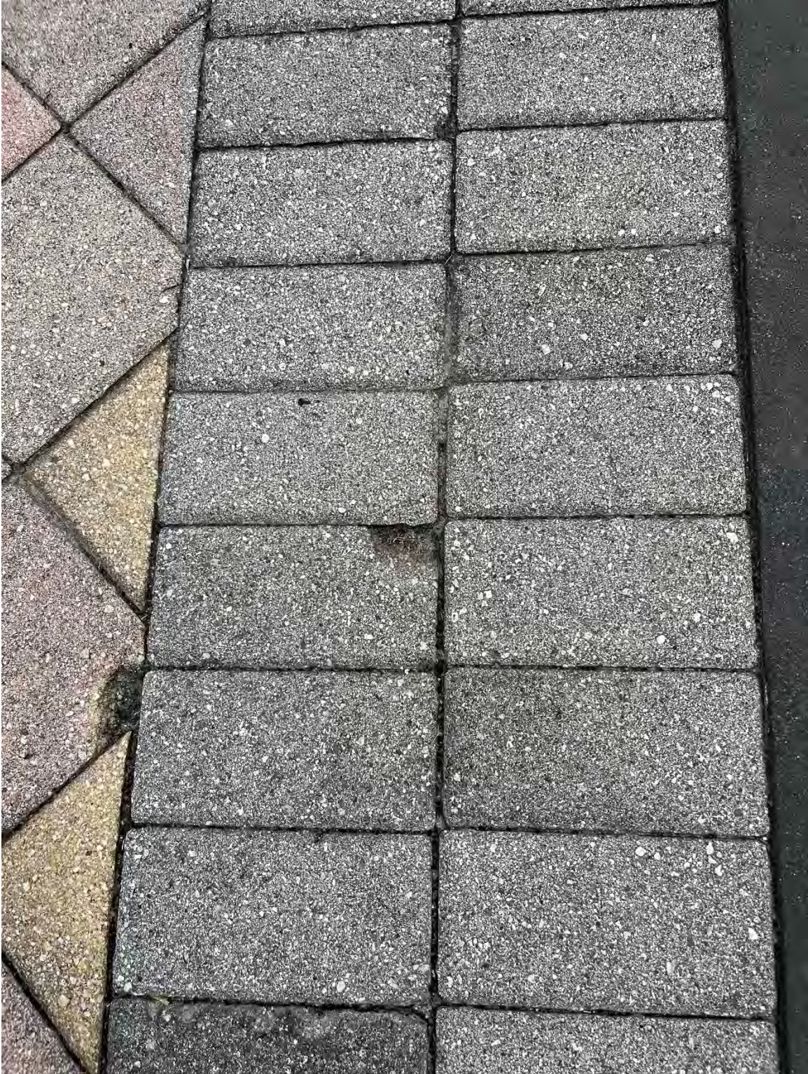
Photo 45 - Multiple Chipped Pavers
