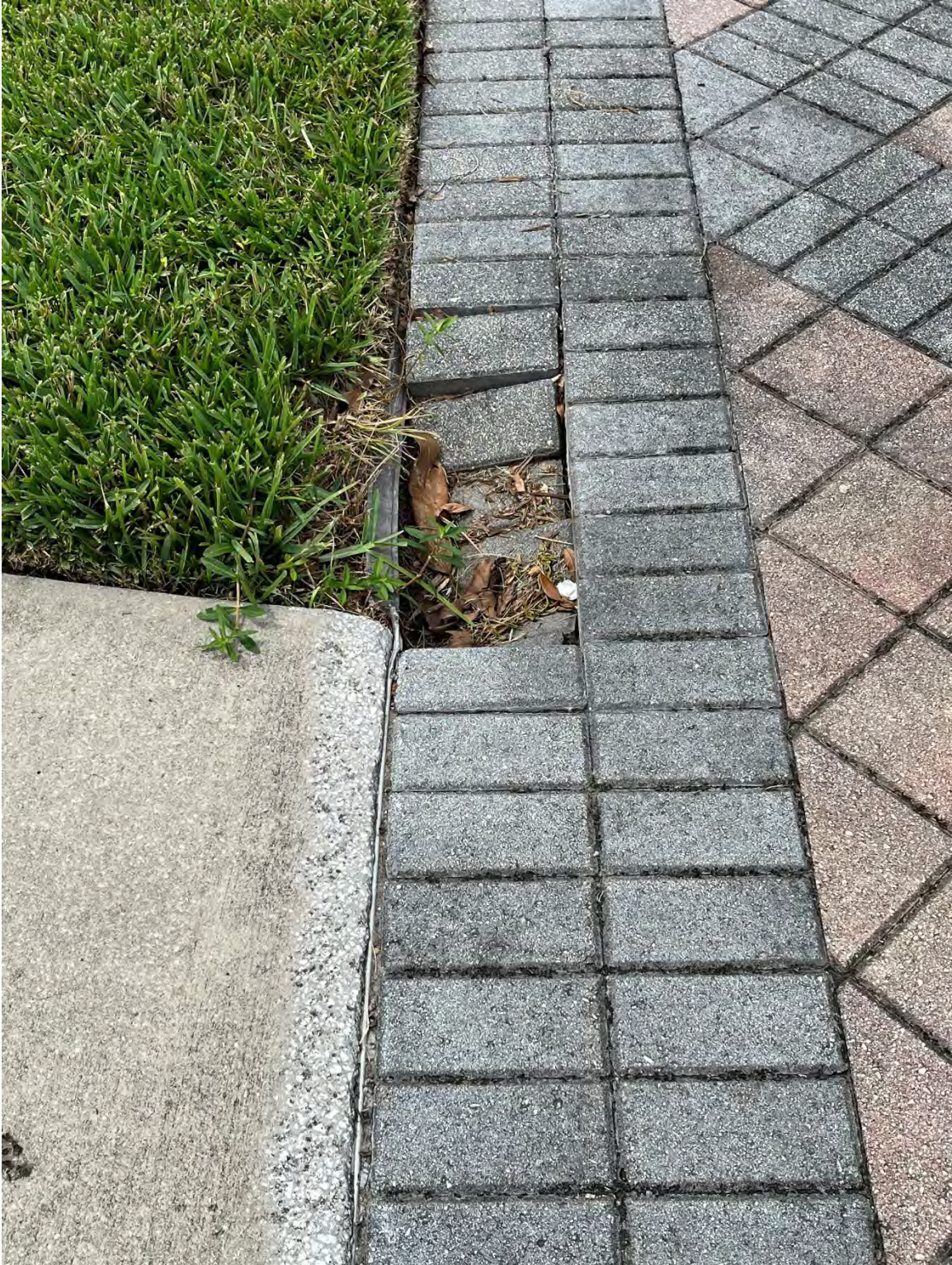
Photo 27 - Paver Base Failure
