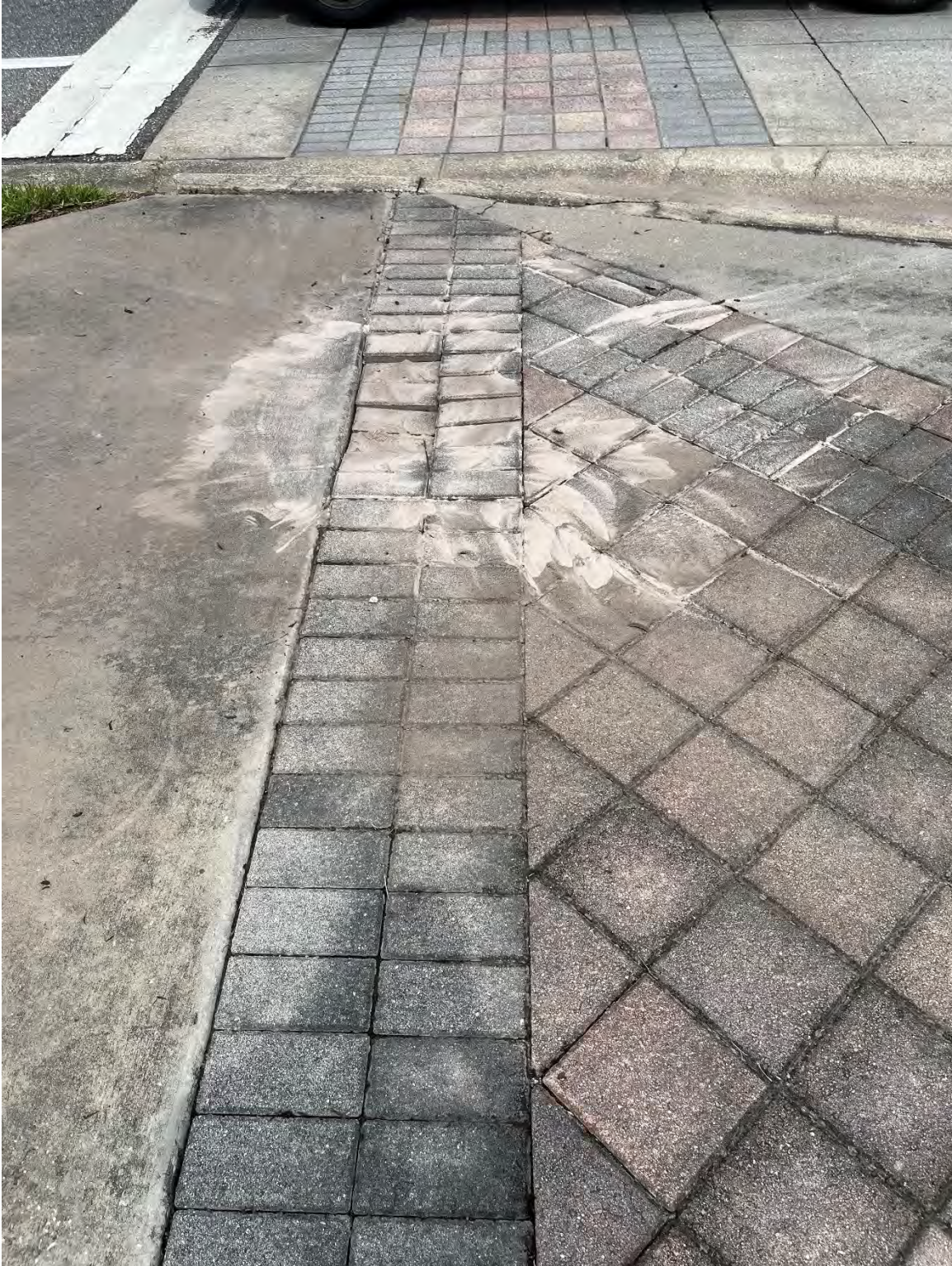
Photo 25 - Paver Base Failure
