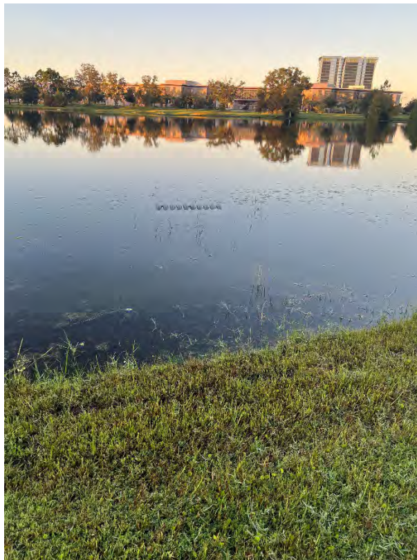
Photo 77 – NW Corner of Pond – Broken Pipe
