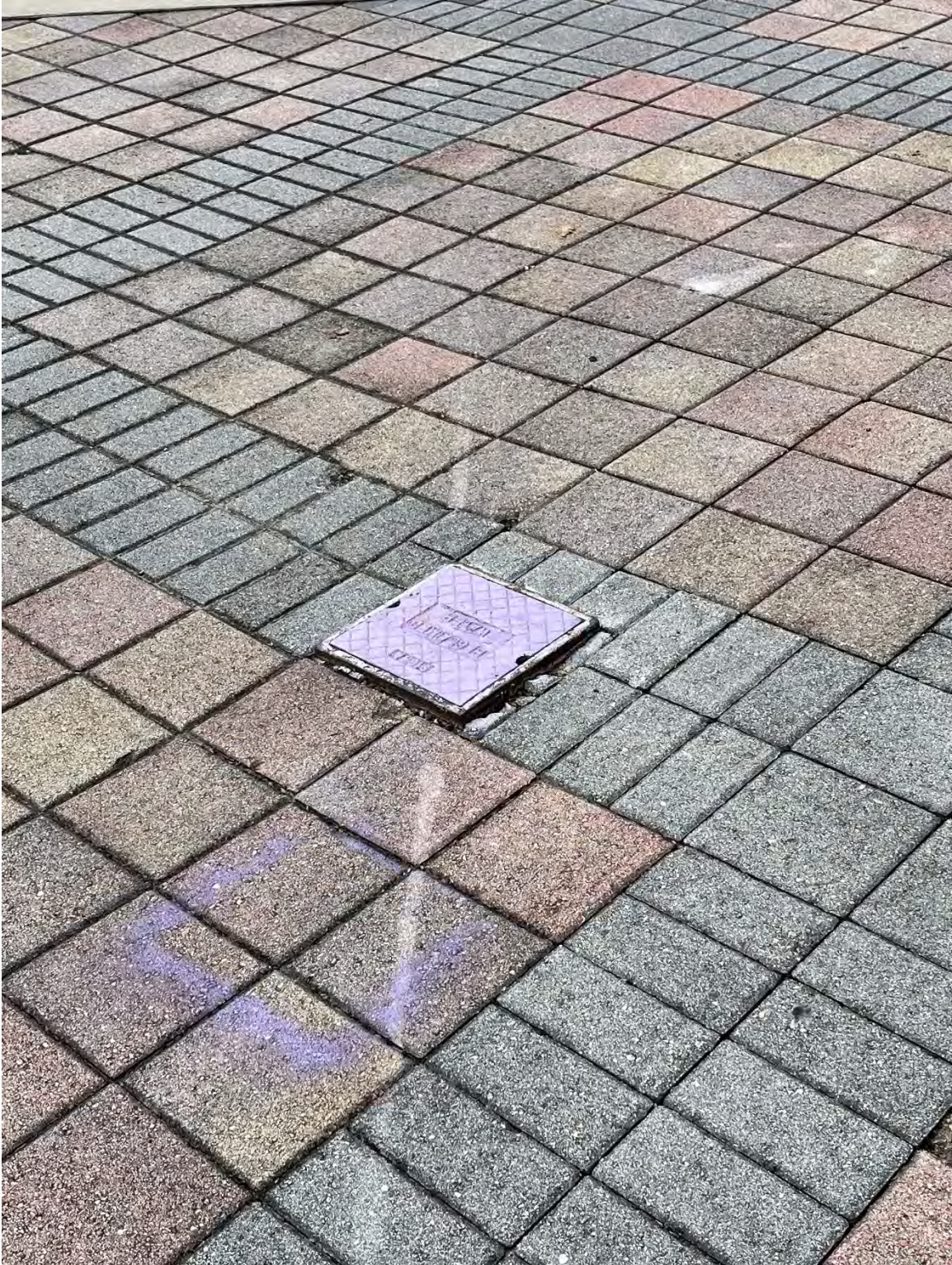
Photo 42 - Raised Reclaim Meter (Approximately 1/2 inch)
