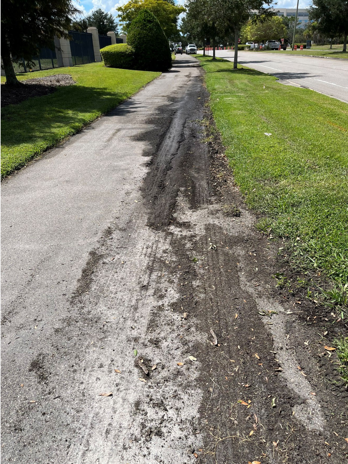
Photo 64 - Poor Drainage Area
