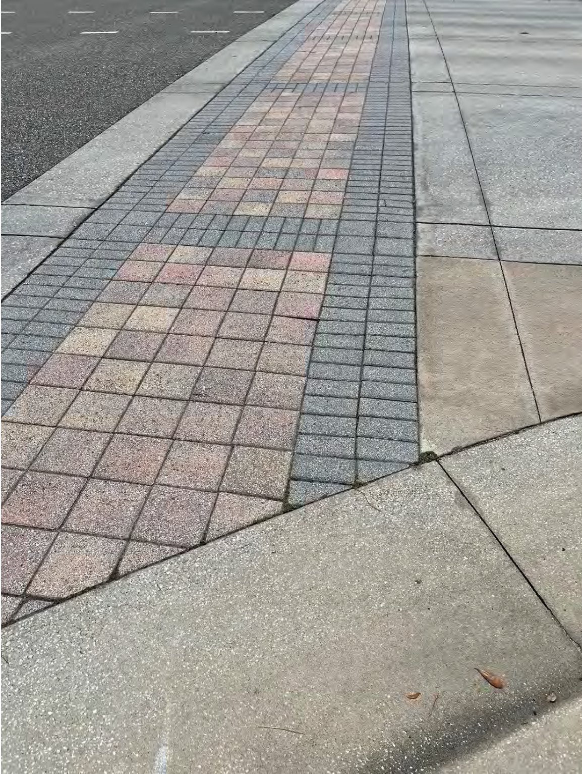
Photo 99 – Cracked Pavers – Paver Settling
