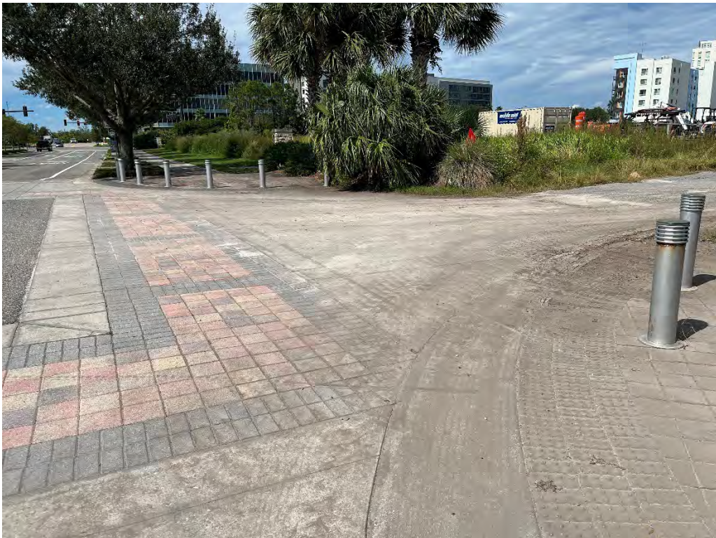
Photo 118 – Construction Entrance – Broken Concrete in Flush Curb
