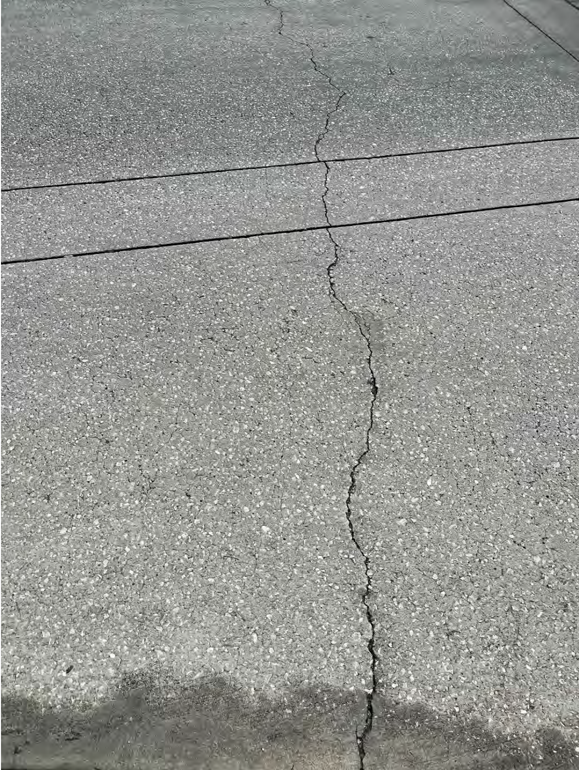
Photo 125 – Surficial Concrete Cracks
