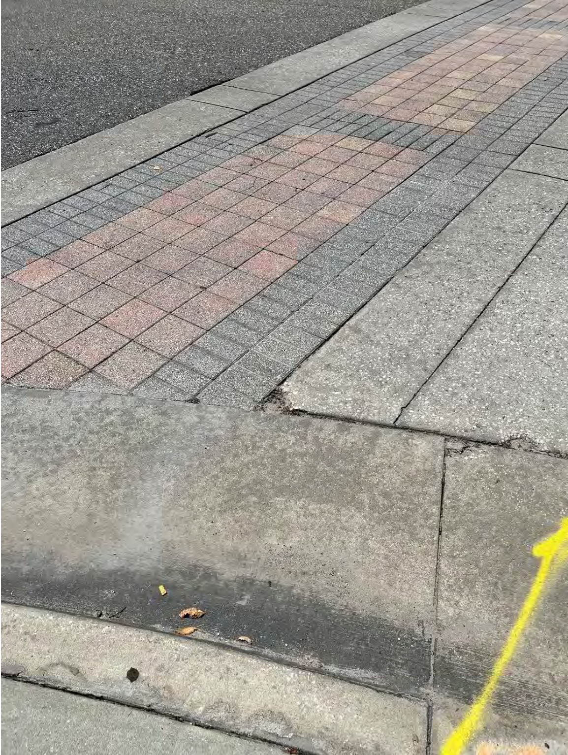
Photo 98 – Cracked Pavers – Broken Concrete
