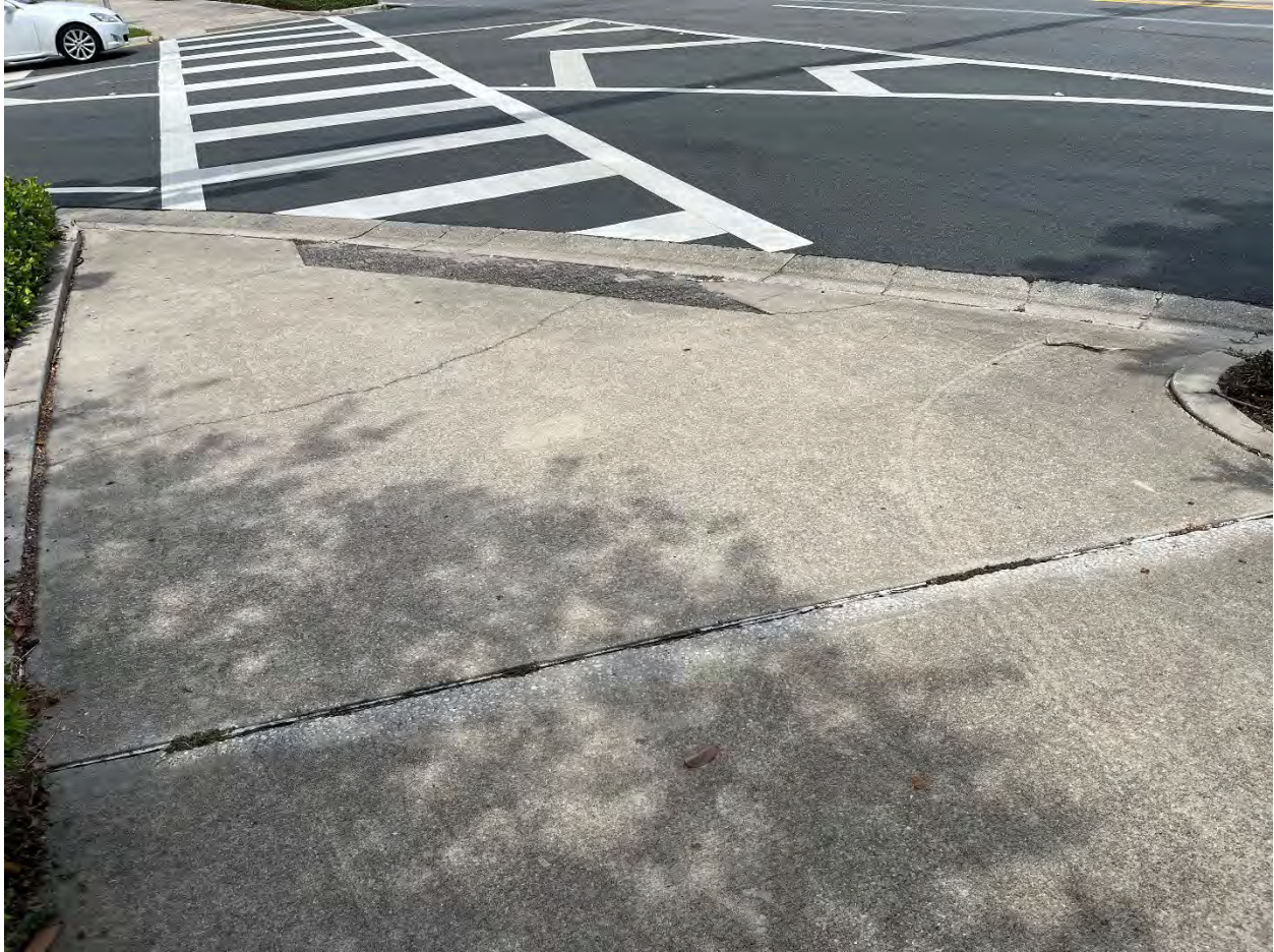
Photo 55 – Surficial Concrete Cracks in Handicap Ramp in Median
