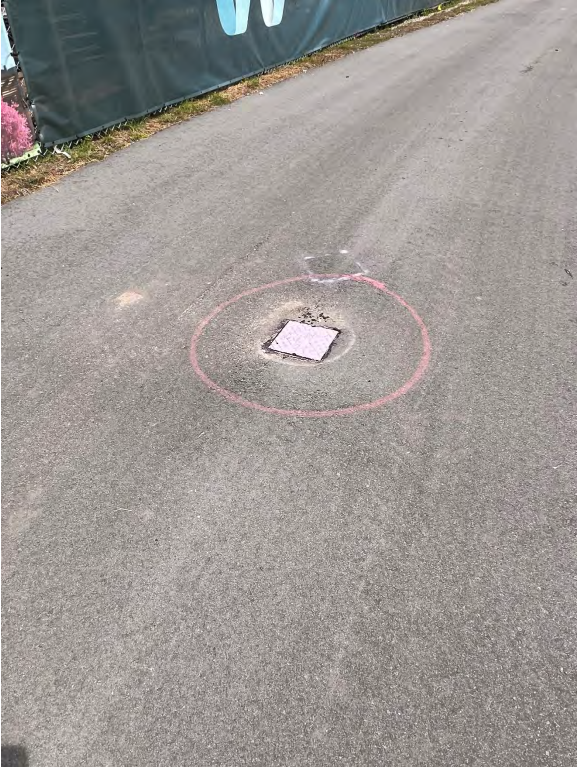
Photo 6 – Sunken Reclaim Water Meter
