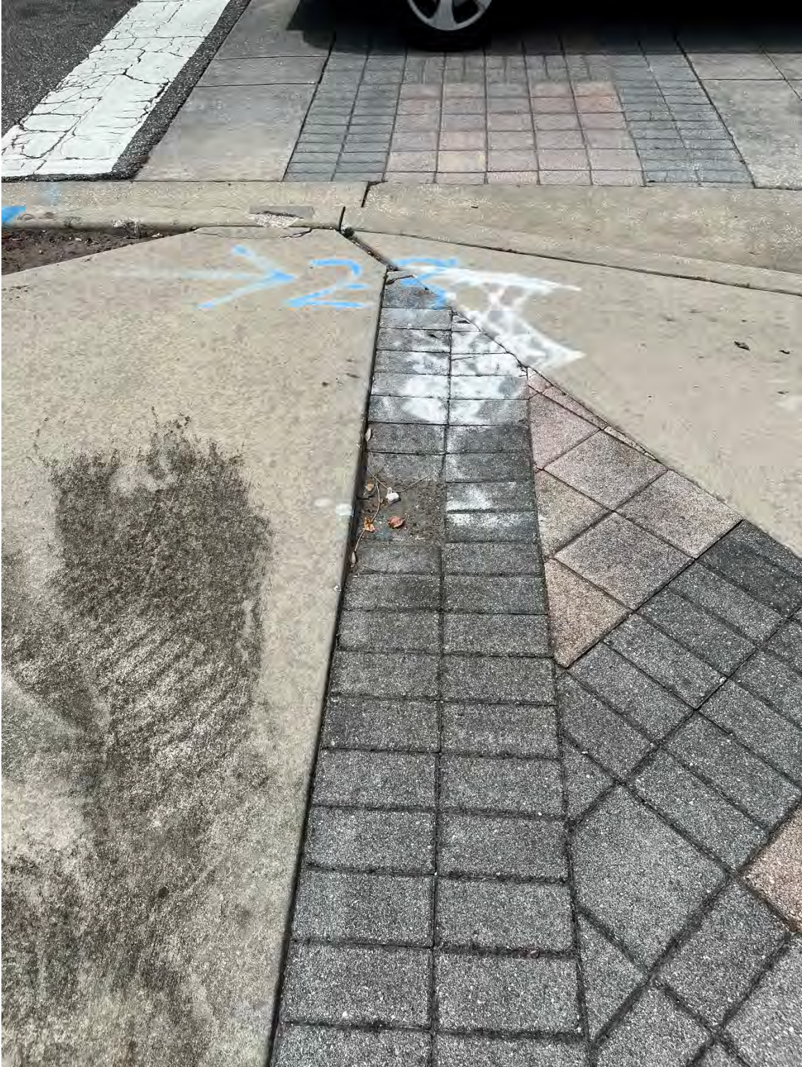
Photo 50 - Cracks in Handicap Ramp, Paver Base Failure
