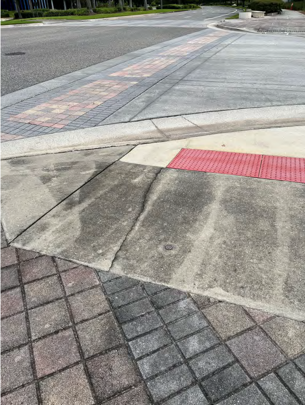
Photo 26 – Surficial Concrete Cracks in Handicap Ramp
