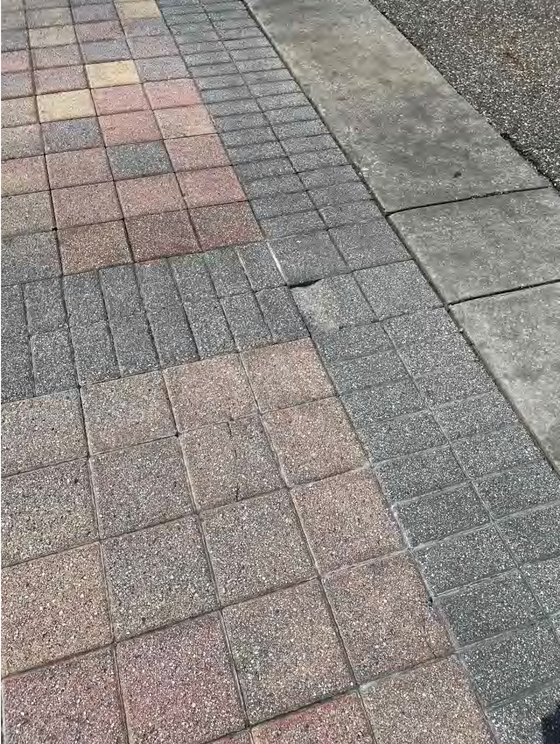
Photo 95 – Cracked Pavers - Minor Settling
