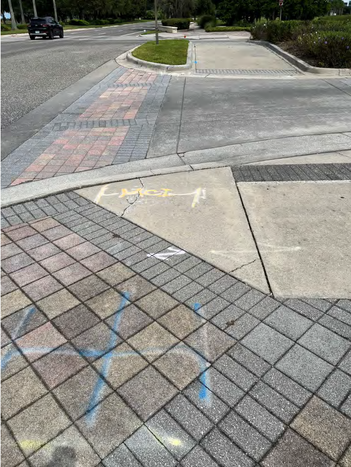
Photo 16 – Surficial Concrete Cracks in Handicap Ramp
