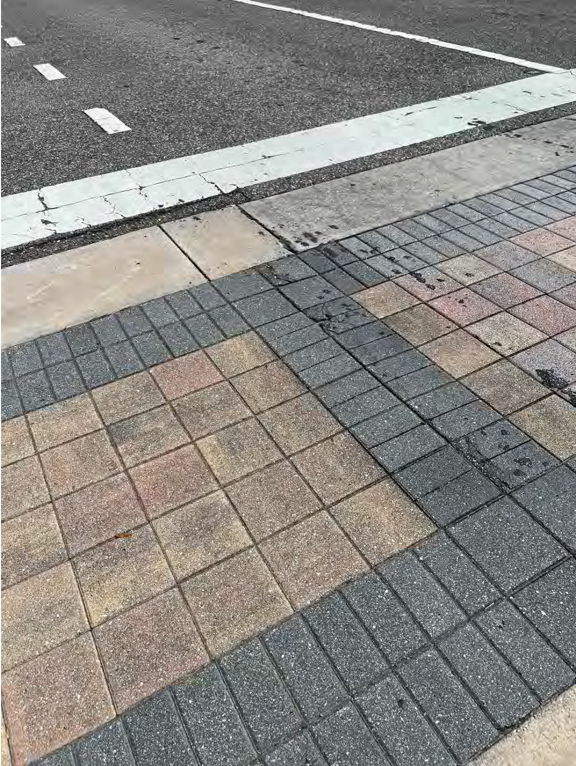
Photo 111 – Broken Concrete Flush Curb
