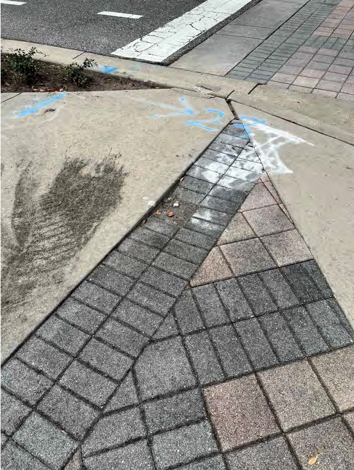
Photo 52 – Surficial Concrete Cracks in Handicap Ramp, Paver Base Failure
