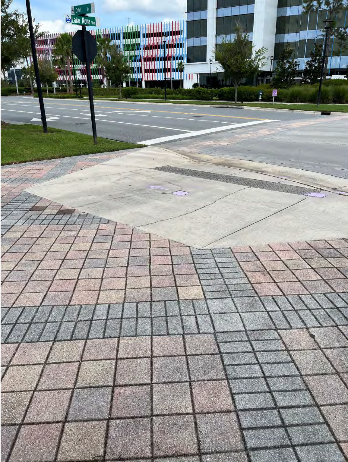
Photo 20 – Surficial Concrete Cracks in Handicap Ramp
