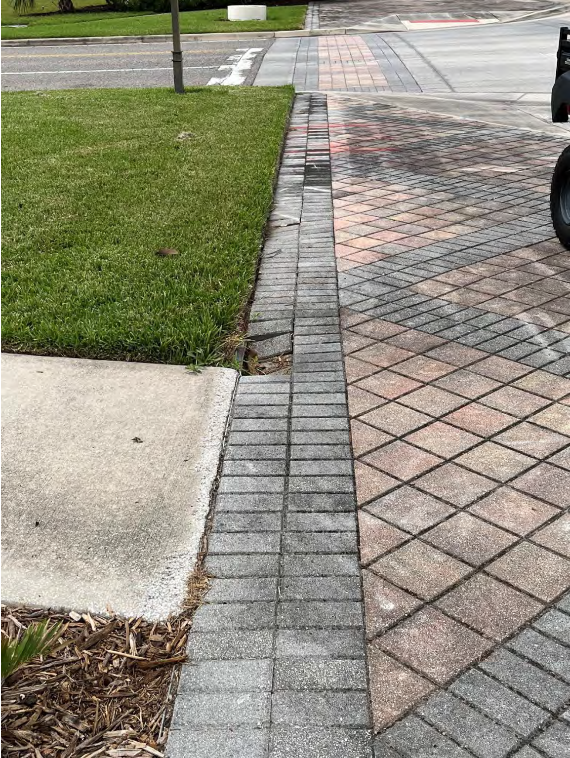
Photo 28 - Paver Base Failure
