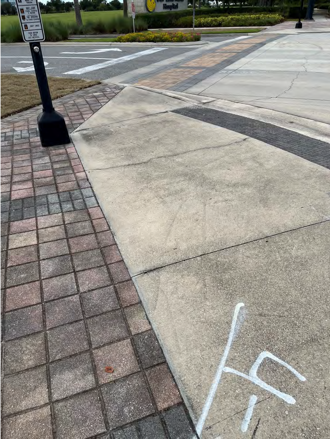
Photo 19 – Surficial Concrete Cracks in Handicap Ramp and Street
