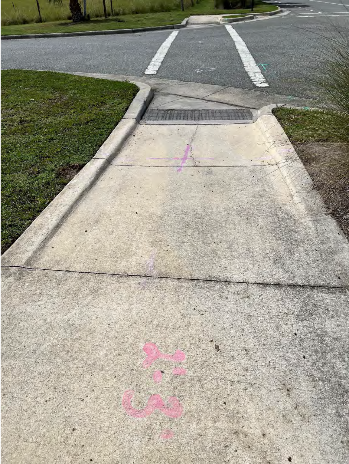
Photo 62 – Surficial Concrete Cracks in Handicap Ramp
