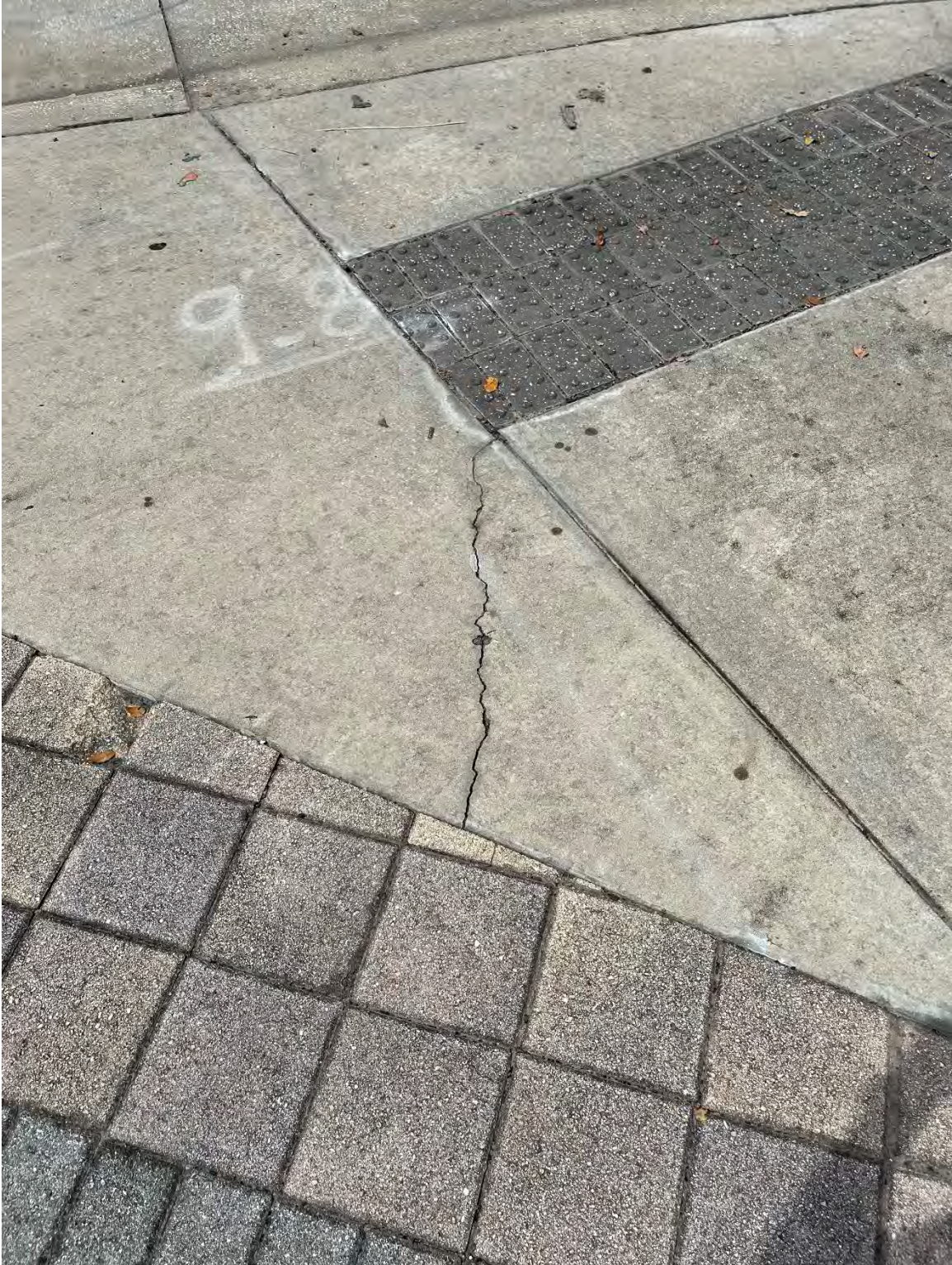
Photo 49 - Surficial Concrete Crack in Handicap Ramp
