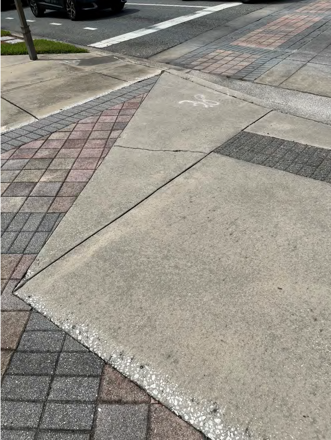
Photo 14 – Surficial Concrete Crack in Handicap Ramp
