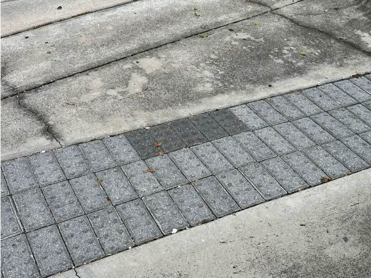
Photo 37 – Surficial Concrete Cracks in Median Strip
