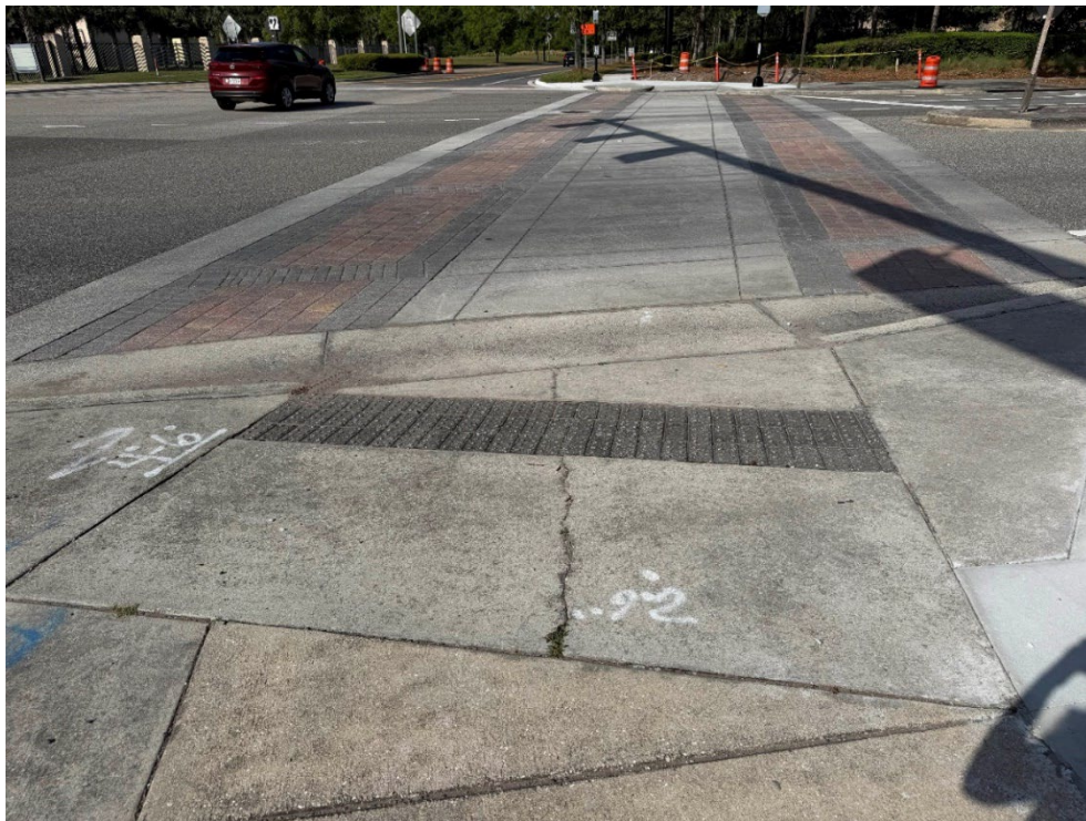
Photo 53.1 – Surficial Concrete Cracks in Handicap Ramp (New Photo – 2026 Assessment)
