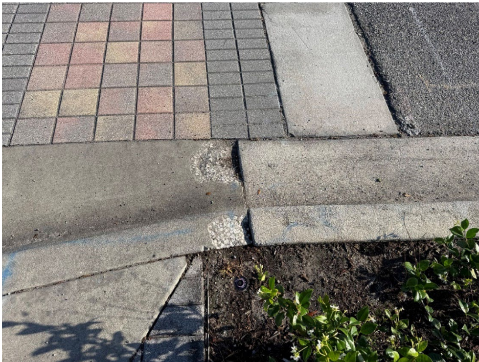
Photo 72.2 – Spalling Concrete, Settling (New Photo – 2026 Assessment)
