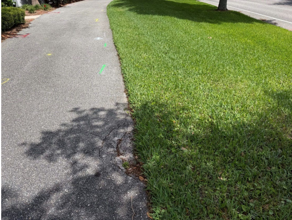
Photo 36 – Raveling Asphalt and Base Failure (No Observed Changes) (Refer to Prior Photo 43- 2025 Assessment)
