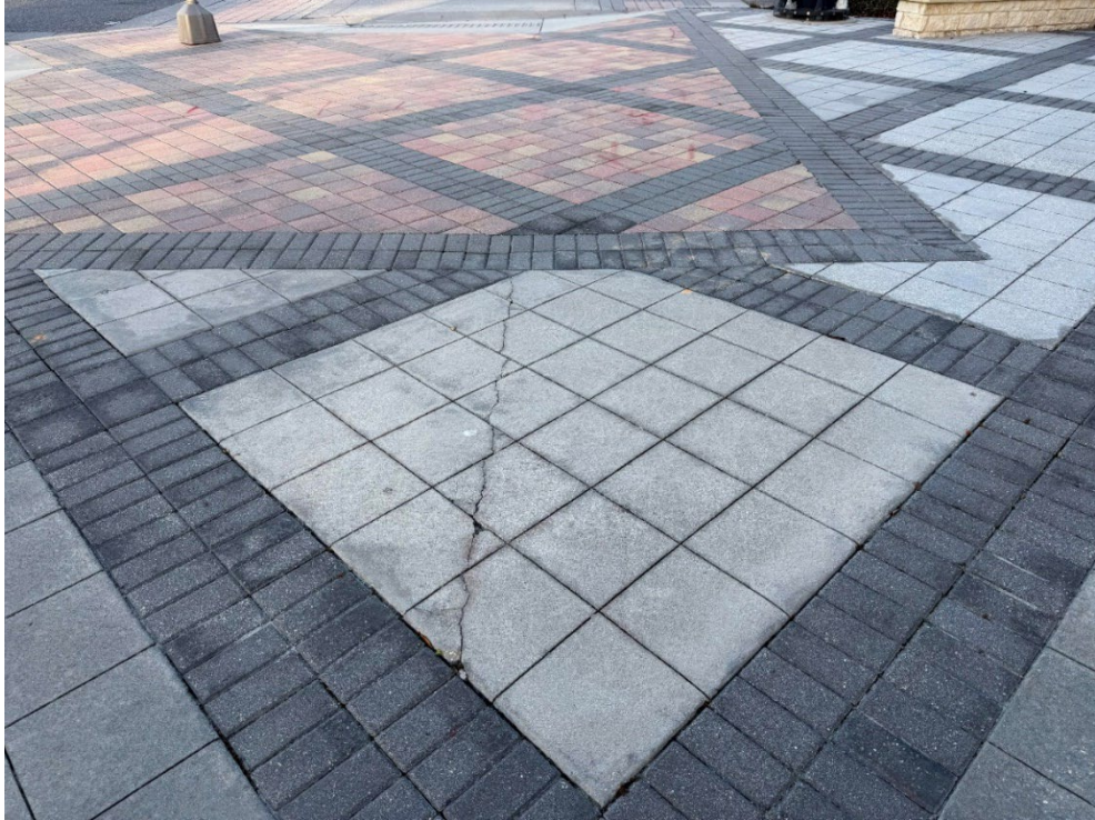
Photo 39 – Multiple Broken Pavers (No Observed Changes) (Refer to Prior Photo 47- 2025 Assessment)
