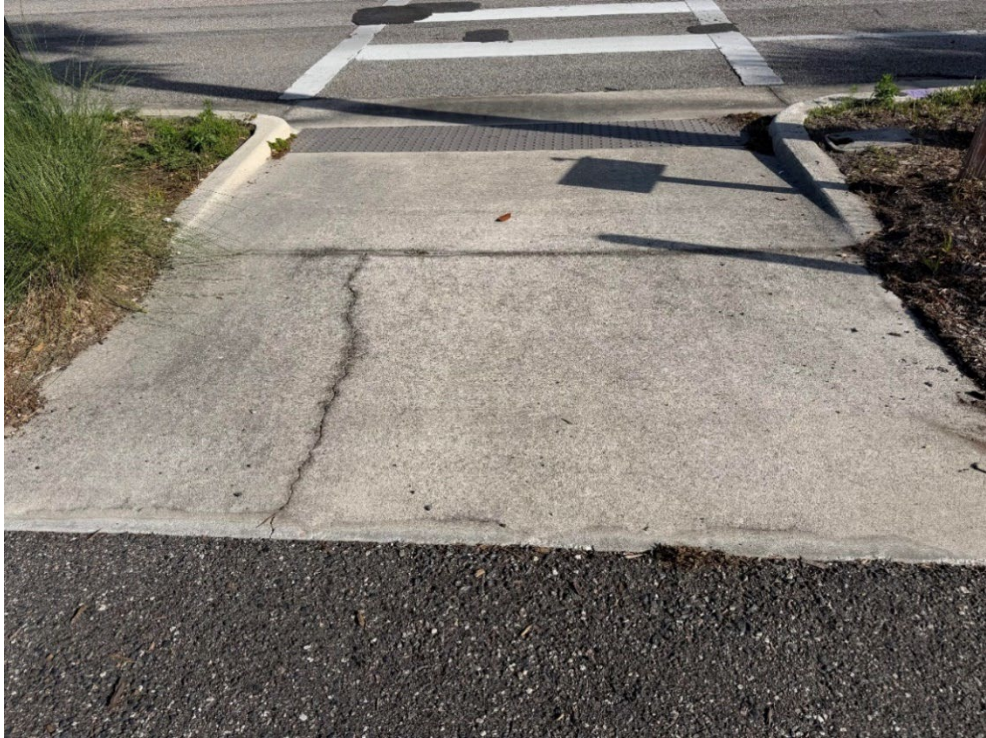
Photo 51 – Surficial Concrete Cracks in Handicap Ramp (No Observed Changes) (Refer to Prior Photo 63 - 2025 Assessment)
