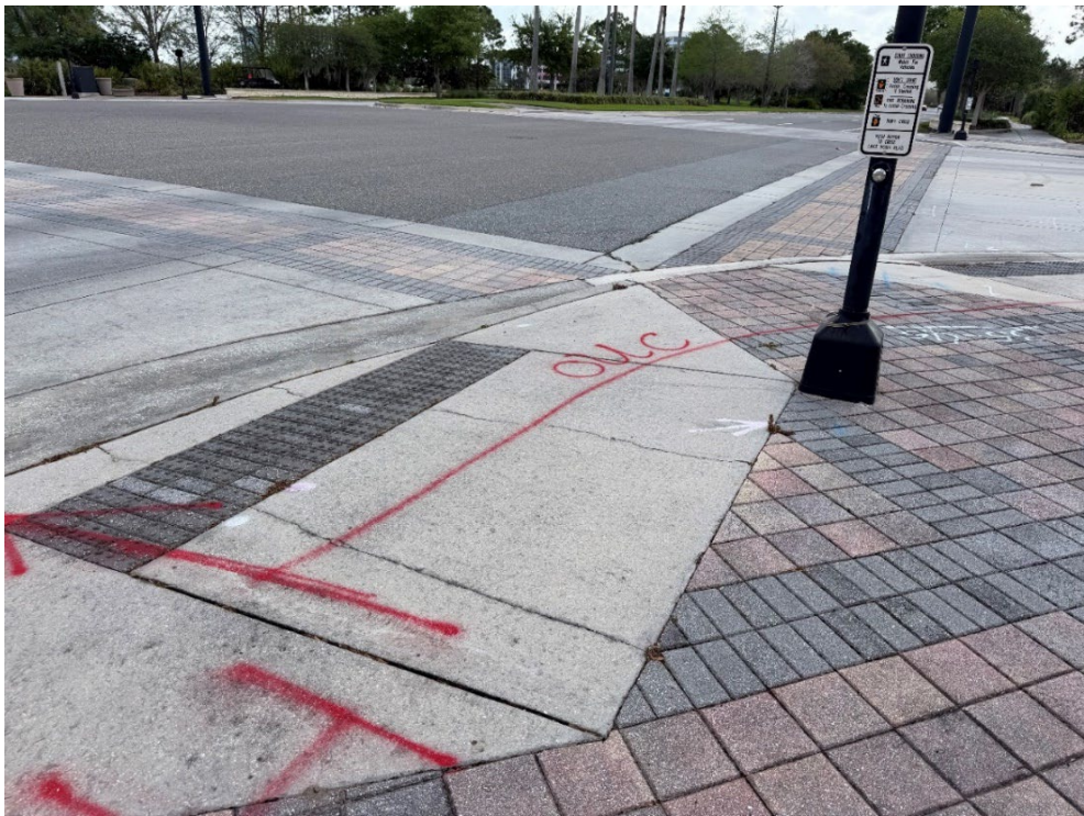
Photo 15 – Surficial Concrete Cracks in Handicap Ramp (No Observed Changes) (Refer to Prior Photo 18- 2025 Assessment)
