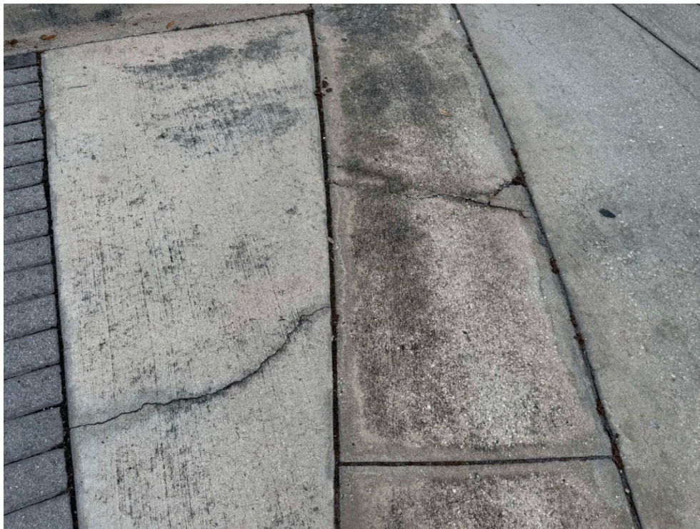
Photo 31 – Surficial Concrete Cracks in Median Strip (No Observed Changes) (Refer to Prior Photo 38- 2025 Assessment)
