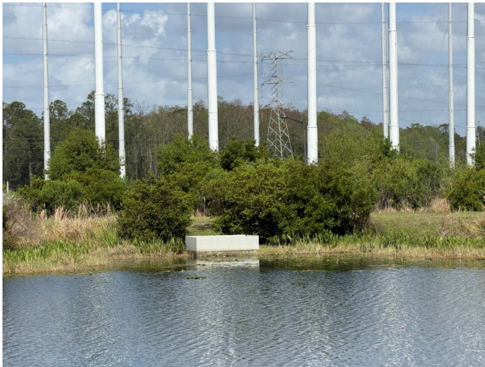
Photo 62 – Outfall Structure View from South Side of Pond Facing NW in Good Condition (No Observed Changes) (Refer to Prior Photo 82- 2025 Assessment)
