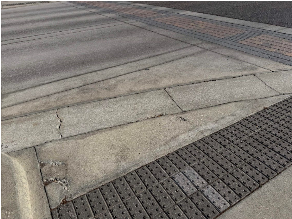
Photo 79.2 – Broken and Spalling Concrete (New Photo – 2026 Assessment)
