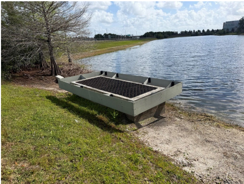
Photo 55 – Pond Outfall Structure in Good Condition (No Observed Changes) (Refer to Prior Photo 73- 2025 Assessment)
