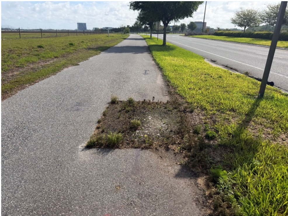
Photo 7 – Asphalt Cutout and Removed (No Observed Changes) (Refer to Prior Photo 9- 2025 Assessment)
