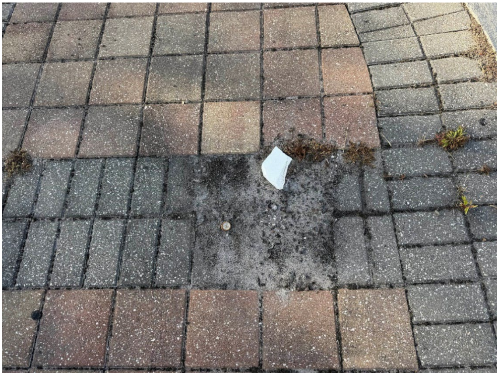
Photo 44 – Paver Base Failure in Median (No Observed Changes) (Refer to Prior Photo 54 – 2025 Assessment)
