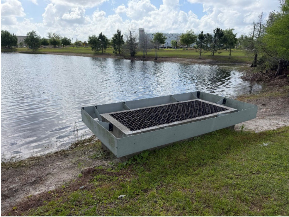
Photo 56 – Pond Outfall Structure in Good Condition (No Observed Changes) (Refer to Prior Photo 74- 2025 Assessment)
