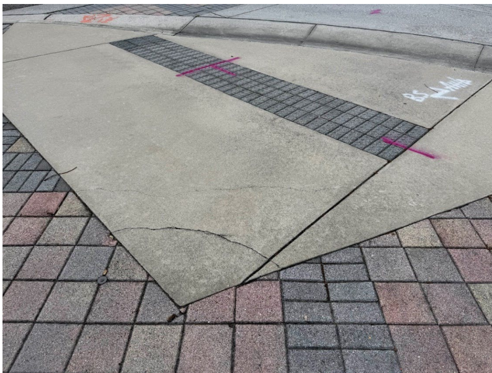
Photo 33 – Surficial Concrete Cracks in Handicap Ramp (No Observed Changes) (Refer to Prior Photo 40- 2025 Assessment)
