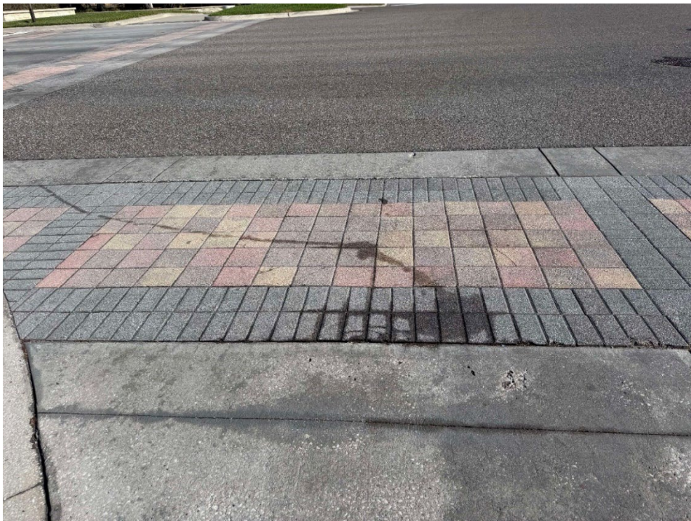
Photo 79 – Cracked Pavers, Some Settling (No Observed Changes) (Refer to Prior Photo 105 - 2025 Assessment)
