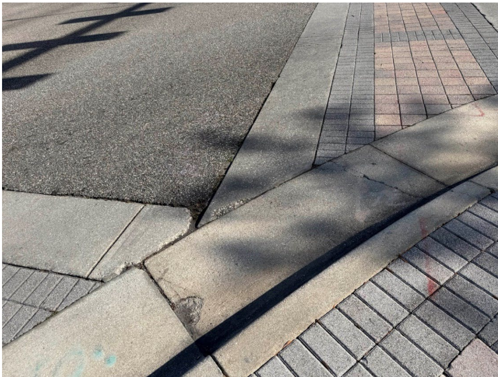
Photo 75.1 – Broken Concrete Ribbon (New Photo – 2026 Assessment)
