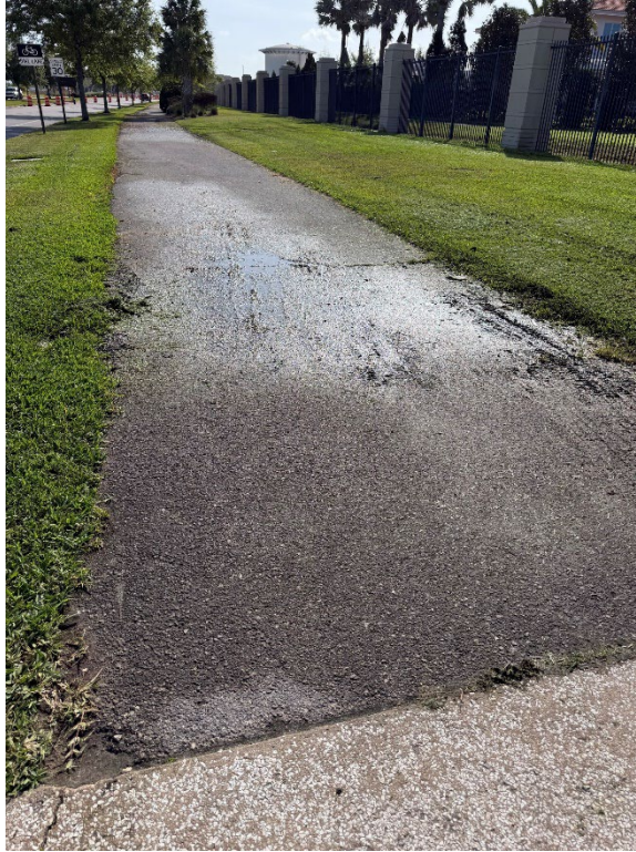
Photo 52.1 – Poor Drainage on Sidewalk (New Photo – 2026 Assessment)
