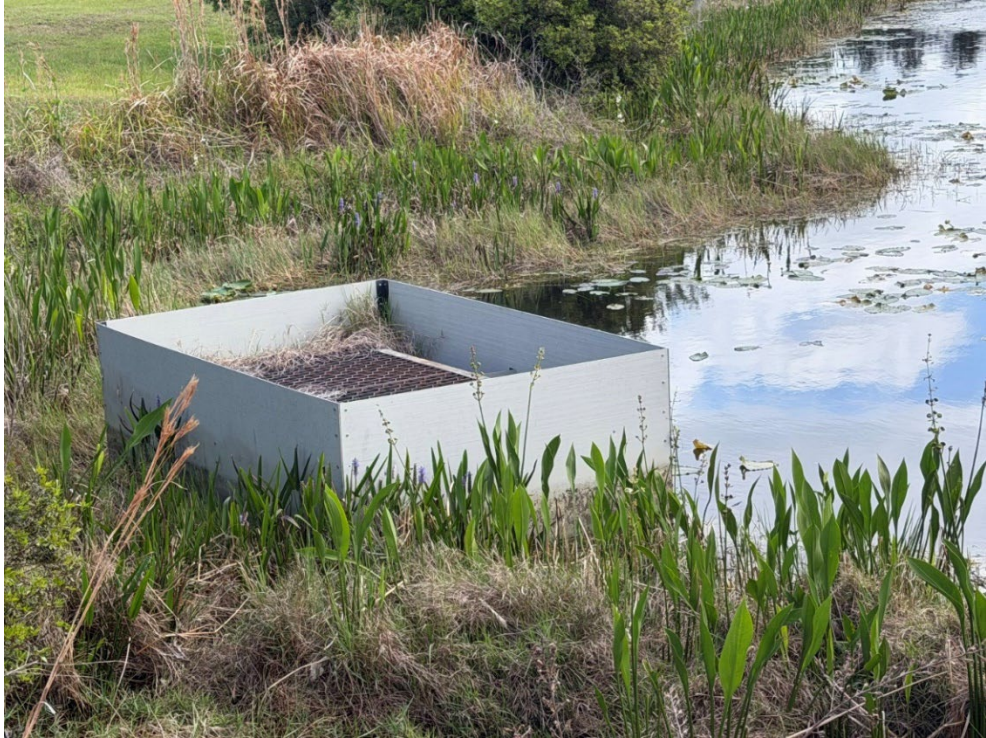
Photo 61.2 – Outfall Structure Containing Vegetation (New Photo – 2026 Assessment)
