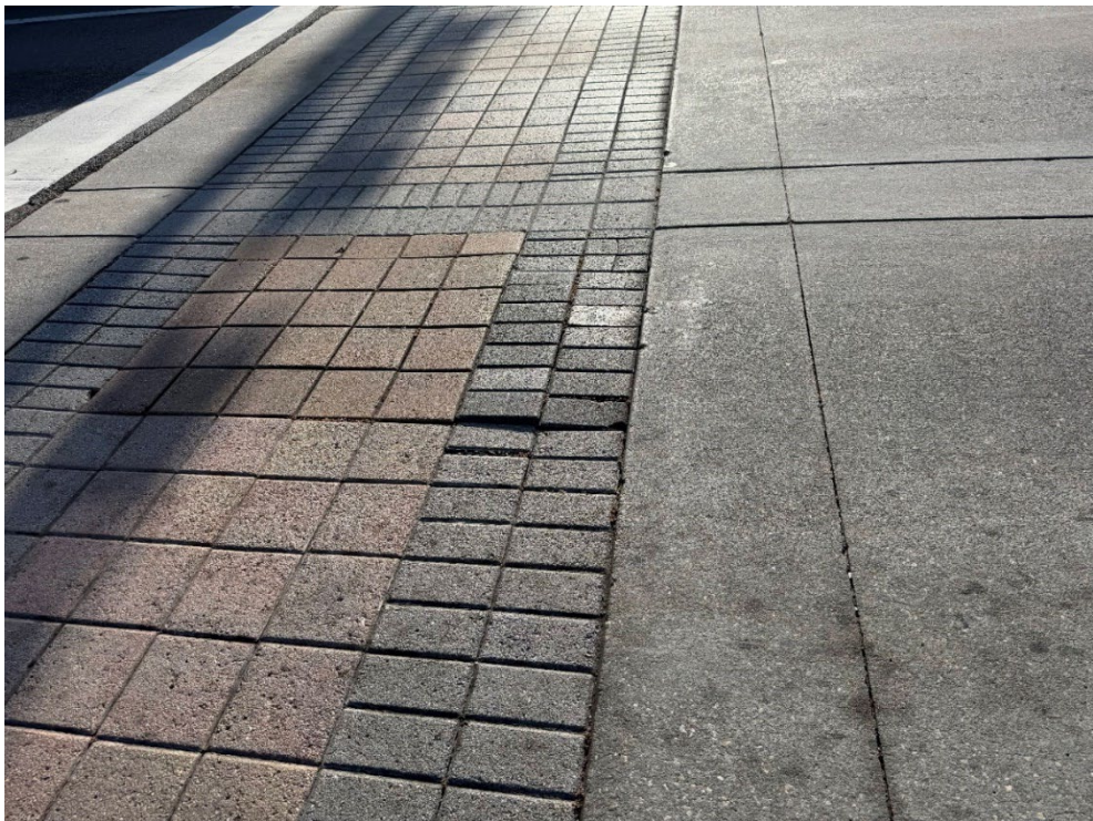
Photo 72 – Surficial Paver Cracks, Minor Settling (No Observed Changes) (Refer to Prior Photo 92- 2025 Assessment)
