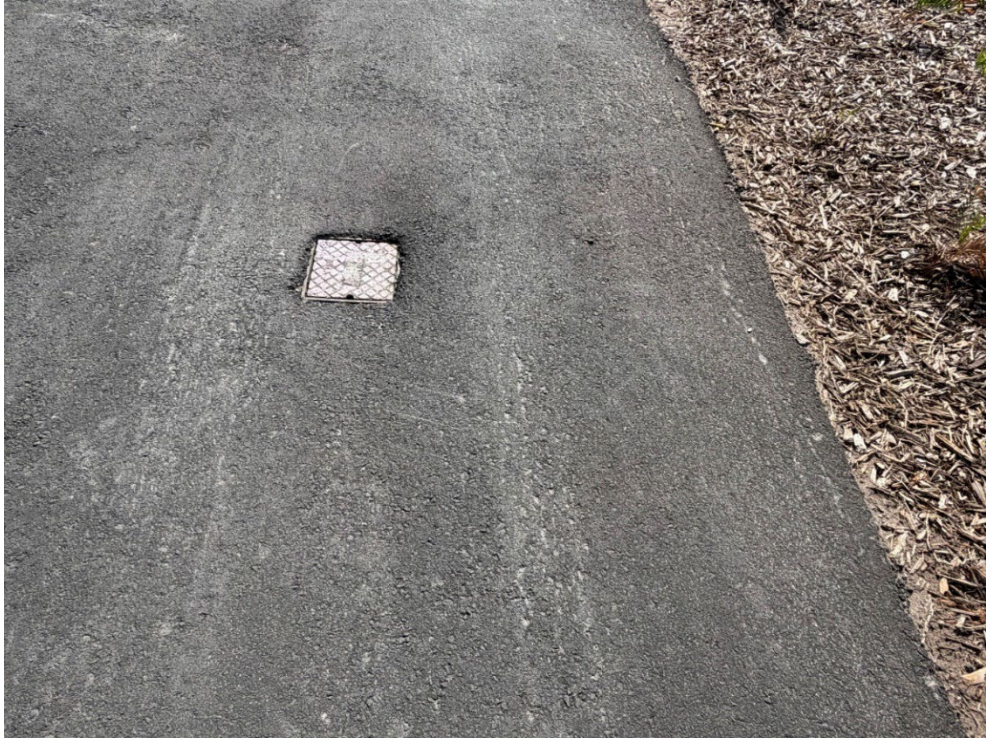
Photo 6 – Sunken Reclaim Water Meter (No Observed Changes) (Refer to Prior Photo 8- 2025 Assessment)
