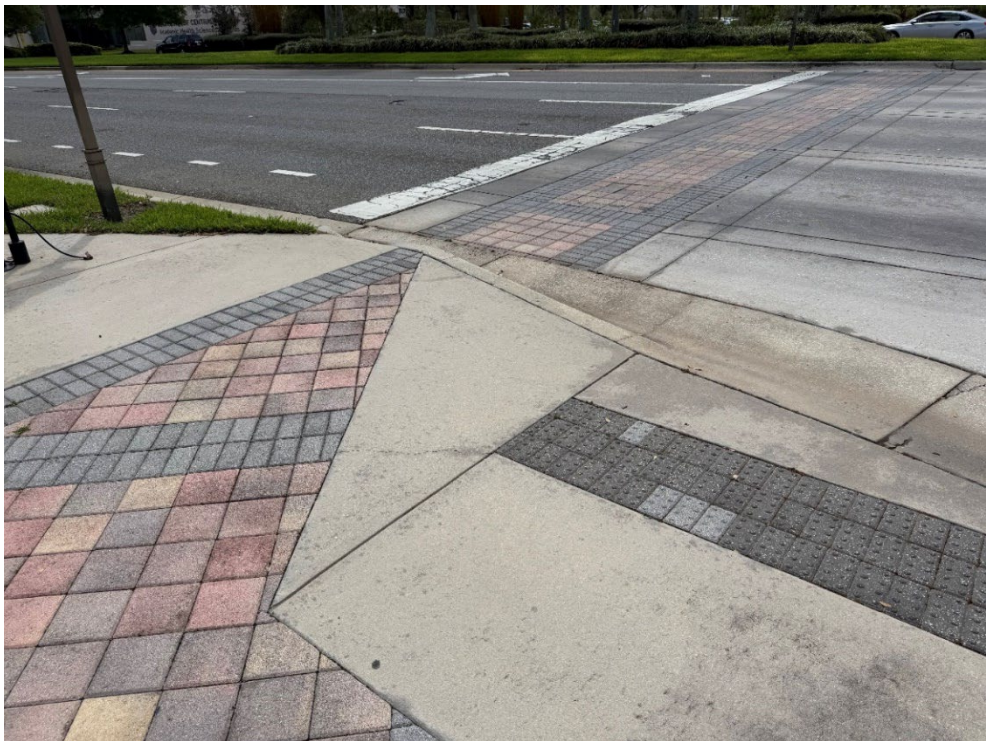
Photo 25 – Surficial Concrete Cracks in Handicap Ramp (No Observed Changes) (Refer to Prior Photo 32- 2025 Assessment)
