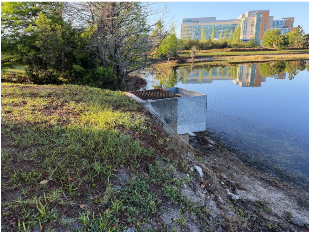
Photo 68 – Outfall Structure in Good Condition (No Observed Changes) (Refer to Prior Photo 88 - 2025 Assessment)
