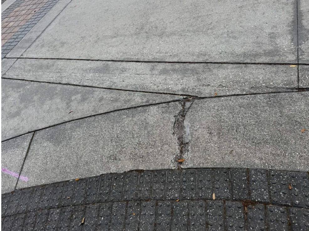
Photo 89 – Construction Entrance – Broken Concrete in Flush Curb (No Observed Changes) (Refer to Prior Photo 120 - 2025 Assessment)
