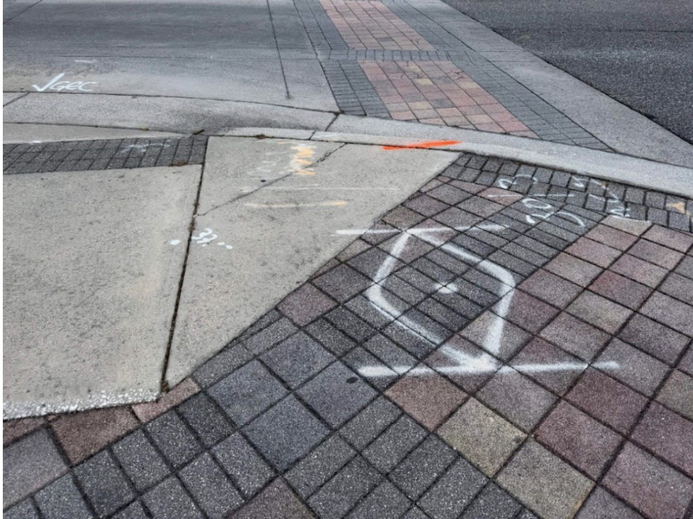
Photo 12 – Surficial Concrete Cracks in Handicap Ramp (No Observed Changes) (Refer to Prior Photo 15- 2025 Assessment)
