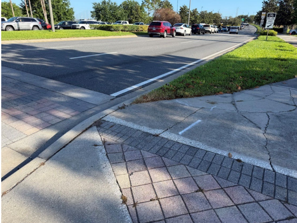
Photo 72.1 – Cracked Concrete, Minor Settling (New Photo – 2026 Assessment)
