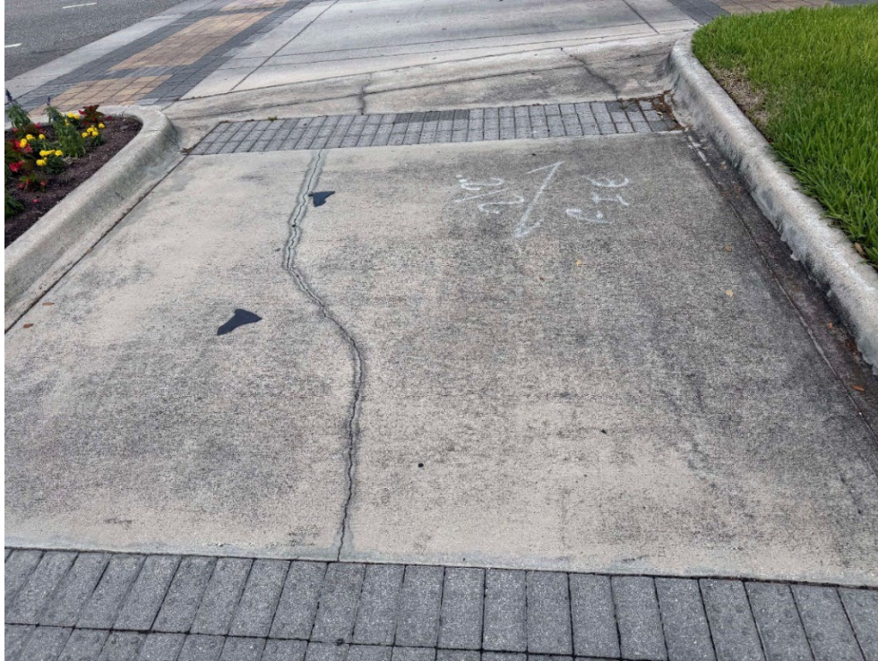
Photo 32 – Surficial Concrete Cracks in Median Strip (No Observed Changes) (Refer to Prior Photo 39- 2025 Assessment)
