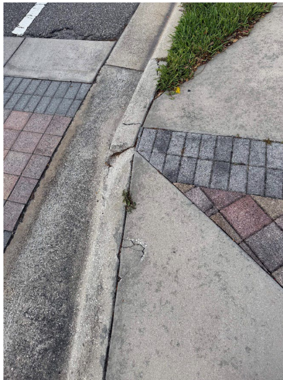
Photo 19 – Cracked and Spalling Concrete in Handicap Ramp (No Observed Changes) (Refer to Prior Photo 23- 2025 Assessment)
