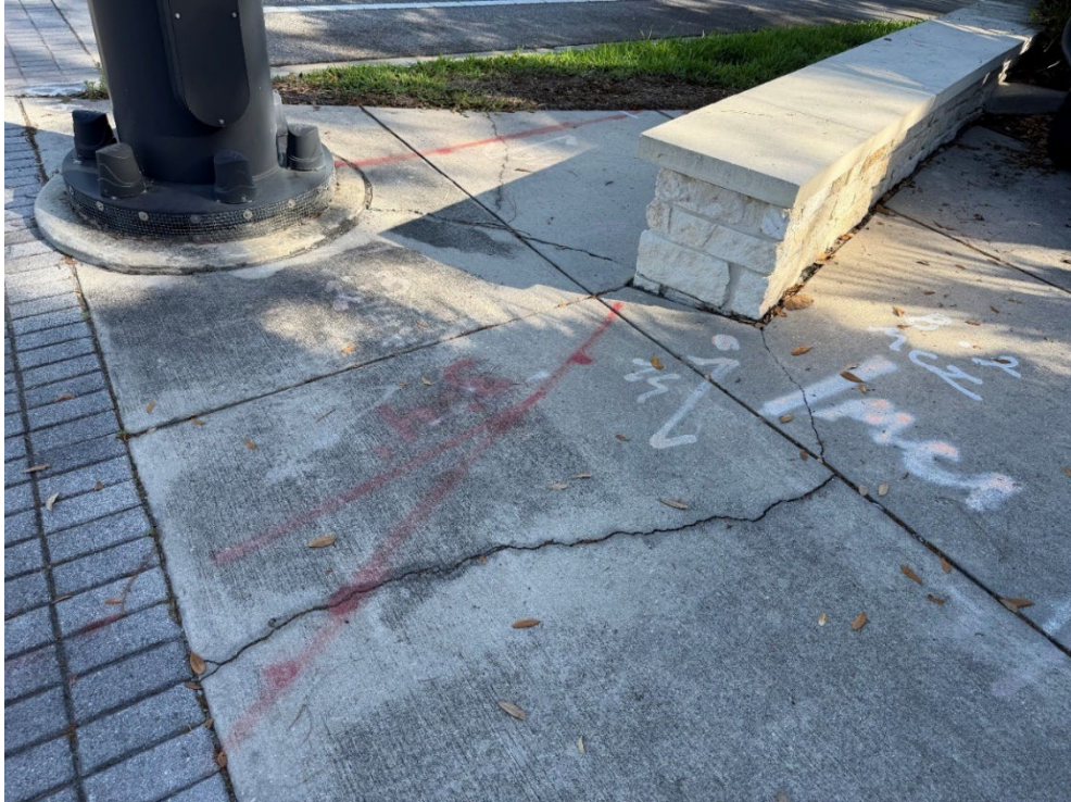
Photo 78.3 – Cracked Concrete in Sidewalk (New Photo – 2026 Assessment)
