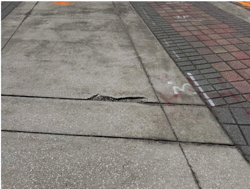
Photo 91 – Broken Concrete (No Observed Changes) (Refer to Prior Photo 124 - 2025 Assessment)
