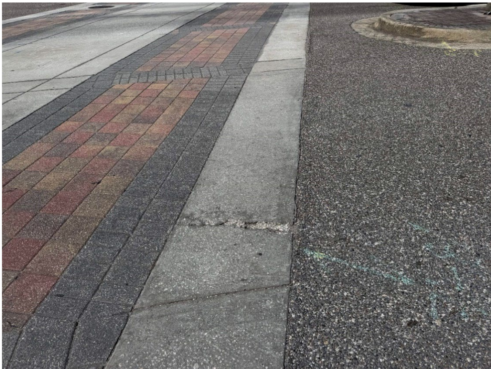
Photo 90 – Broken Concrete (No Observed Changes) (Refer to Prior Photo 122 - 2025 Assessment)
