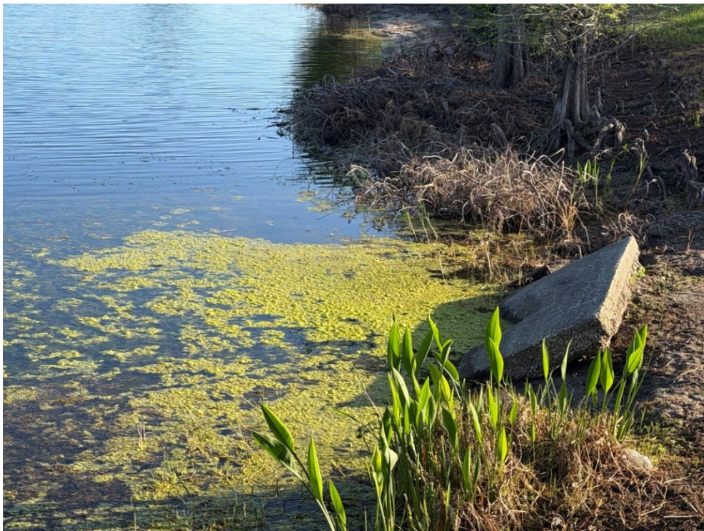
Photo 70.2 – Stormwater Inflow Erosion Behind Mitered End Section (New Photo – 2026 Assessment)
