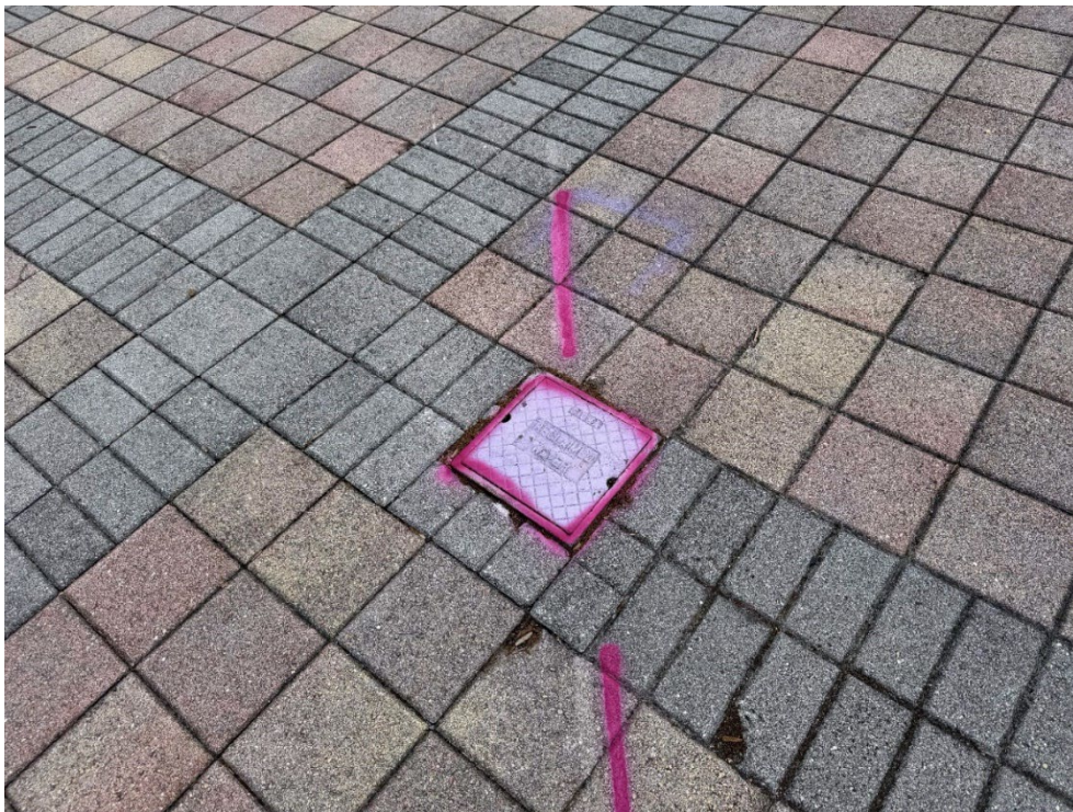
Photo 35 – Raised Reclaim Meter (Approximately ½ -inch) (No Observed Changes) (Refer to Prior Photo 42- 2025 Assessment)
