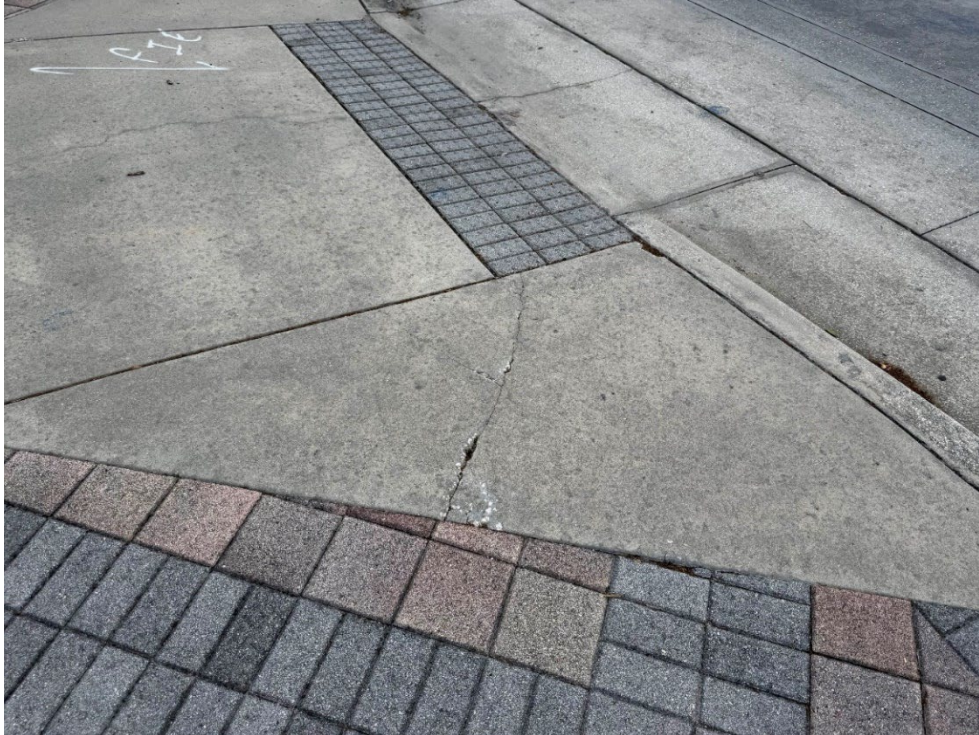
Photo 34 – Surficial Concrete Cracks in Handicap Ramp (No Observed Changes) (Refer to Prior Photo 41- 2025 Assessment)
