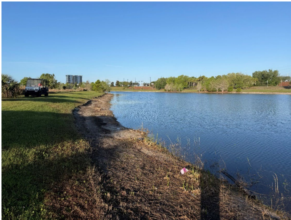
Photo 70 – South Berm Facing West in Good Condition (No Observed Changes) (Refer to Prior Photo 90 - 2025 Assessment)
