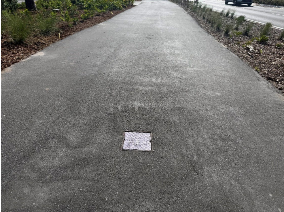
Photo 5 – Sunken Reclaim Water Meter (No Observed Changes) (Refer to Prior Photo 6- 2025 Assessment)
