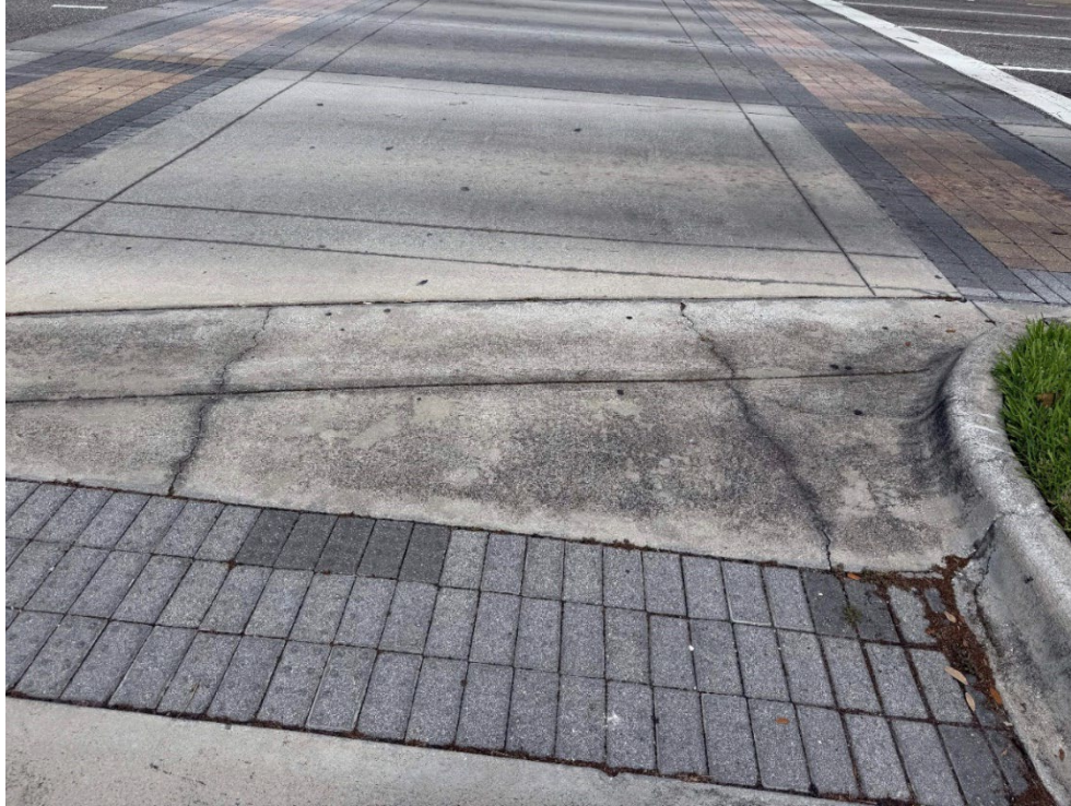
Photo 30 – Surficial Concrete Cracks in Median Strip (No Observed Changes) (Refer to Prior Photo 37- 2025 Assessment)
