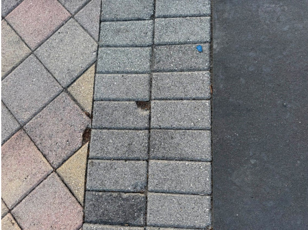
Photo 38 – Multiple Chipped Pavers (No Observed Changes) (Refer to Prior Photo 45- 2025 Assessment)
