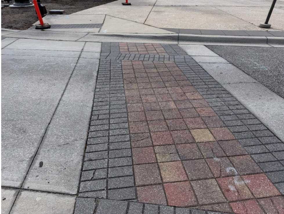
Photo 90.1 – Cracked Pavers (New Photo – 2026 Assessment)
