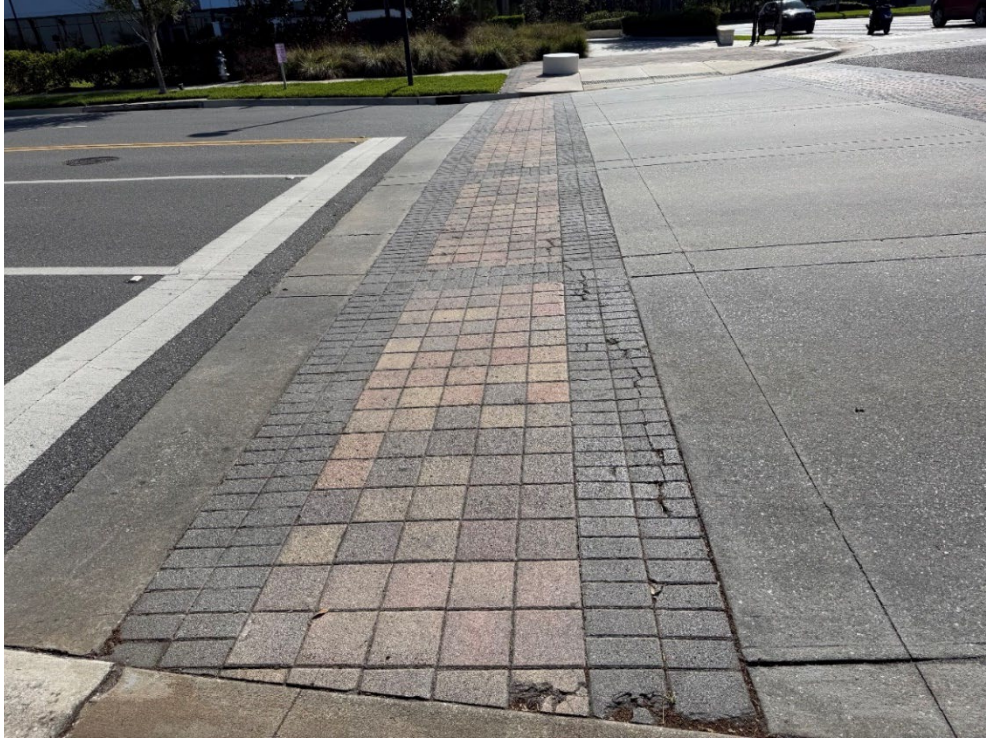
Photo 81 – Cracked and Broken Pavers, Some Settling (No Observed Changes) (Refer to Prior Photo 108 - 2025 Assessment)
