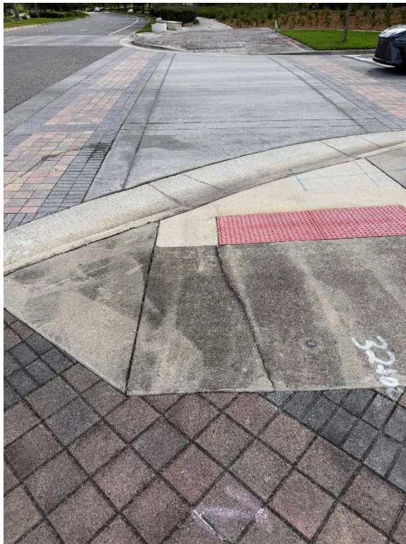
Photo 21 – Surficial Concrete Cracks in Handicap Ramp (No Observed Changes) (Refer to Prior Photo 26- 2025 Assessment)
