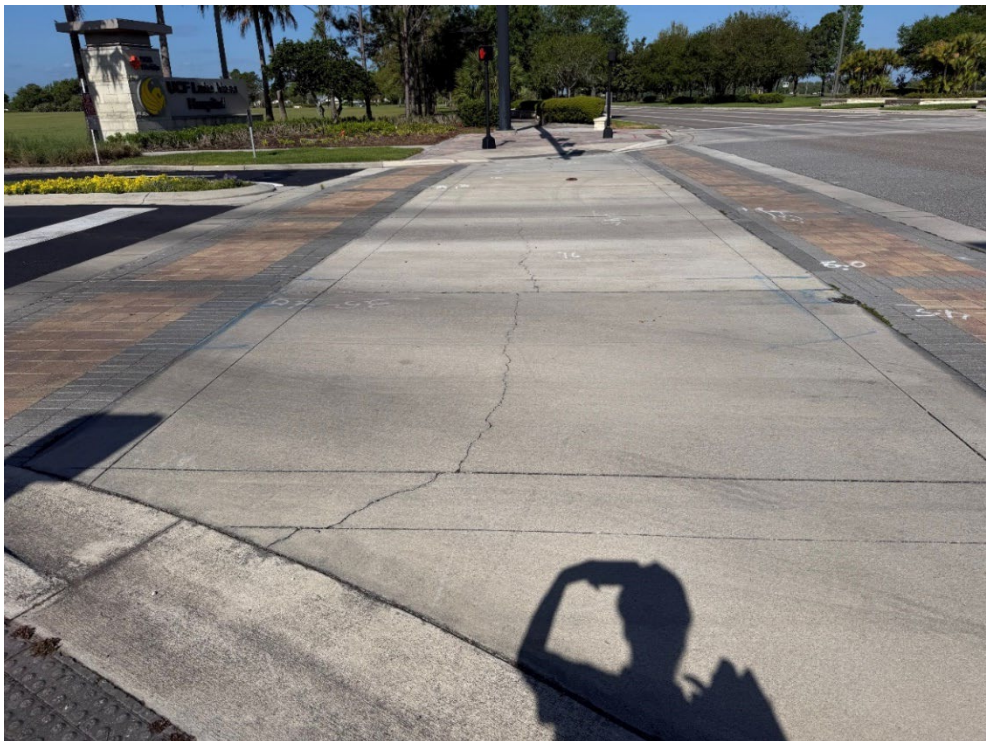
Photo 82 – Surficial Concrete Cracks, Multiple Cracked Pavers, Some Settling (No Observed Changes) (Refer to Prior Photo 109 - 2025 Assessment)
