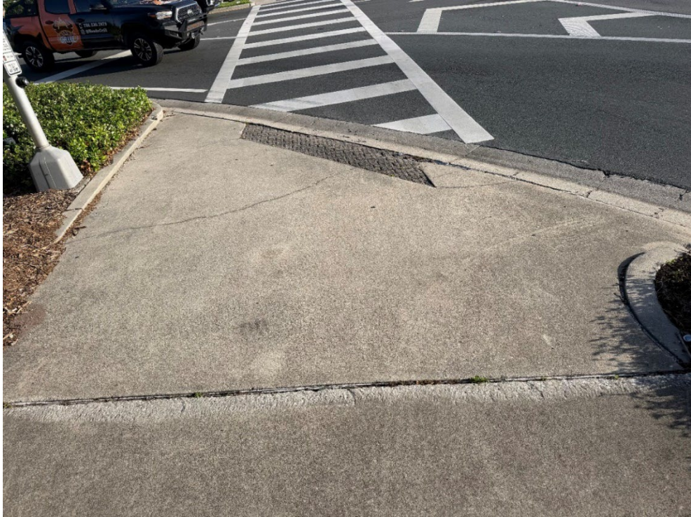
Photo 45 – Surficial Concrete Cracks in Handicap Ramp in Median (No Observed Changes) (Refer to Prior Photo 55- 2025 Assessment)
