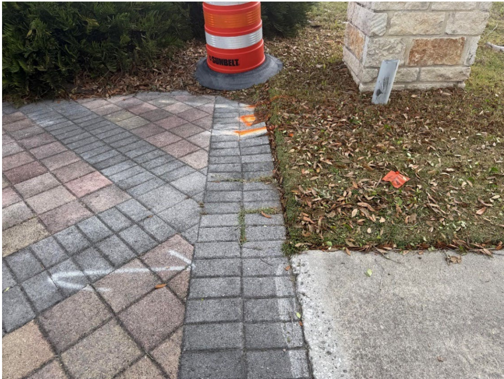
Photo 54 – Paver Base Failure (No Observed Changes) (Refer to Prior Photo 69- 2025 Assessment)
