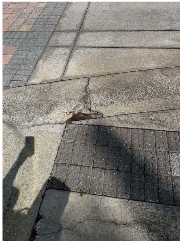
Photo 23 – Cracked Concrete in East Median (No Observed Changes) (Refer to Prior Photo 30- 2025 Assessment)
