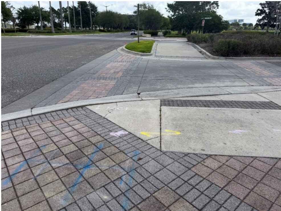
Photo 13 – Surficial Concrete Cracks in Handicap Ramp (No Observed Changes) (Refer to Prior Photo 16- 2025 Assessment)
