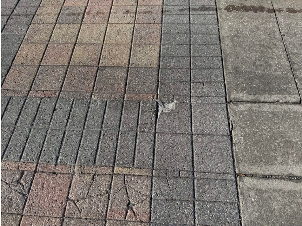
Photo 73 – Cracked Pavers, Minor Settling (No Observed Changes) (Refer to Prior Photo 95 - 2025 Assessment)
