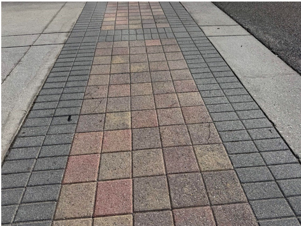
Photo 78 – Cracked Pavers, Minor Settling (No Observed Changes) (Refer to Prior Photo 102 - 2025 Assessment)
