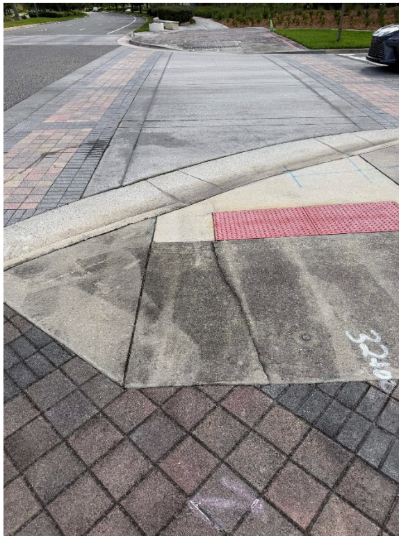
Photo 21 – Surficial Concrete Cracks in Handicap Ramp (No Observed Changes) (Refer to Prior Photo 26- 2025 Assessment)
