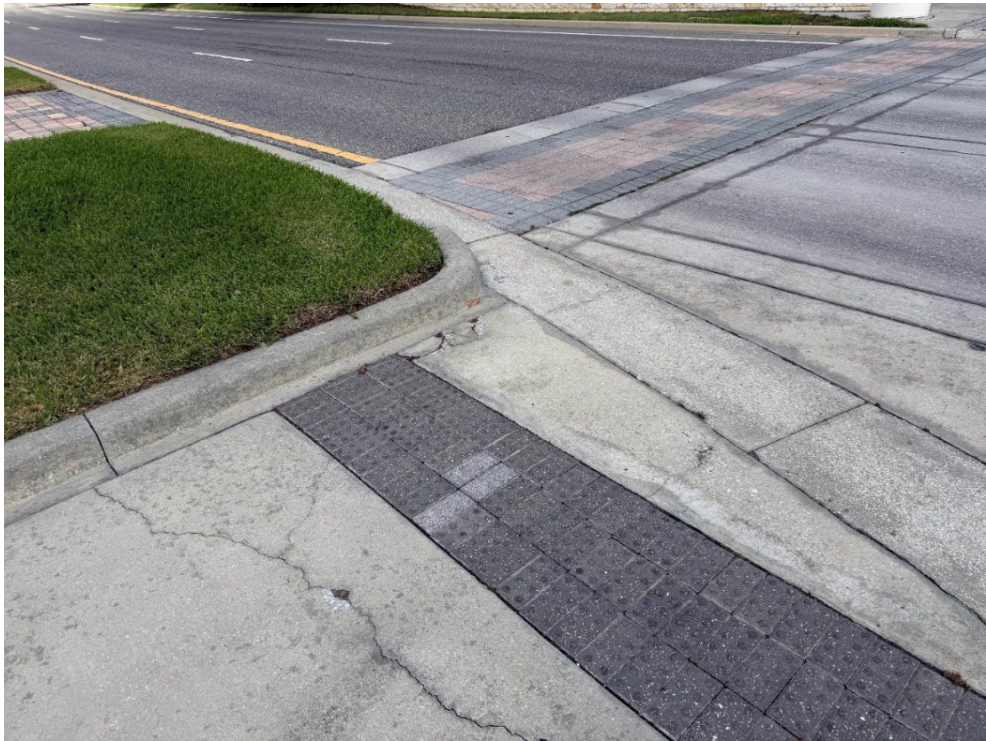
Photo 17 – Surficial Concrete Cracks in Handicap Ramp (No Observed Changes) (Refer to Prior Photo 21- 2025 Assessment)
