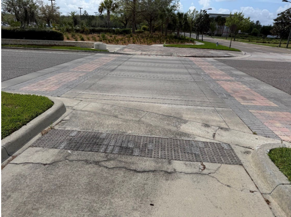
Photo 22 – Surficial Concrete Cracks in Handicap Ramp (No Observed Changes) (Refer to Prior Photo 29- 2025 Assessment)
