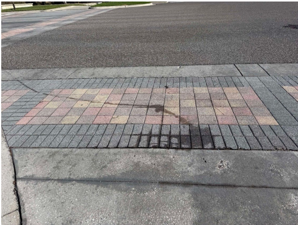
Photo 79 – Cracked Pavers, Some Settling (No Observed Changes) (Refer to Prior Photo 105 - 2025 Assessment)
