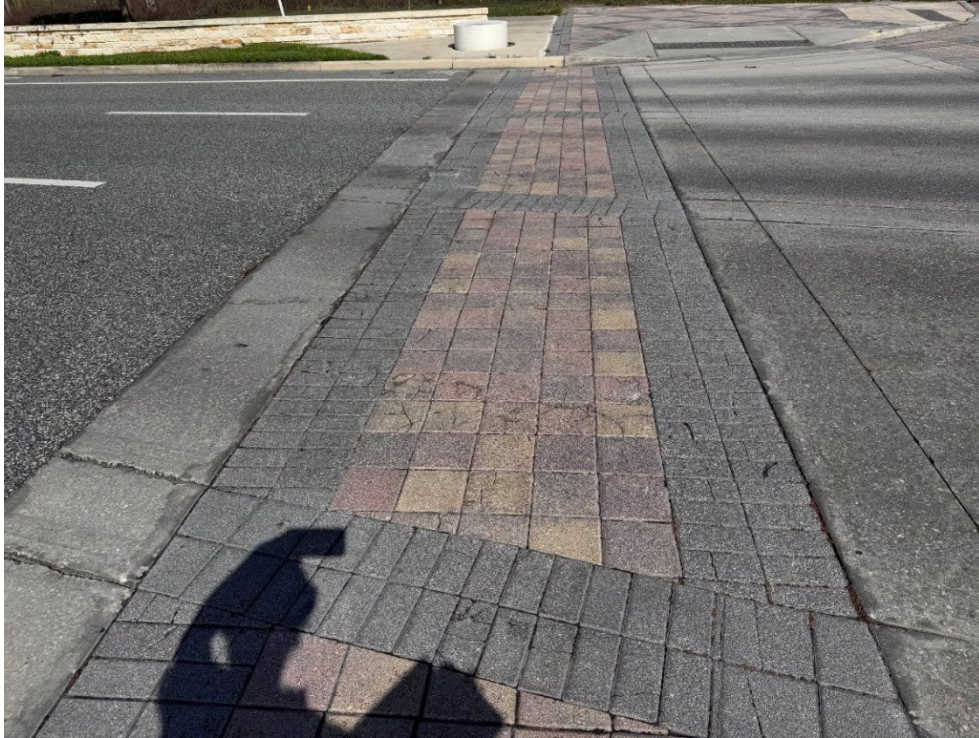
Photo 85.1 – Multiple Cracked Concrete, Pavers Settling, Broken Flush Curb (New Photo – 2026 Assessment)
