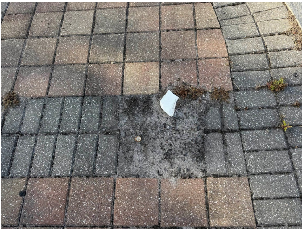
Photo 44 – Paver Base Failure in Median (No Observed Changes) (Refer to Prior Photo 54 – 2025 Assessment)
