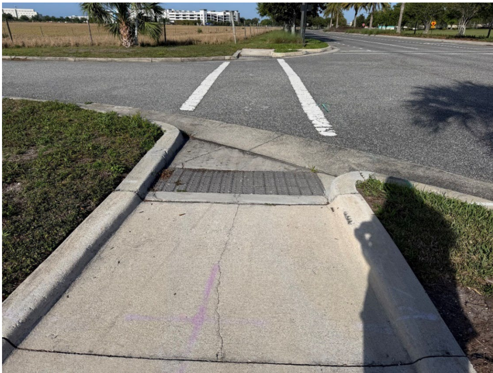
Photo 50 – Surficial Concrete Cracks in Handicap Ramp (No Observed Changes) (Refer to Prior Photo 61 and 62- 2025 Assessment)
