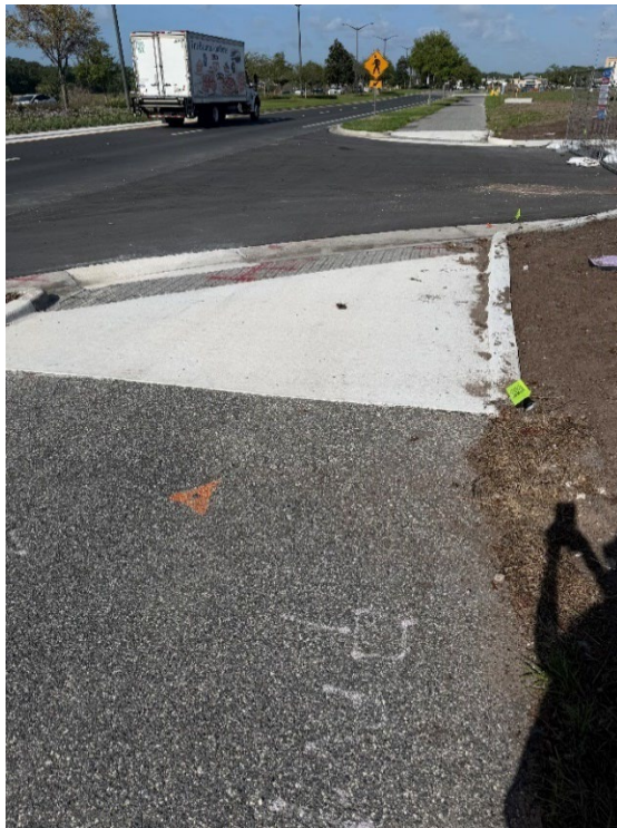
Photo 2 – Surficial Concrete Cracks in Curb Ramp -Construction Ongoing (Concrete Cracked in Curb Ramp Has Been Corrected) (Refer to Prior Photo 3- 2025 Assessment)
