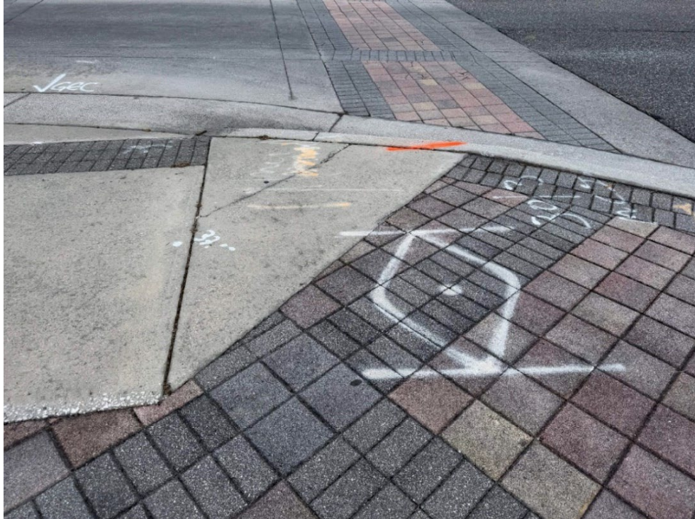
Photo 12 – Surficial Concrete Cracks in Handicap Ramp (No Observed Changes) (Refer to Prior Photo 15- 2025 Assessment)
