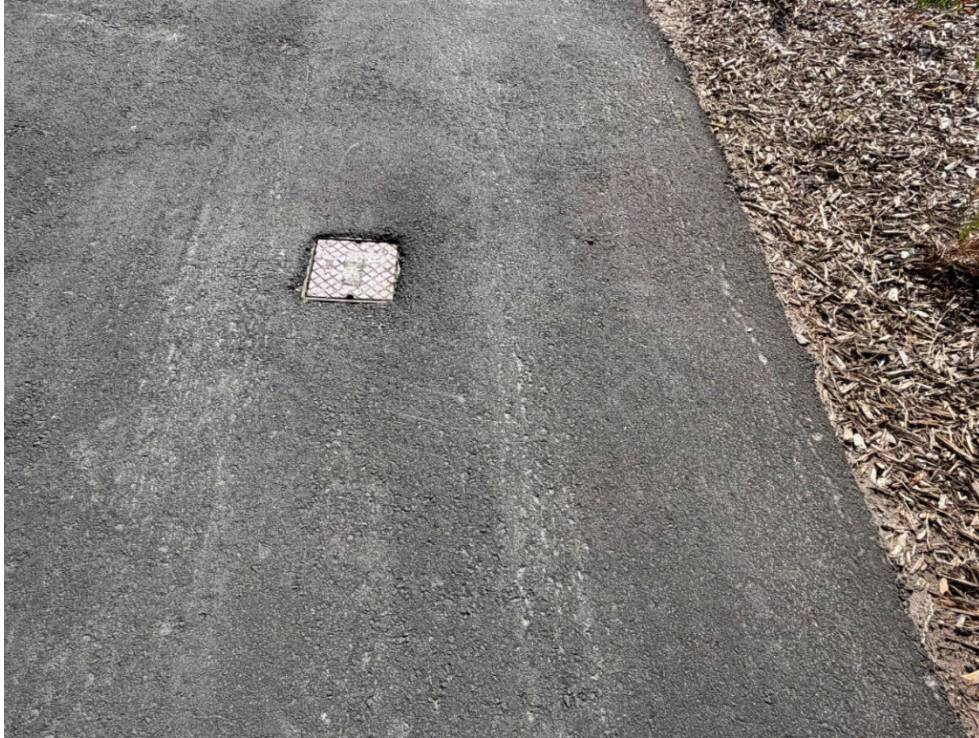
Photo 6 – Sunken Reclaim Water Meter (No Observed Changes) (Refer to Prior Photo 8- 2025 Assessment)
