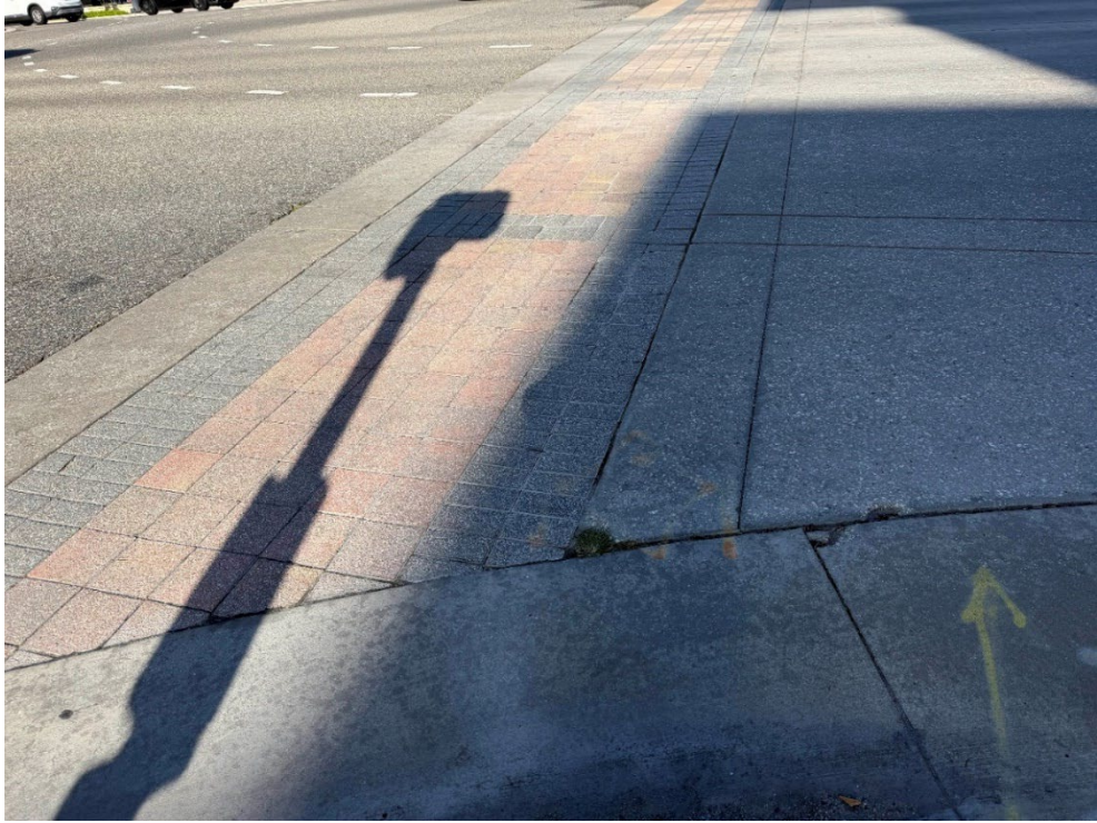
Photo 76 – Cracked Pavers, Broken Concrete (No Observed Changes) (Refer to Prior Photo 98 - 2025 Assessment)
