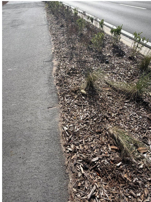
Photo 5.1 – Damaged Asphalt (New Photo – 2026 Assessment)
