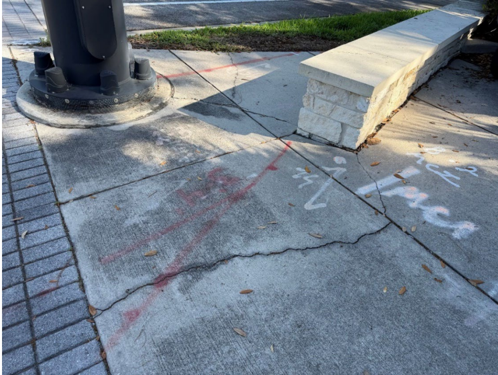
Photo 78.3 – Cracked Concrete in Sidewalk (New Photo – 2026 Assessment)
