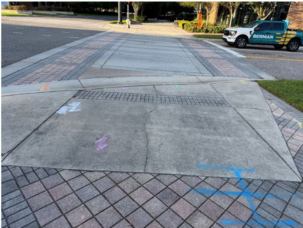
Photo 40 – Surficial Concrete Cracks in Handicap Ramp (No Observed Changes) (Refer to Prior Photo 48- 2025 Assessment)
