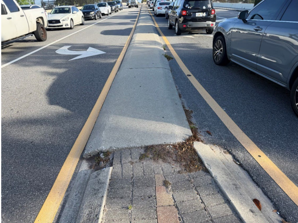
Photo 47 – Paver Base Failure in North Median Looking North (No Observed Changes) (Refer to Prior Photo 57- 2025 Assessment)
