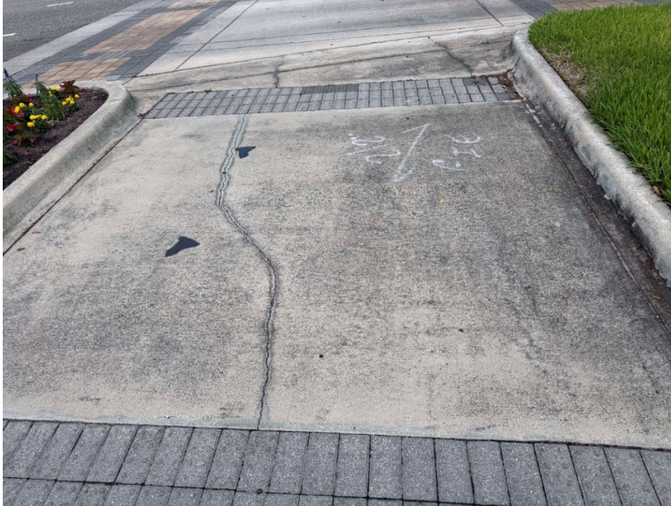
Photo 32 – Surficial Concrete Cracks in Median Strip (No Observed Changes) (Refer to Prior Photo 39- 2025 Assessment)
