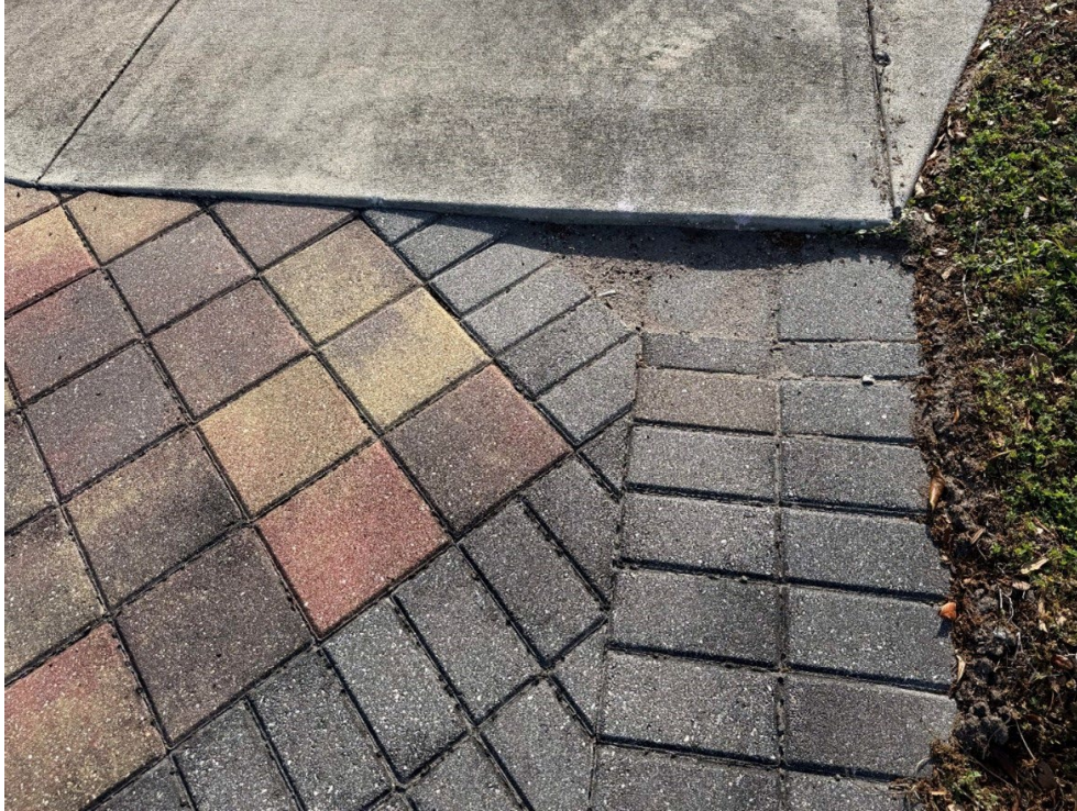
Photo 49 – Paver Base Failure (No Observed Changes) (Refer to Prior Photo 59- 2025 Assessment)
