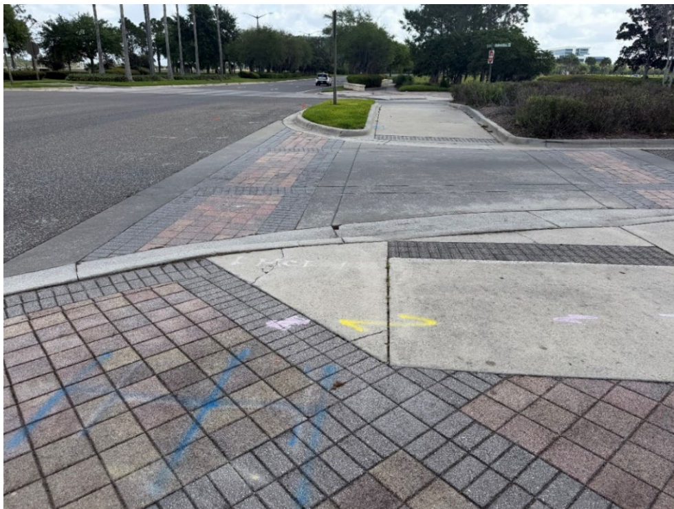
Photo 13 – Surficial Concrete Cracks in Handicap Ramp (No Observed Changes) (Refer to Prior Photo 16- 2025 Assessment)
