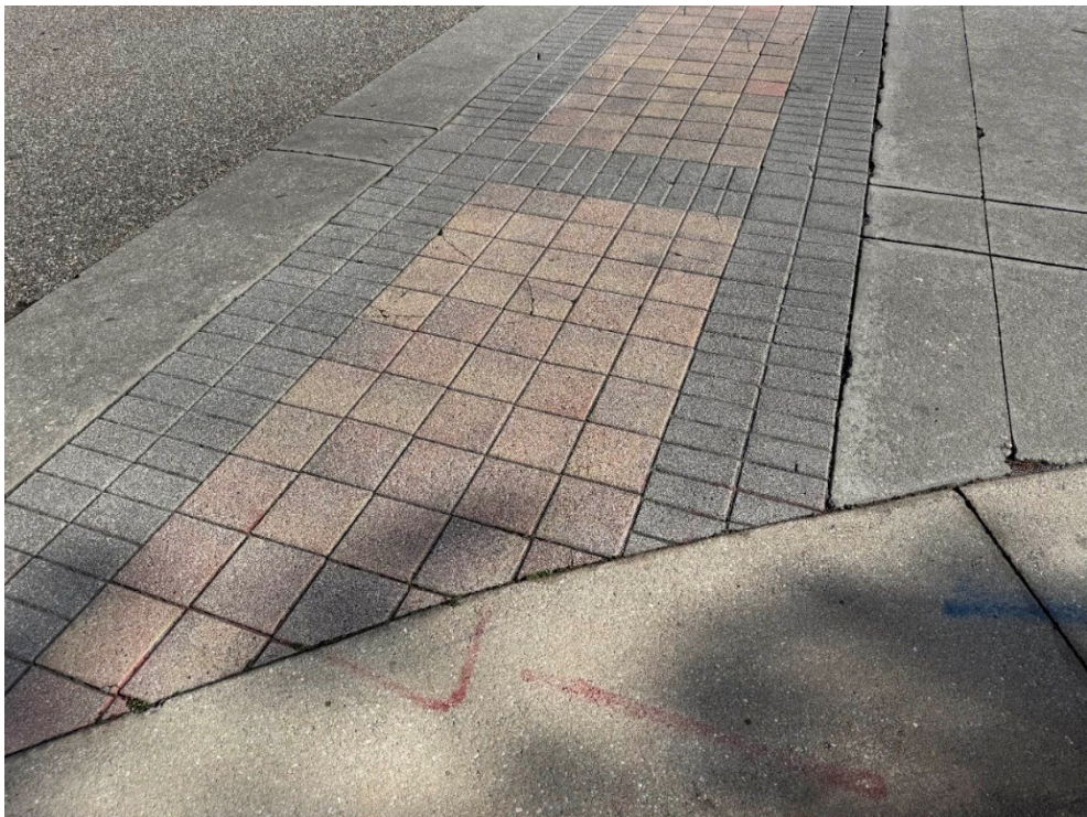
Photo 74 – Cracked Pavers (No Observed Changes) (Refer to Prior Photo 96- 2025 Assessment)
