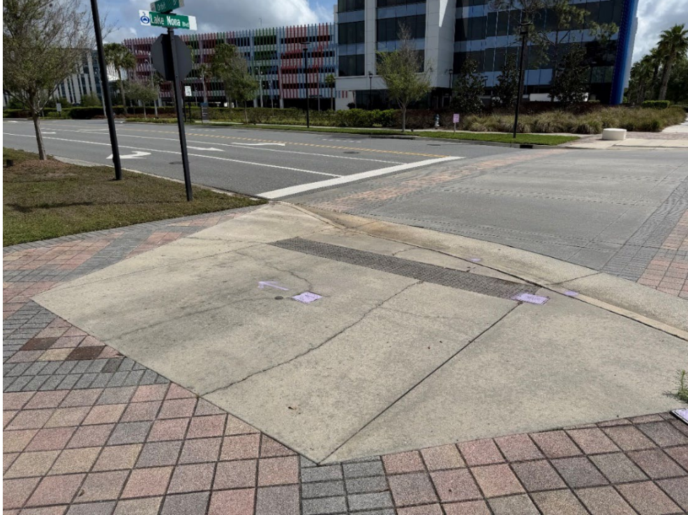
Photo 16 – Surficial Concrete Cracks in Handicap Ramp (No Observed Changes) (Refer to Prior Photo 20- 2025 Assessment)
