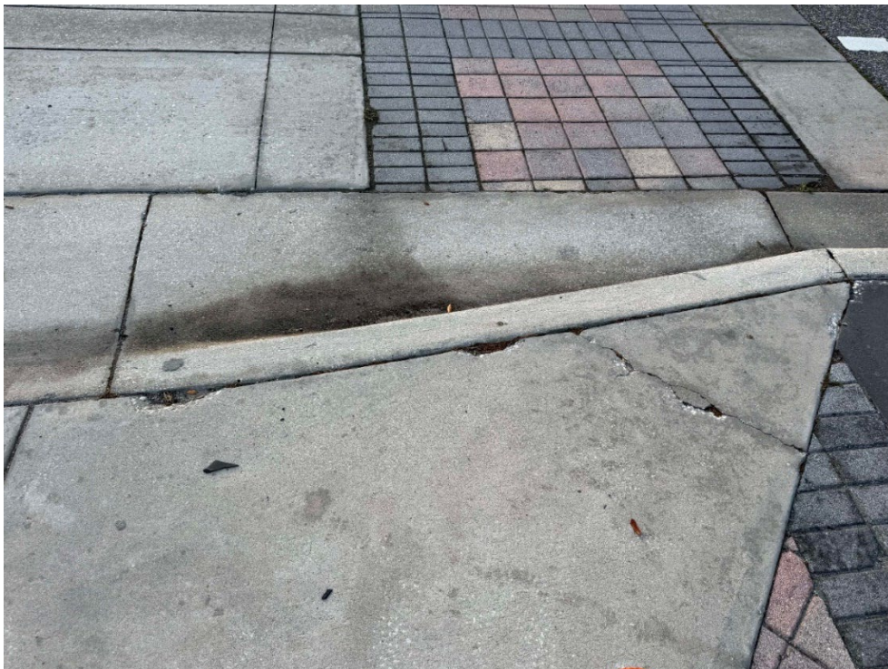
Photo 38.1 – Surficial Concrete Cracks and Spalling in Handicap Ramp (New Photo – 2026 Assessment)
