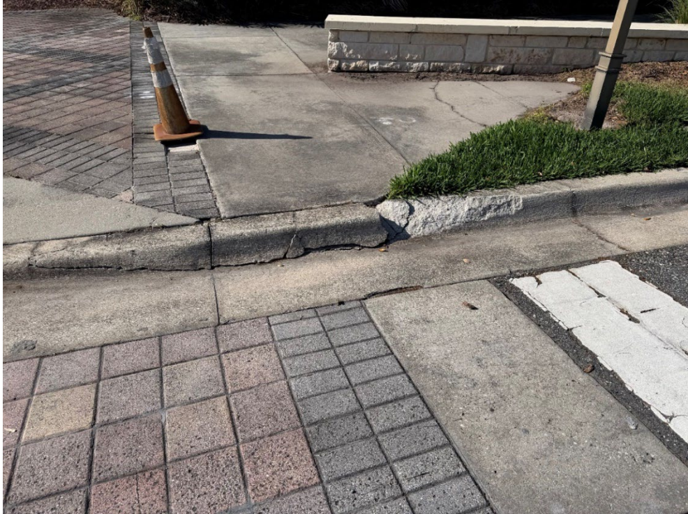
Photo 79.1 – Broken Curb, Cracked Pavers and Surficial Concrete Cracks (New Photo – 2026 Assessment)
