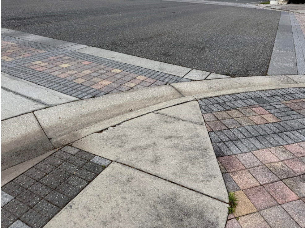
Photo 24 – Surficial Concrete Cracks in Handicap Ramp (No Observed Changes) (Refer to Prior Photo 31- 2025 Assessment)
