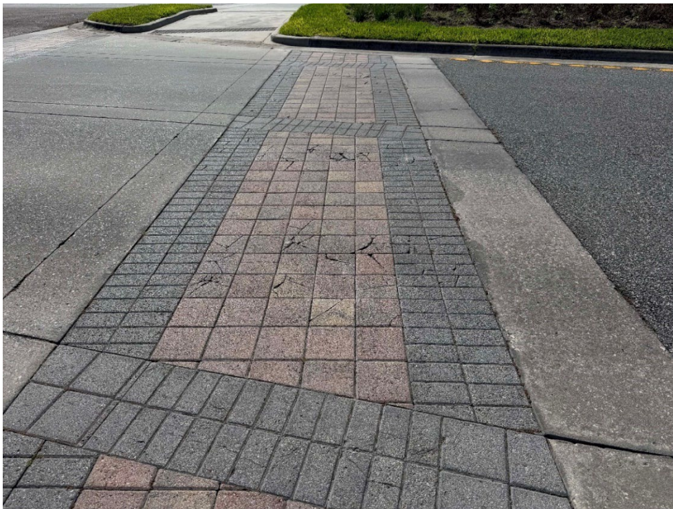
Photo 85 – Multiple Cracked Concrete, Pavers Settling, Broken Flush Curb (No Observed Changes) (Refer to Prior Photo 113 - 2025 Assessment)
