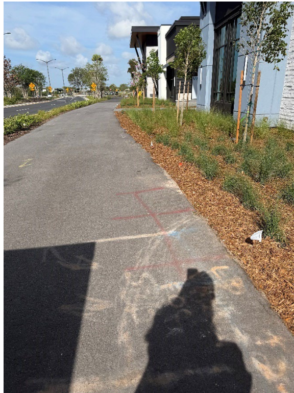
Photo 4 – Asphalt Damage - Construction Ongoing (Asphalt Damage Has Been Corrected) (Refer to Prior Photo 5- 2025 Assessment)
