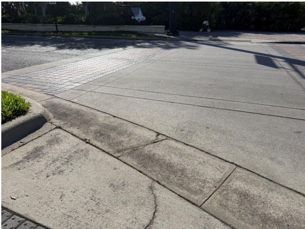
Photo 78.2 – Cracked Concrete (New Photo – 2026 Assessment)
