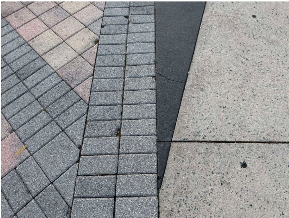
Photo 37 – Multiple Chipped Pavers (No Observed Changes) (Refer to Prior Photo 44- 2025 Assessment)
