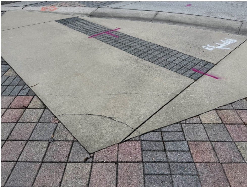
Photo 33 – Surficial Concrete Cracks in Handicap Ramp (No Observed Changes) (Refer to Prior Photo 40- 2025 Assessment)
