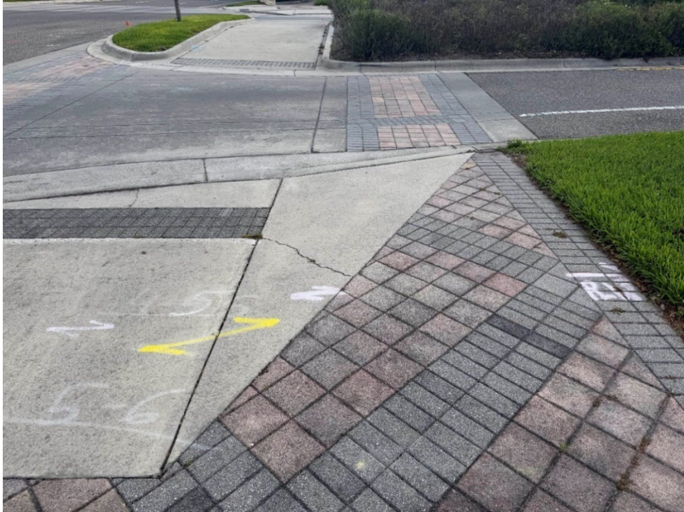
Photo 14 – Surficial Concrete Cracks in Handicap Ramp (No Observed Changes) (Refer to Prior Photo 17 - 2025 Assessment)
