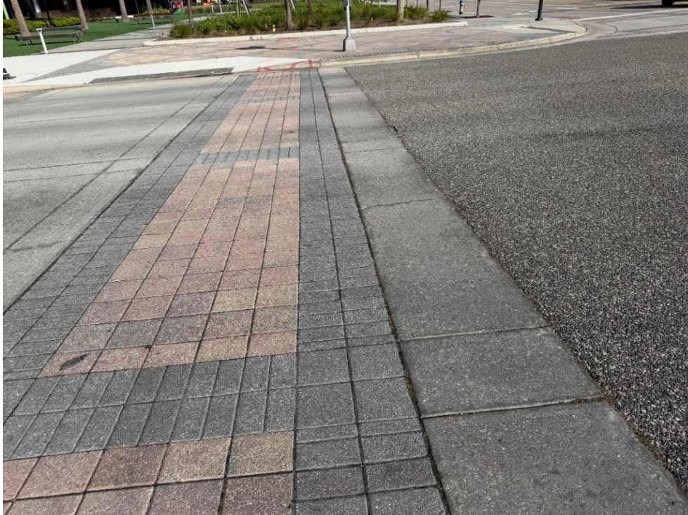
Photo 77 – Cracked Pavers, Minor Settling (No Observed Changes) (Refer to Prior Photo 101 - 2025 Assessment)
