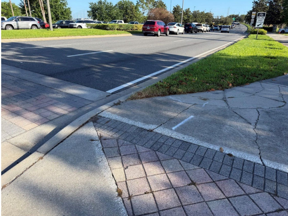
Photo 72.1 – Cracked Concrete, Minor Settling (New Photo – 2026 Assessment)
