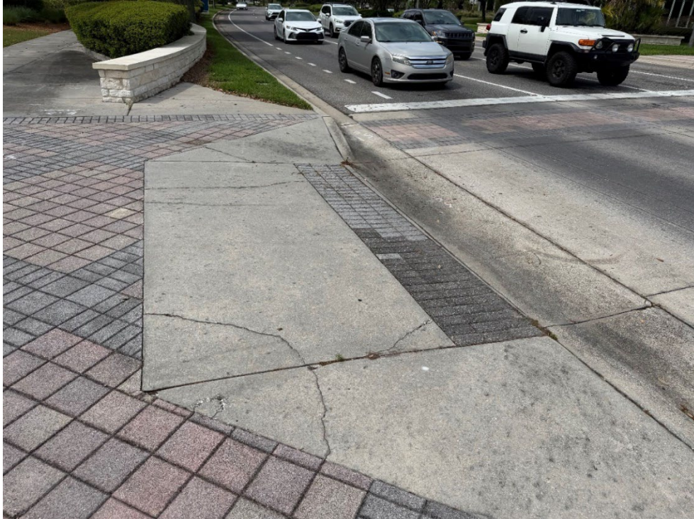
Photo 26 – Surficial Concrete Cracks in Handicap Ramp (No Observed Changes) (Refer to Prior Photo 33- 2025 Assessment)
