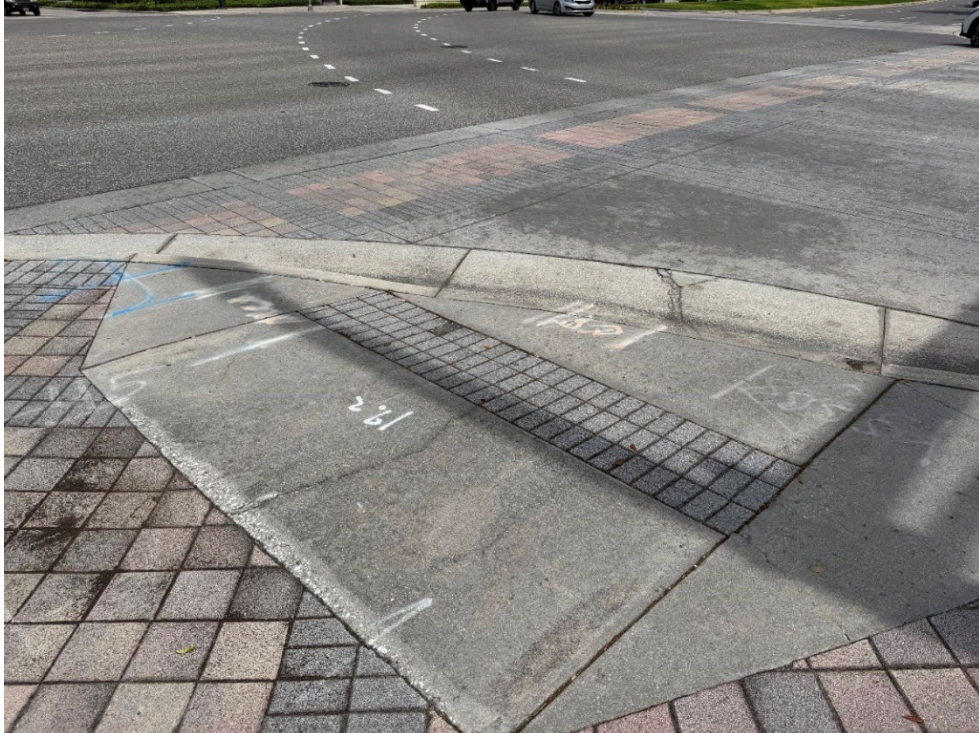
Photo 28 – Surficial Concrete Cracks in Handicap Ramp (No Observed Changes) (Refer to Prior Photo 35- 2025 Assessment)
