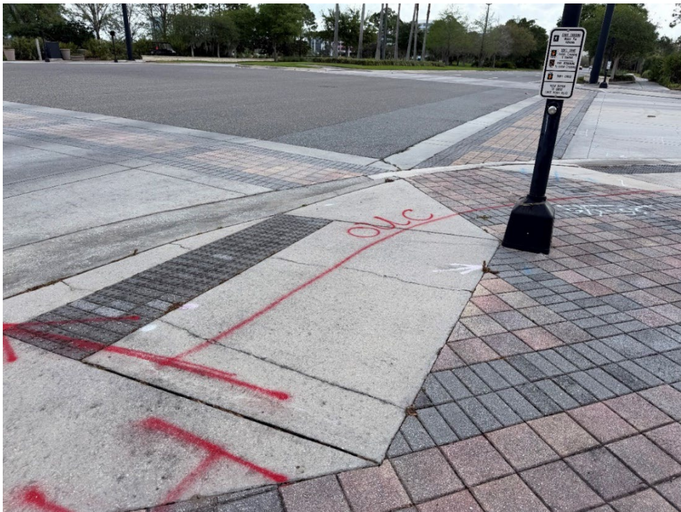
Photo 15 – Surficial Concrete Cracks in Handicap Ramp (No Observed Changes) (Refer to Prior Photo 18- 2025 Assessment)
