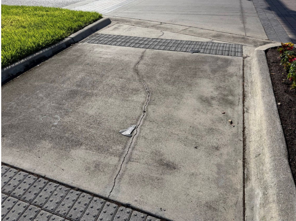
Photo 78.1 – Surficial Concrete Cracks in East Median (New Photo – 2026 Assessment)
