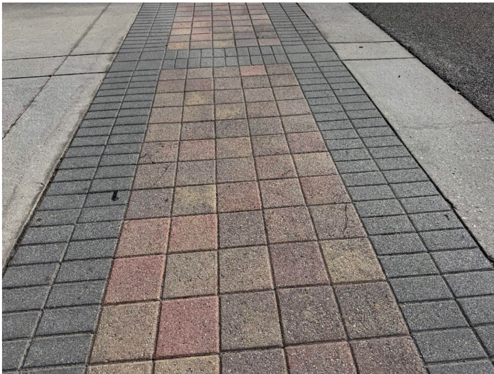
Photo 78 – Cracked Pavers, Minor Settling (No Observed Changes) (Refer to Prior Photo 102 - 2025 Assessment)
