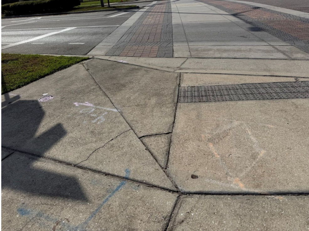
Photo 53.2 – Surficial Concrete Cracks in Handicap Ramp (New Photo – 2026 Assessment)
