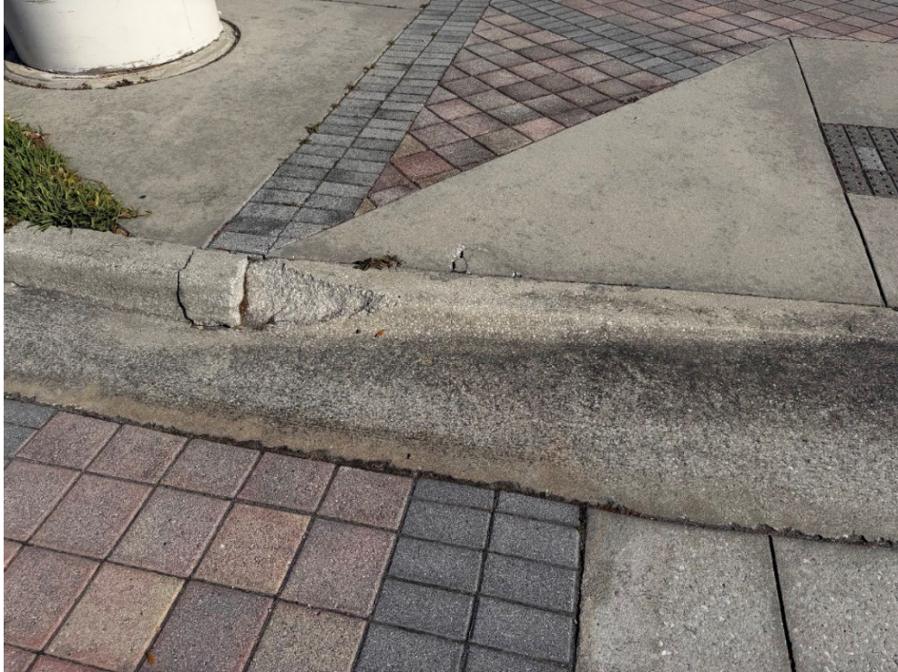
Photo 79.3 – Broken Curb (New Photo – 2026 Assessment)
