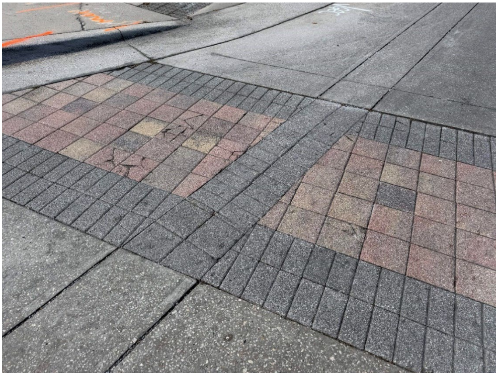
Photo 84.2 – Cracked Concrete, Multiple Cracked Pavers, Some Settling (New Photo – 2026 Assessment)
