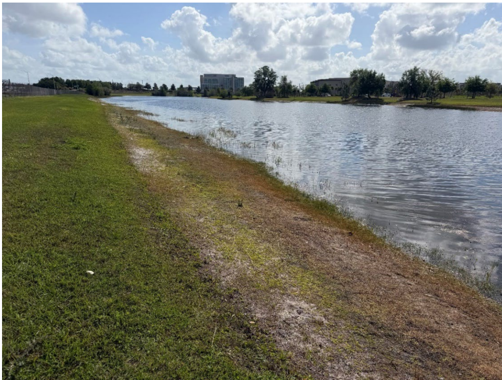
Photo 57 – Pond Berm Facing East in Good Condition (No Observed Changes) (Refer to Prior Photo 75- 2025 Assessment)
