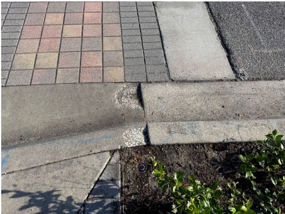
Photo 72.2 – Spalling Concrete, Settling (New Photo – 2026 Assessment)
