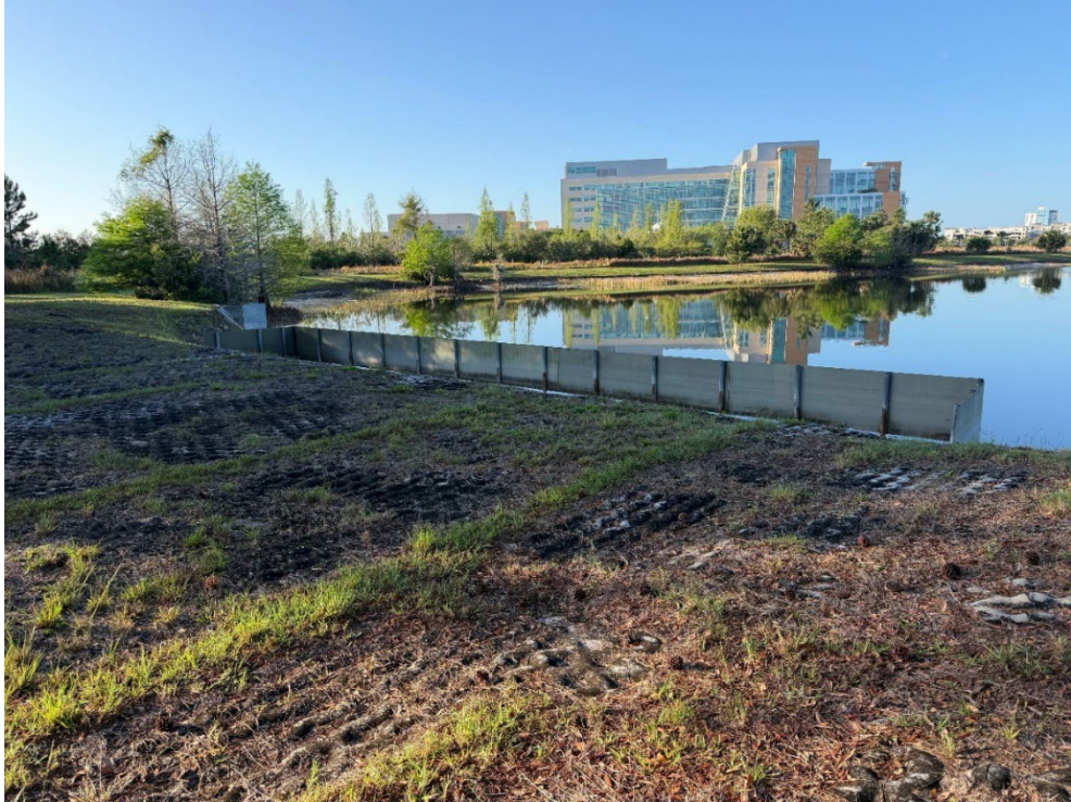
Photo 67 – Weir on NE Corner in Good Condition (No Observed Changes) (Refer to Prior Photo 87 - 2025 Assessment)
