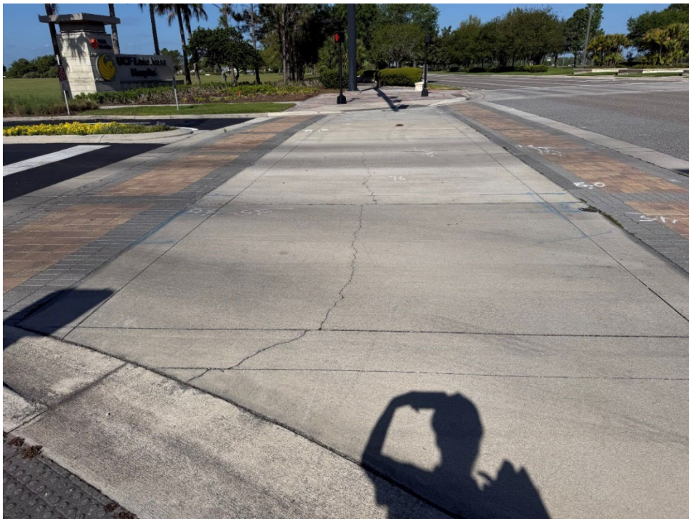
Photo 82 – Surficial Concrete Cracks, Multiple Cracked Pavers, Some Settling (No Observed Changes) (Refer to Prior Photo 109 - 2025 Assessment)
