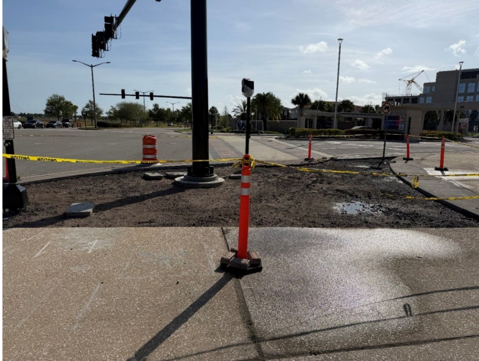
Photo 53 – Construction in All Quads at VA Hospital Intersection (Construction Continues) (Refer to Prior Photo 68- 2025 Assessment)
