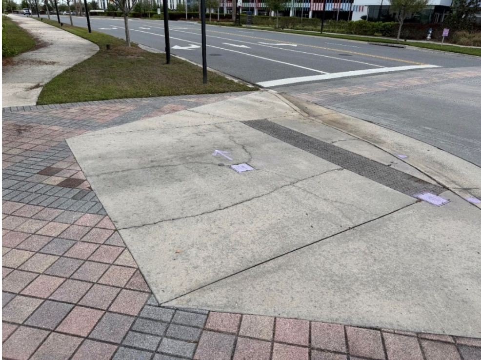
Photo 18 – Surficial Concrete Cracks in Handicap Ramp (No Observed Changes) (Refer to Prior Photo 22- 2025 Assessment)
