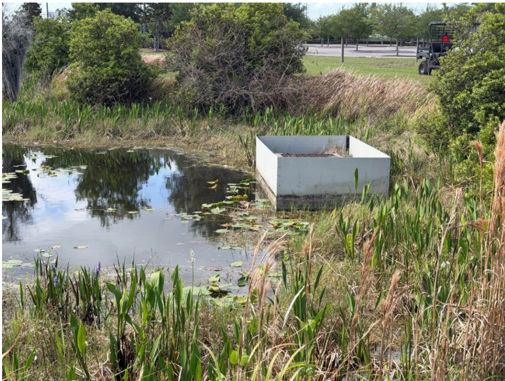
Photo 61.3 – Outfall Structure Containing Vegetation (New Photo – 2026 Assessment)
