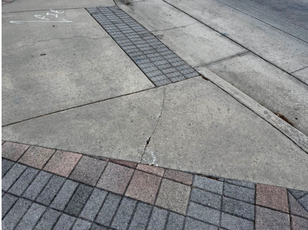
Photo 34 – Surficial Concrete Cracks in Handicap Ramp (No Observed Changes) (Refer to Prior Photo 41- 2025 Assessment)
