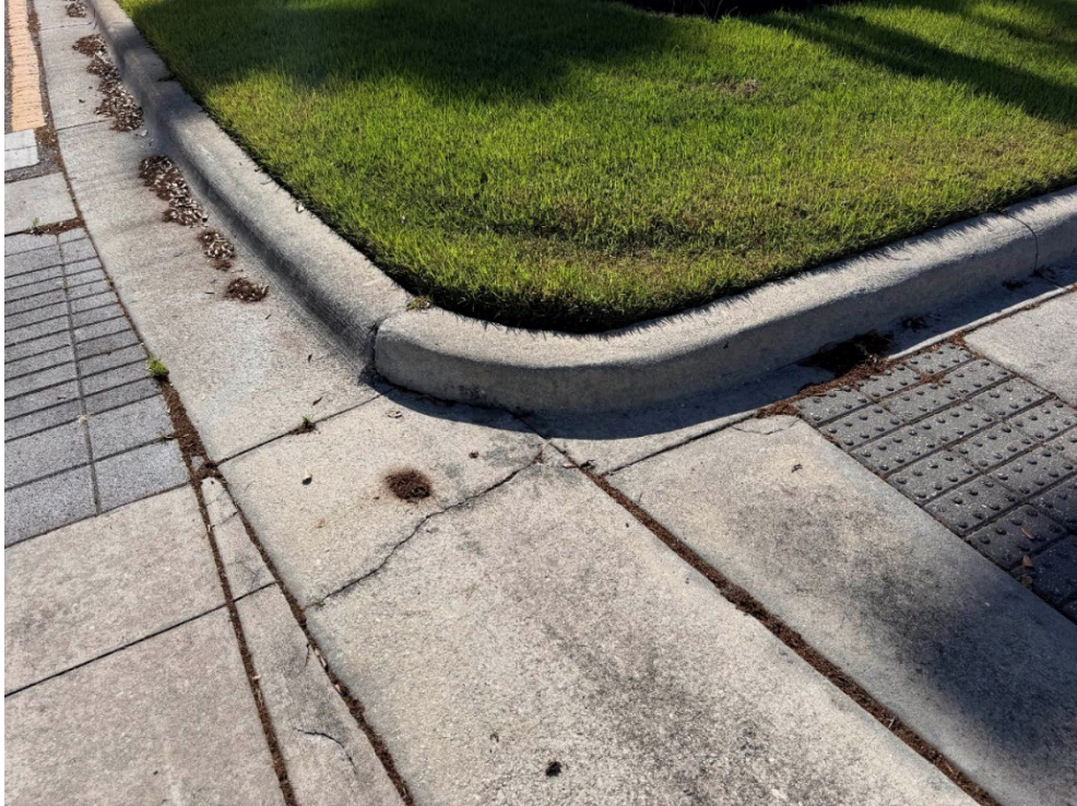
Photo 84.1 – Surficial Cracks in Concrete (New Photo – 2026 Assessment)
