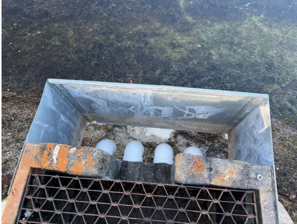
Photo 69 – Drawdown Pipe Inside of Outfall Structure (No Observed Changes) (Refer to Prior Photo 89- 2025 Assessment)
