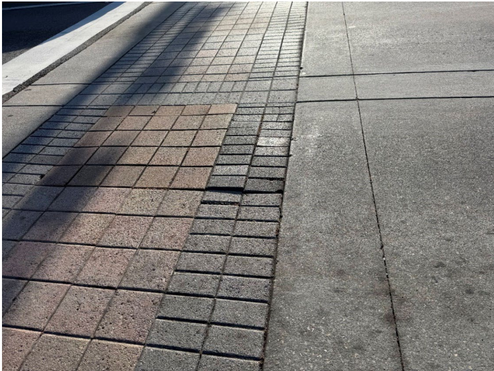
Photo 72 – Surficial Paver Cracks, Minor Settling (No Observed Changes) (Refer to Prior Photo 92- 2025 Assessment)
