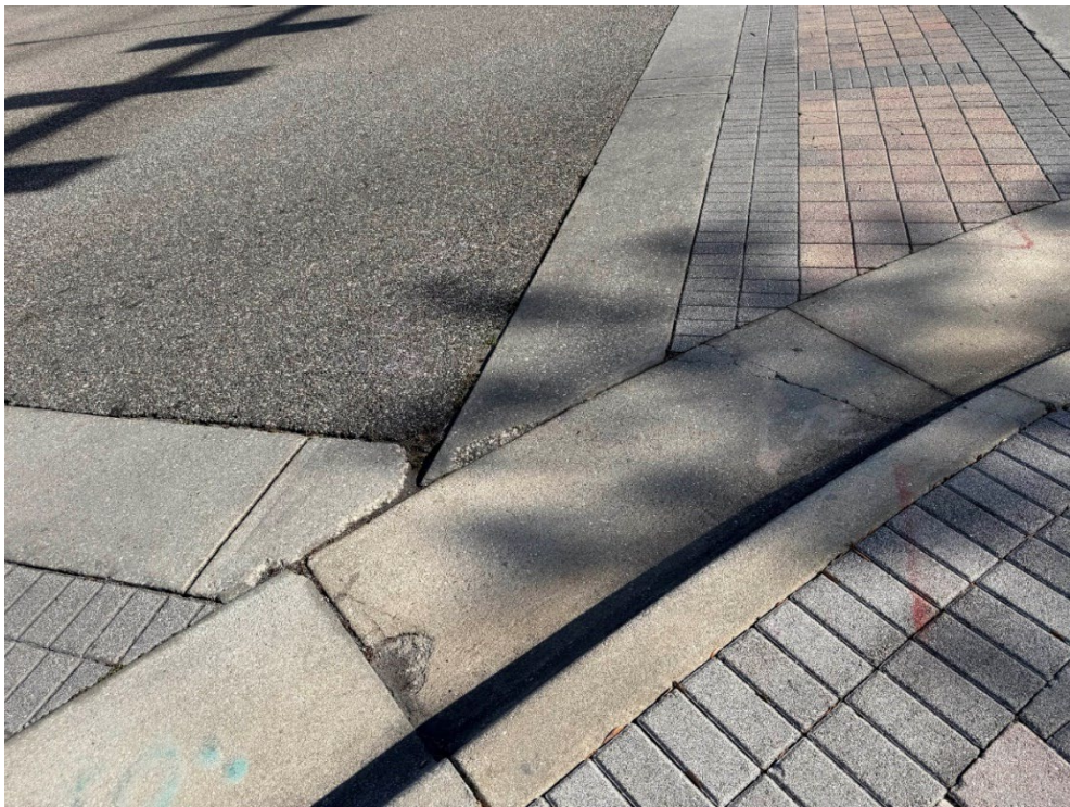
Photo 75.1 – Broken Concrete Ribbon (New Photo – 2026 Assessment)
