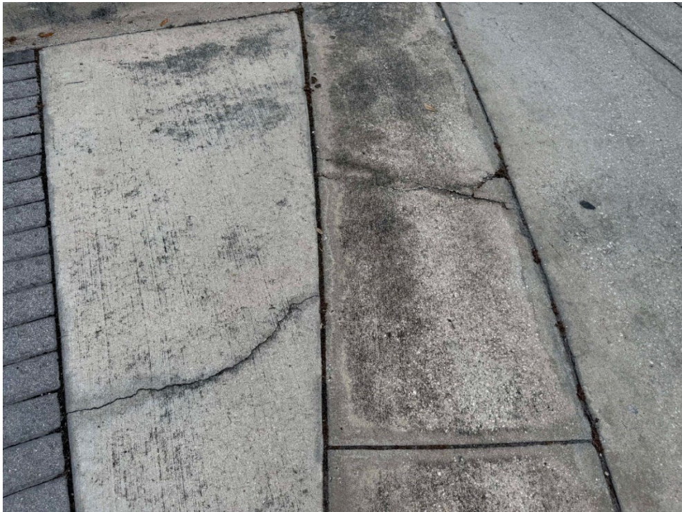
Photo 31 – Surficial Concrete Cracks in Median Strip (No Observed Changes) (Refer to Prior Photo 38- 2025 Assessment)
