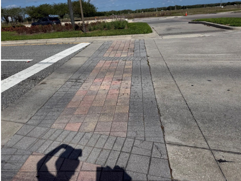
Photo 84.3 – Multiple Cracked Concrete, Pavers Settling, Broken Flush Curb (New Photo – 2026 Assessment)
