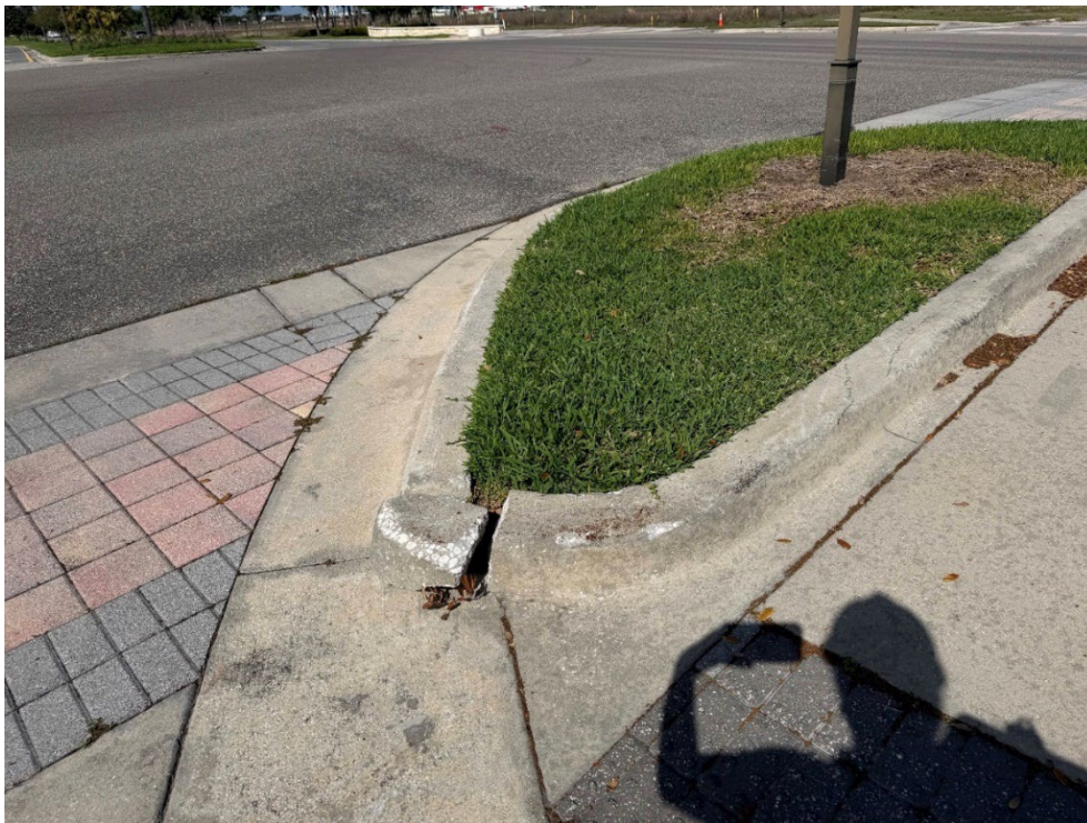
Photo 86 – Broken Curb (No Observed Changes) (Refer to Prior Photo 116 - 2025 Assessment)
