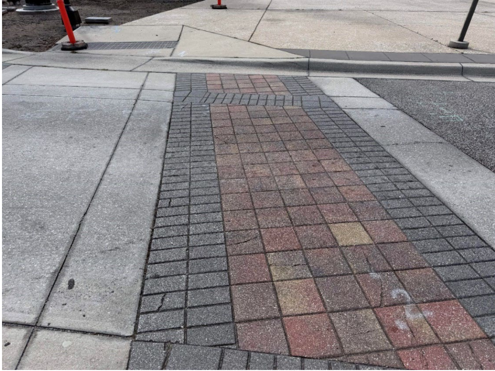
Photo 90.1 – Cracked Pavers (New Photo – 2026 Assessment)
