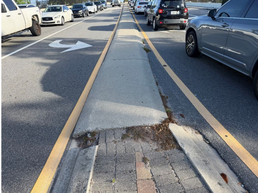
Photo 47 – Paver Base Failure in North Median Looking North (No Observed Changes) (Refer to Prior Photo 57- 2025 Assessment)
