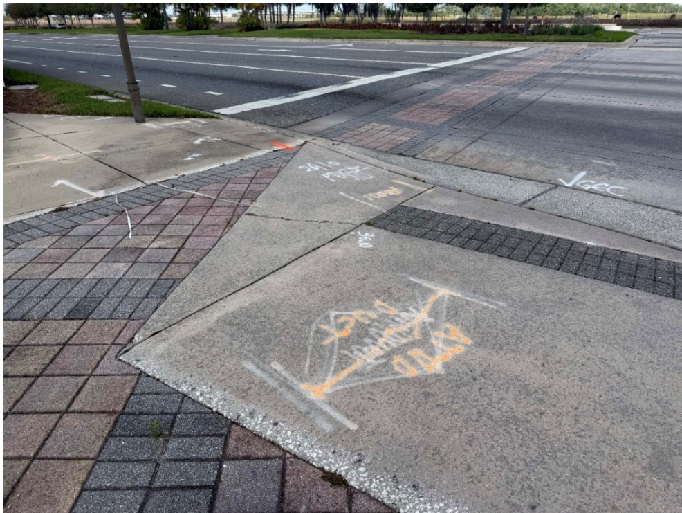
Photo 11 – Surficial Concrete Cracks in Handicap Ramp (No Observed Changes) (Refer to Prior Photo 14- 2025 Assessment)
