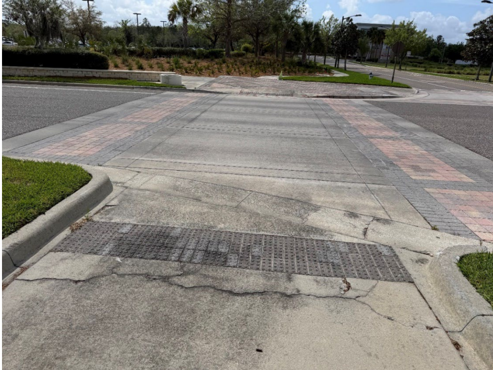
Photo 22 – Surficial Concrete Cracks in Handicap Ramp (No Observed Changes) (Refer to Prior Photo 29- 2025 Assessment)
