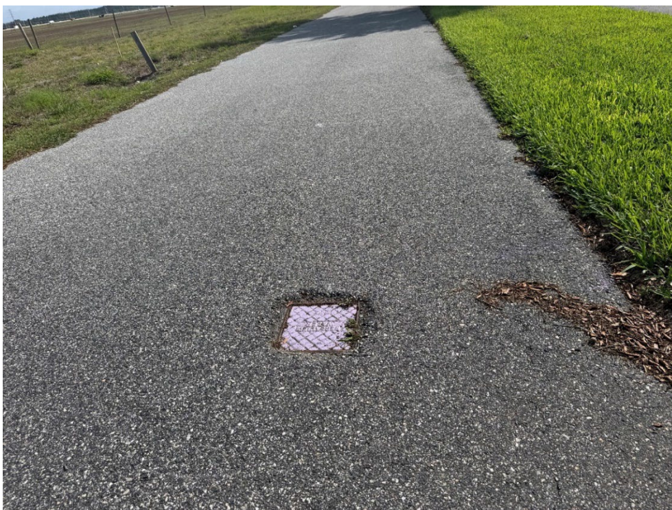
Photo 9 – Sunken Reclaim Water Meter (No Observed Changes) (Refer to Prior Photo 12- 2025 Assessment)
