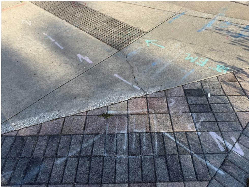
Photo 42 – Surficial Concrete Cracks in Handicap Ramp (No Observed Changes) (Refer to Prior Photo 51- 2025 Assessment)
