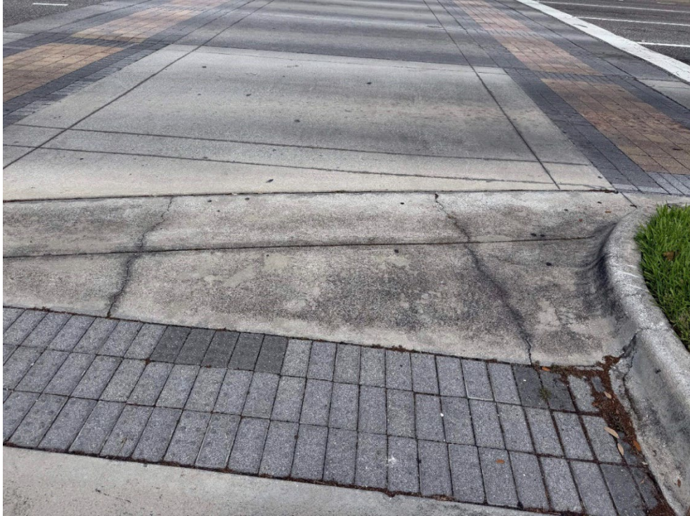
Photo 30 – Surficial Concrete Cracks in Median Strip (No Observed Changes) (Refer to Prior Photo 37- 2025 Assessment)
