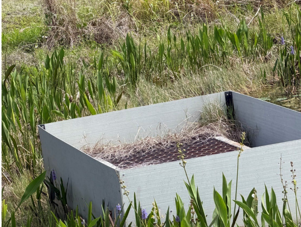
Photo 61.4 – Outfall Structure Containing Vegetation (New Photo – 2026 Assessment)
