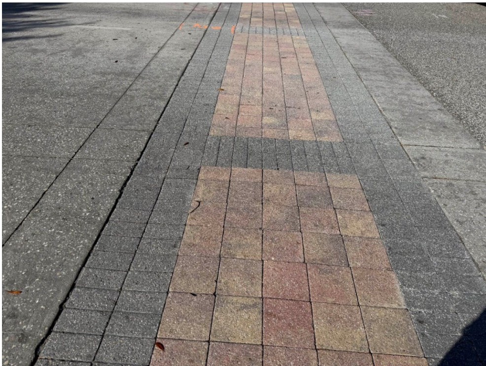
Photo 76.1 – Cracked Pavers (New Photo – 2026 Assessment)
