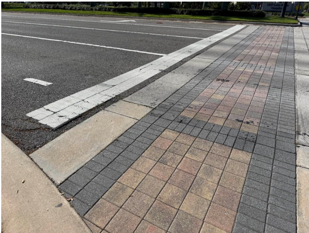
Photo 84 – Broken Concrete Flush Curb (No Observed Changes) (Refer to Prior Photo 111 - 2025 Assessment)
