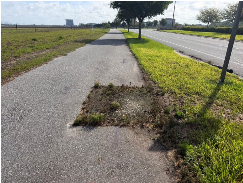
Photo 7 – Asphalt Cutout and Removed (No Observed Changes) (Refer to Prior Photo 9- 2025 Assessment)
