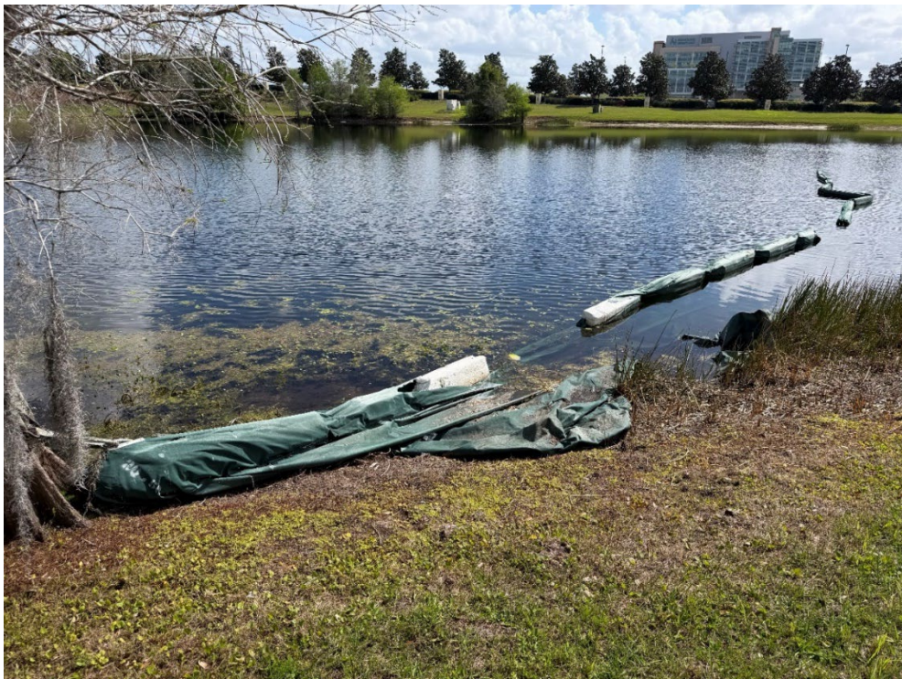
Photo 60 – Detached and Broken Floating Turbidity Barrier (No Observed Changes) (Refer to Prior Photo 79- 2025 Assessment)
