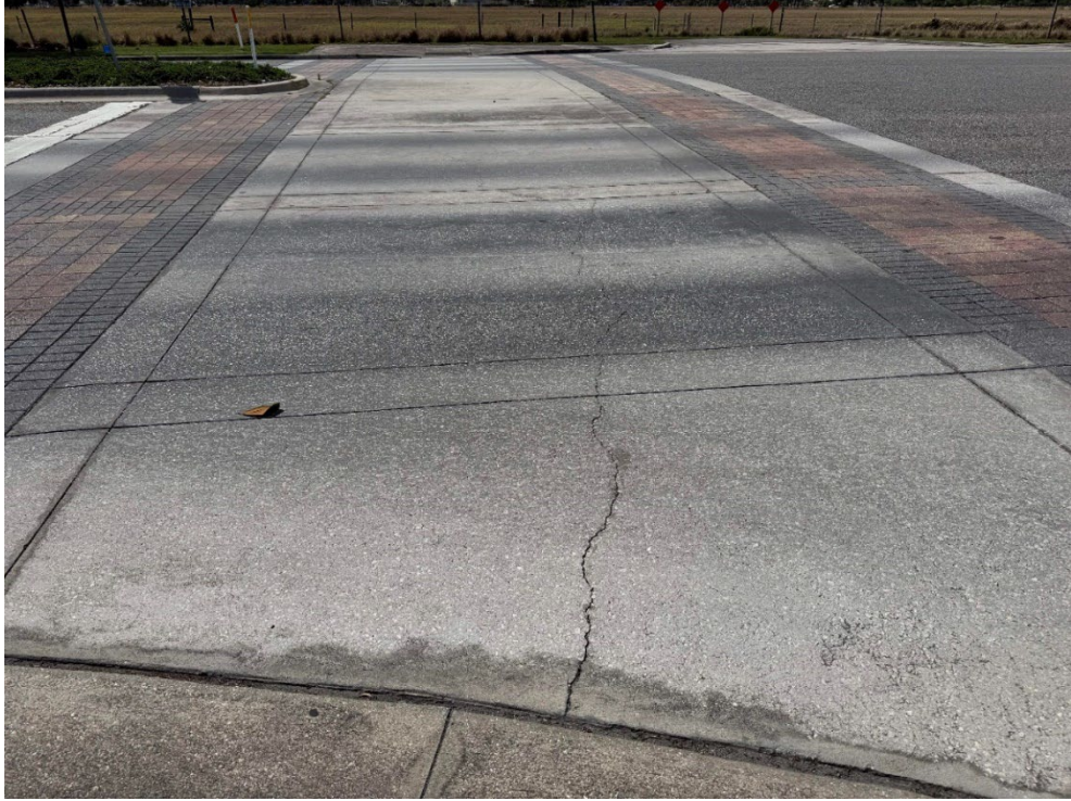
Photo 92 – Surficial Concrete Cracks (No Observed Changes) (Refer to Prior Photo 125 - 2025 Assessment)
