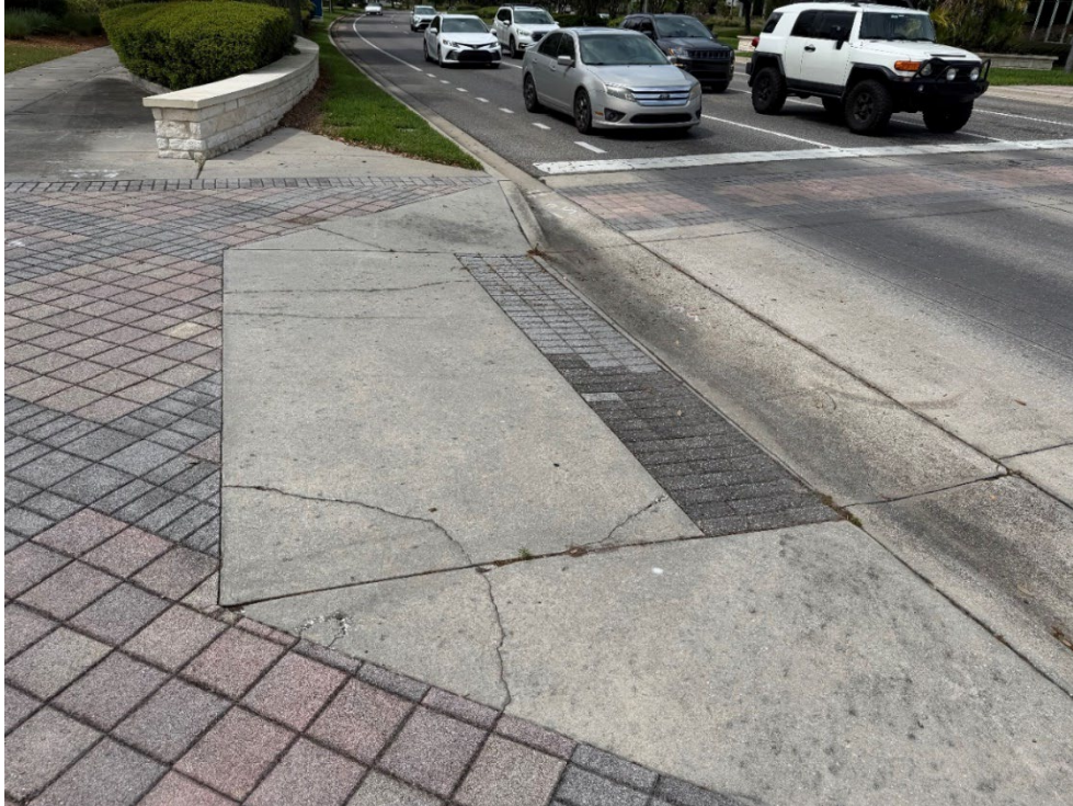
Photo 26 – Surficial Concrete Cracks in Handicap Ramp (No Observed Changes) (Refer to Prior Photo 33- 2025 Assessment)
