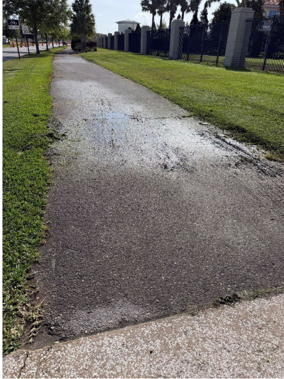
Photo 52.1 – Poor Drainage on Sidewalk (New Photo – 2026 Assessment)
