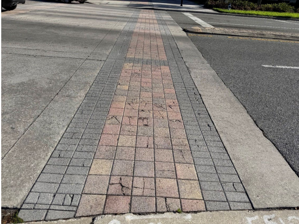
Photo 75 – Cracked Pavers (No Observed Changes) (Refer to Prior Photo 97 - 2025 Assessment)
