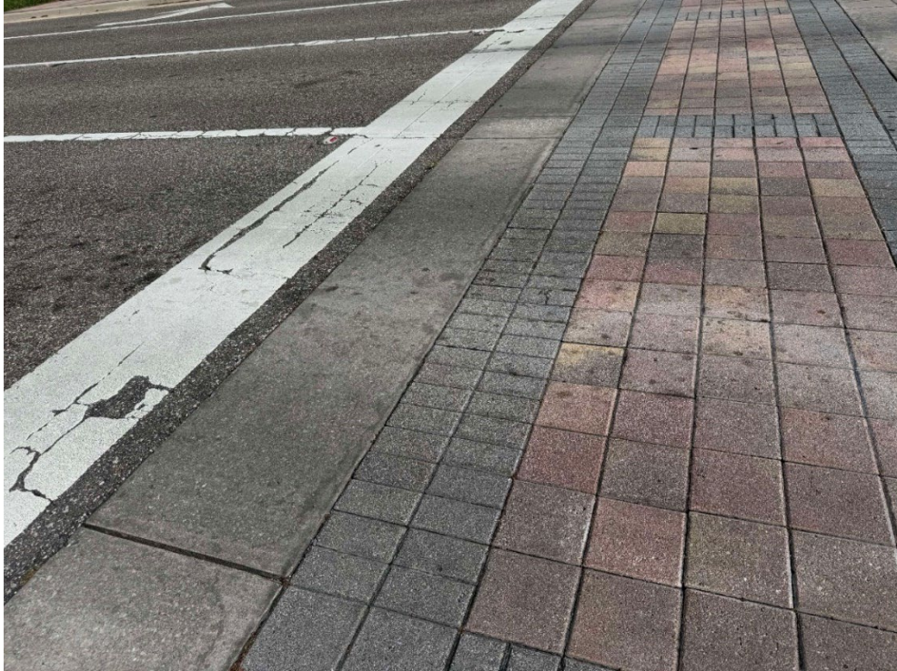
Photo 83 – Cracked Pavers, Some Settling (No Observed Changes) (Refer to Prior Photo 110 - 2025 Assessment)
