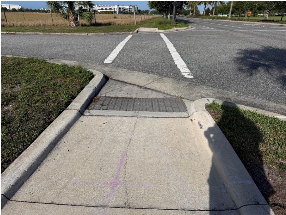
Photo 50 – Surficial Concrete Cracks in Handicap Ramp (No Observed Changes) (Refer to Prior Photo 61 and 62- 2025 Assessment)
