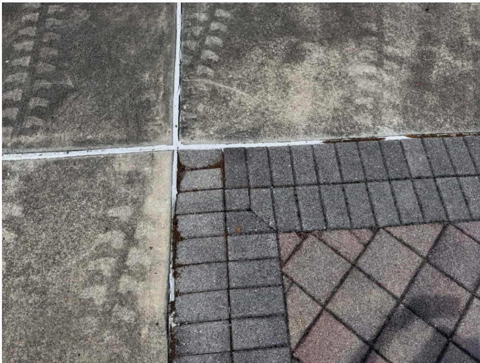
Photo 27 – Paver Base Failure (No Observed Changes) (Refer to Prior Photo 34- 2025 Assessment)
