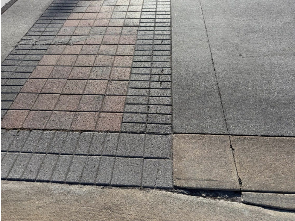
Photo 71 – Cracked Pavers, Minor Settling (No Observed Changes) (Refer to Prior Photo 91- 2025 Assessment)
