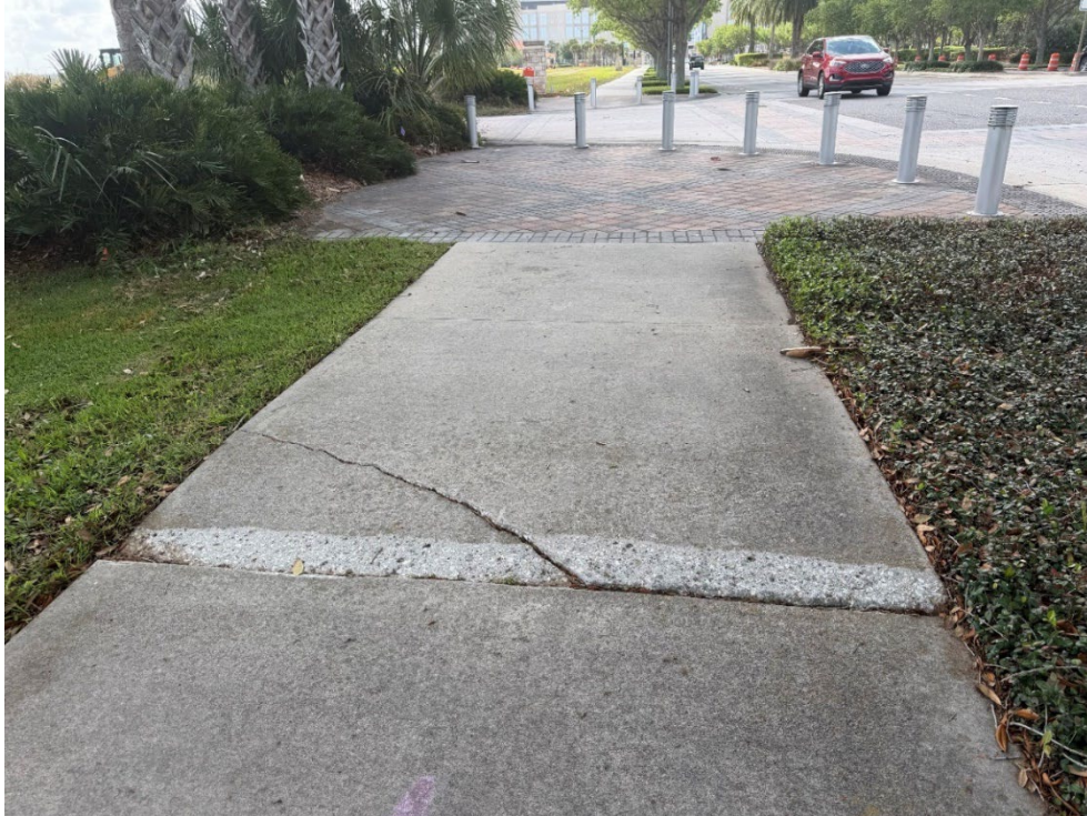
Photo 54.1 – Concrete Crack in Uneven Sidewalk (New Photo – 2026 Assessment)
