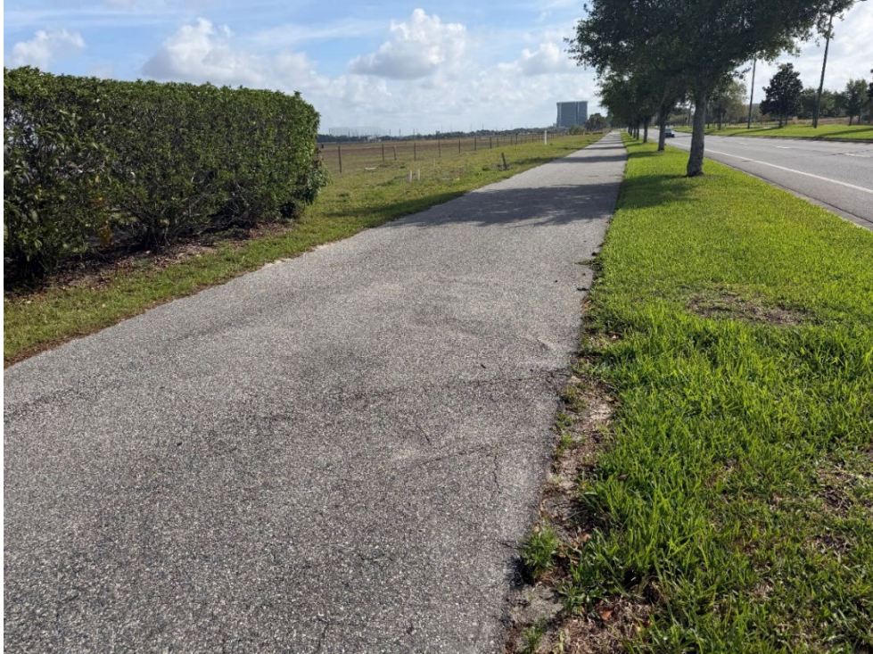
Photo 8 – Raveling Asphalt with Depression and Base Failure (No Observed Changes) (Refer to Prior Photo 11- 2025 Assessment)
