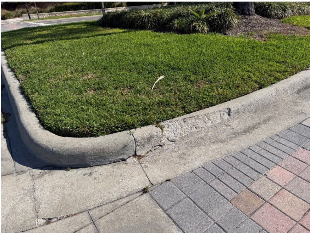
Photo 80 – Broken Curb (No Observed Changes) (Refer to Prior Photo 107 - 2025 Assessment)
