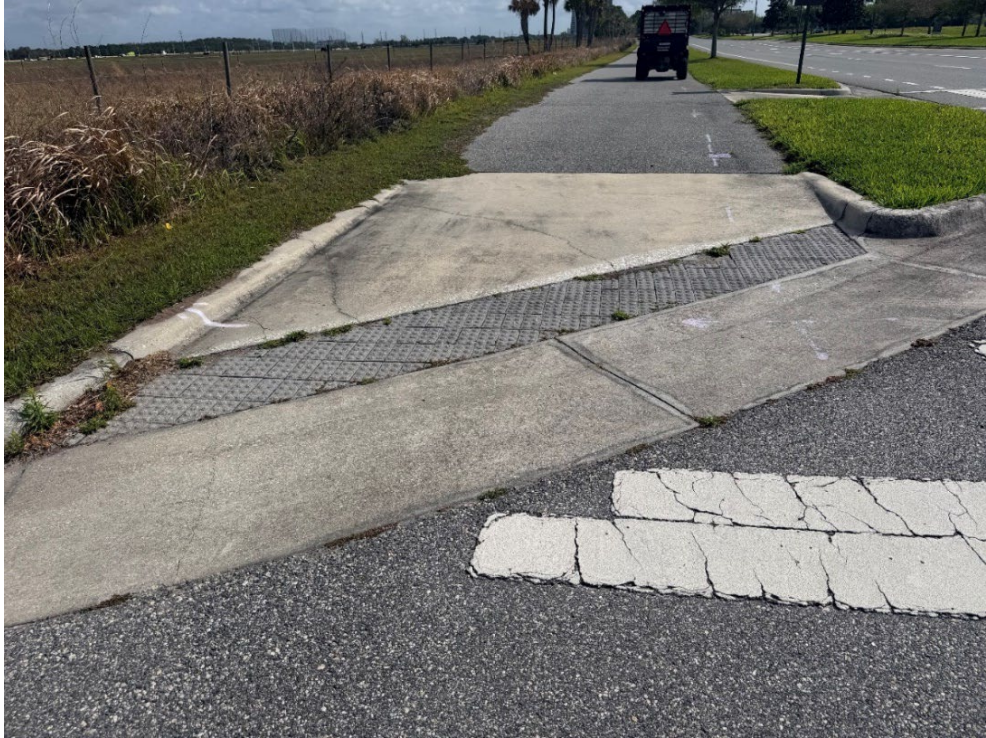
Photo 10 – Surficial Concrete Cracks in Handicap Ramp (No Observed Changes) (Refer to Prior Photo 13- 2025 Assessment)
