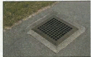
12" CATCH BASIN IN TRAIL ASPHALT
