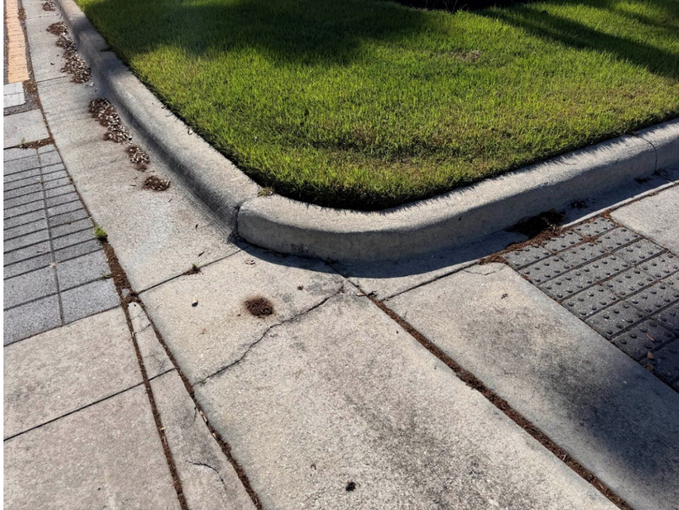
Photo 84.1 – Surficial Cracks in Concrete (New Photo – 2026 Assessment)
