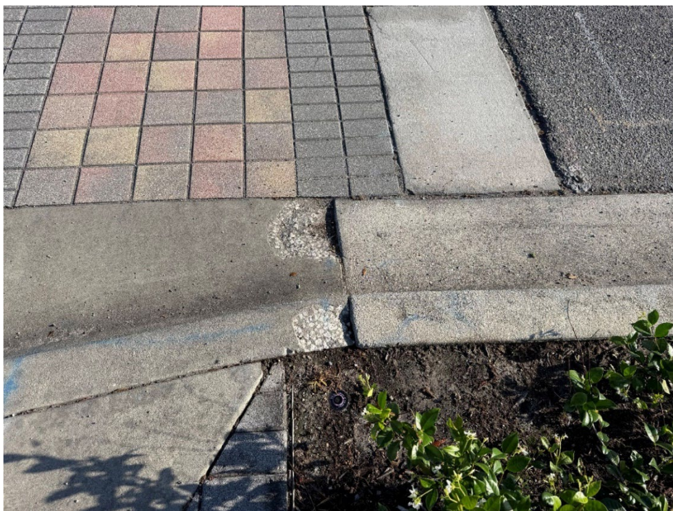
Photo 72.2 – Spalling Concrete, Settling (New Photo – 2026 Assessment)
