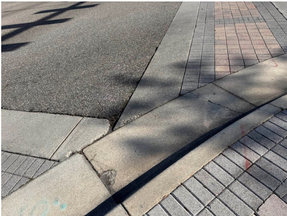
Photo 75.1 – Broken Concrete Ribbon (New Photo – 2026 Assessment)
