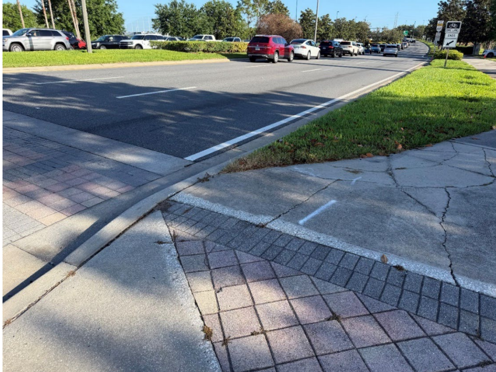
Photo 72.1 – Cracked Concrete, Minor Settling (New Photo – 2026 Assessment)
