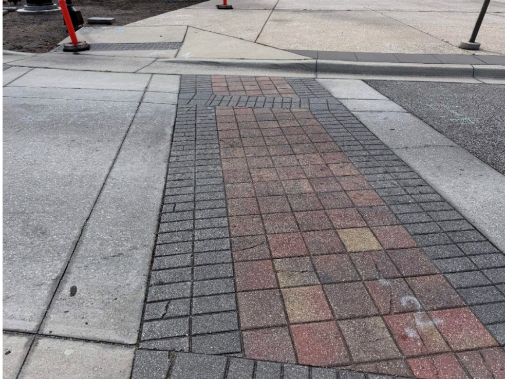
Photo 90.1 – Cracked Pavers (New Photo – 2026 Assessment)
