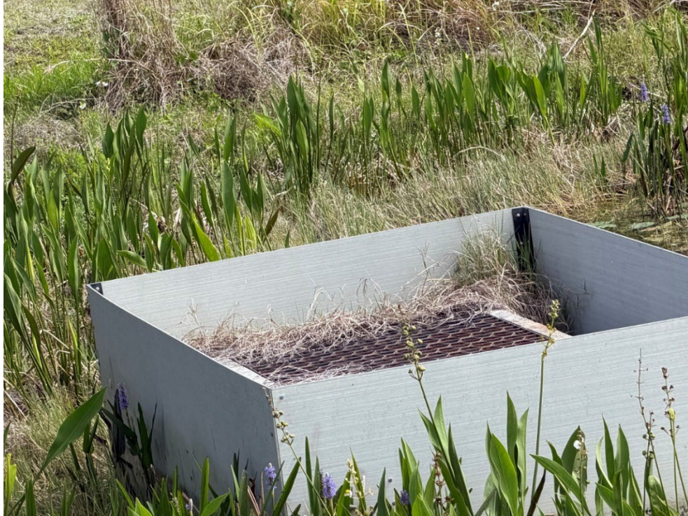
Photo 61.4 – Outfall Structure Containing Vegetation (New Photo – 2026 Assessment)
