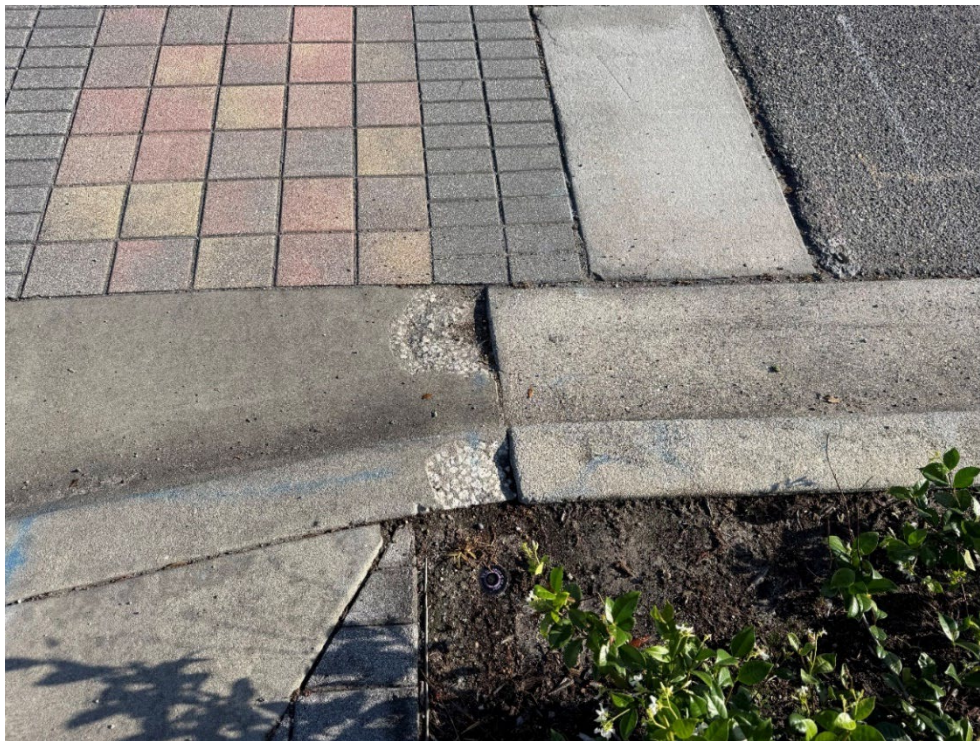
Photo 72.2 – Spalling Concrete, Settling (New Photo – 2026 Assessment)
