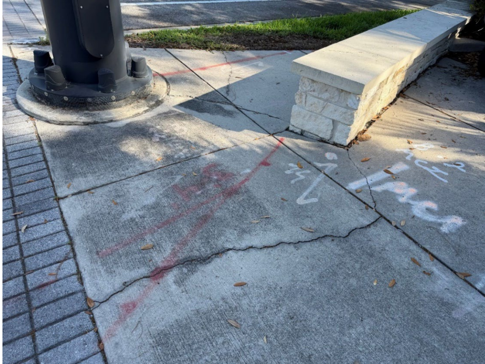
Photo 78.3 – Cracked Concrete in Sidewalk (New Photo – 2026 Assessment)
