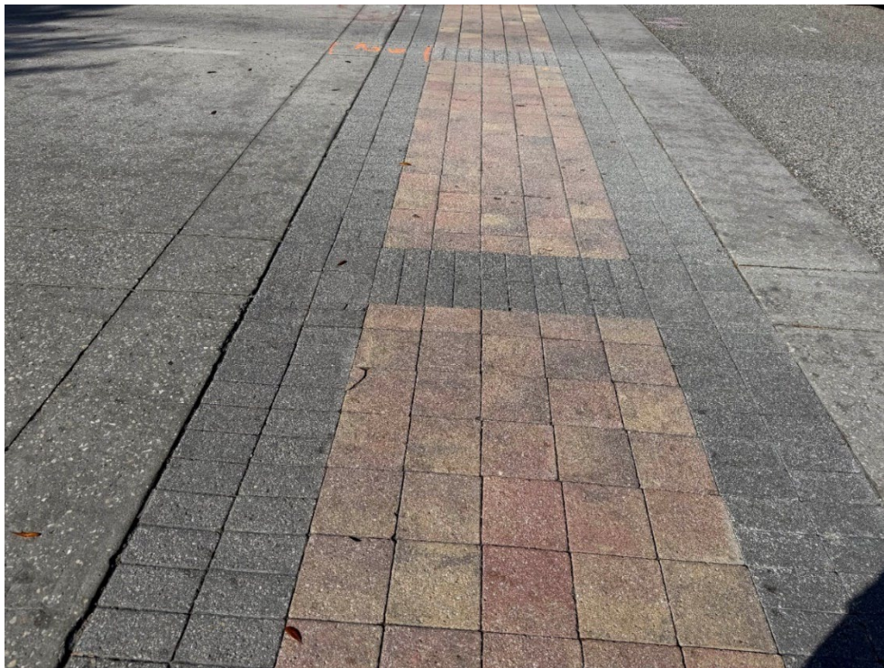
Photo 76.1 – Cracked Pavers (New Photo – 2026 Assessment)
