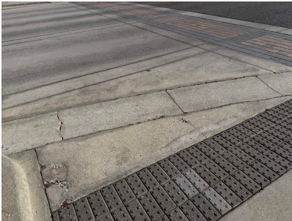
Photo 79.2 – Broken and Spalling Concrete (New Photo – 2026 Assessment)
