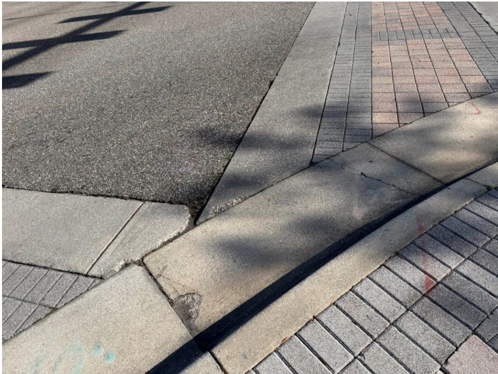
Photo 75.1 – Broken Concrete Ribbon (New Photo – 2026 Assessment)
