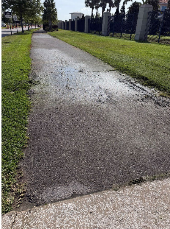
Photo 52.1 – Poor Drainage on Sidewalk (New Photo – 2026 Assessment)
