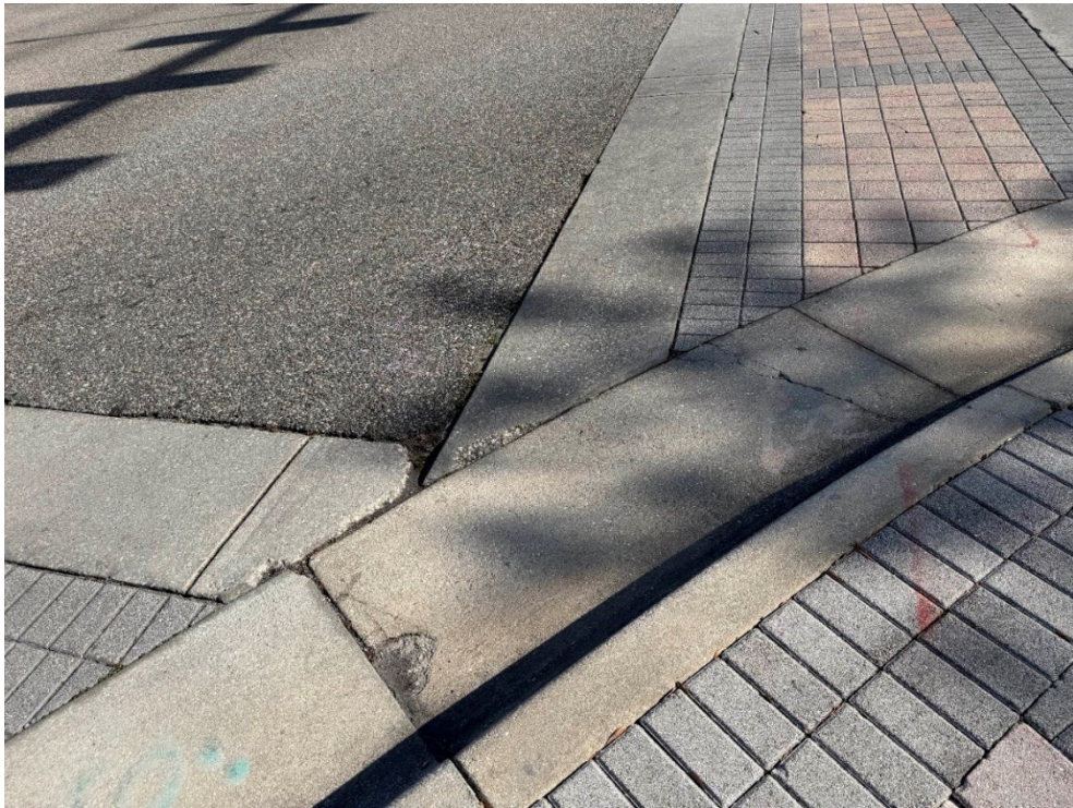
Photo 75.1 – Broken Concrete Ribbon (New Photo – 2026 Assessment)
