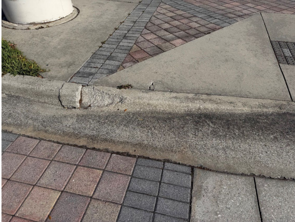
Photo 79.3 – Broken Curb (New Photo – 2026 Assessment)
