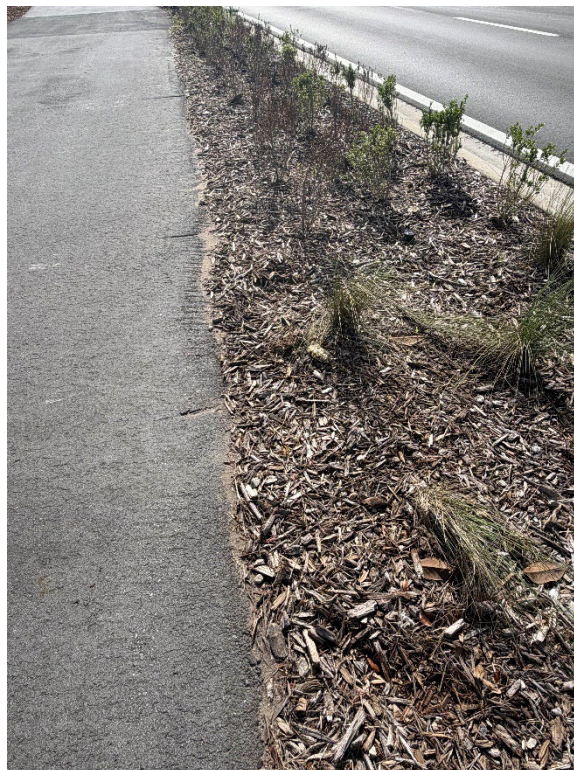
Photo 5.1 – Damaged Asphalt (New Photo – 2026 Assessment)
