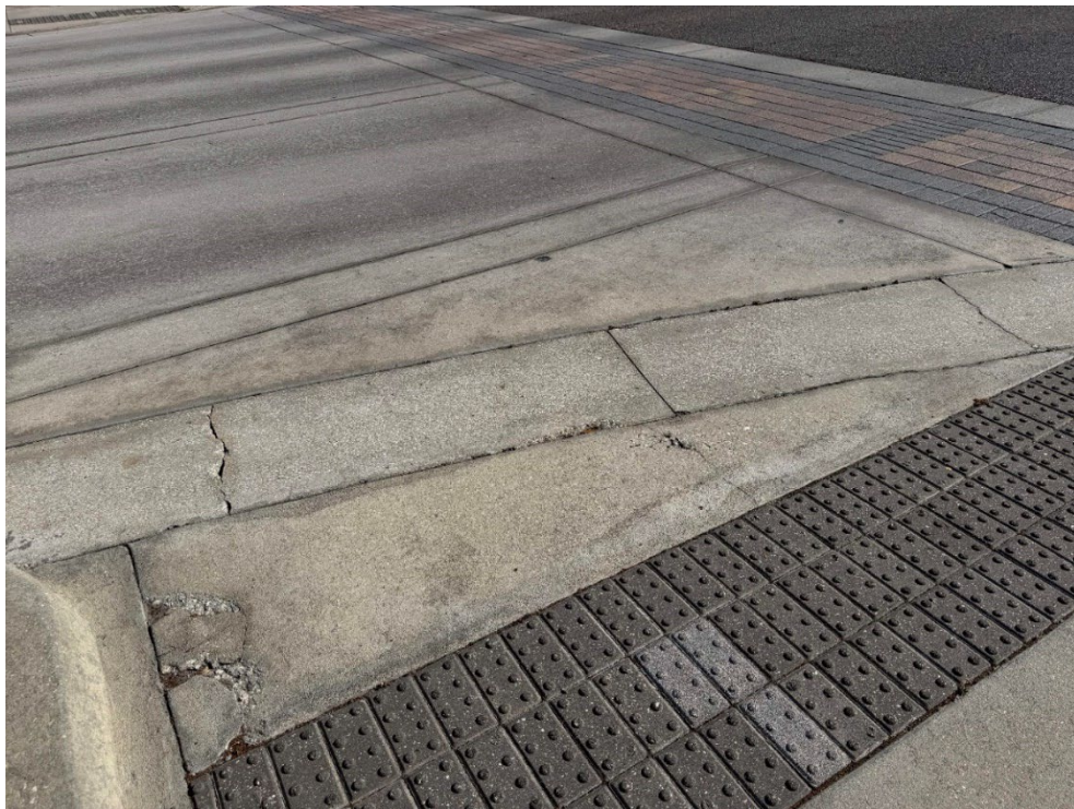
Photo 79.2 – Broken and Spalling Concrete (New Photo – 2026 Assessment)
