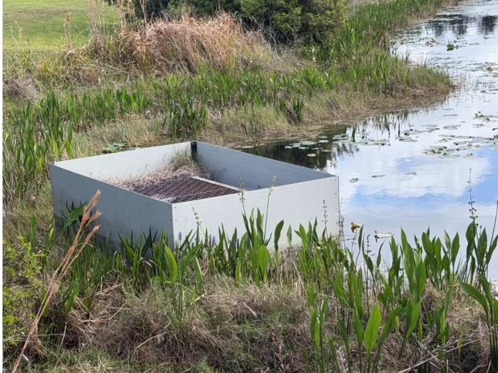
Photo 61.2 – Outfall Structure Containing Vegetation (New Photo – 2026 Assessment)
