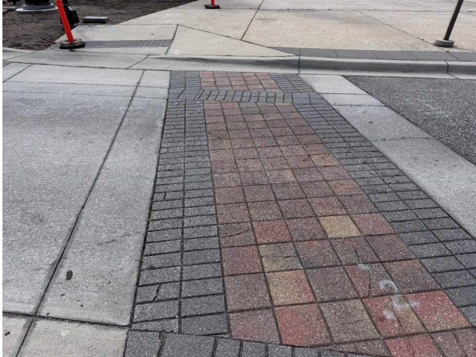
Photo 90.1 – Cracked Pavers (New Photo – 2026 Assessment)
