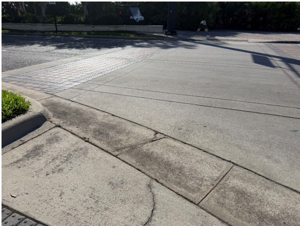
Photo 78.2 – Cracked Concrete (New Photo – 2026 Assessment)
