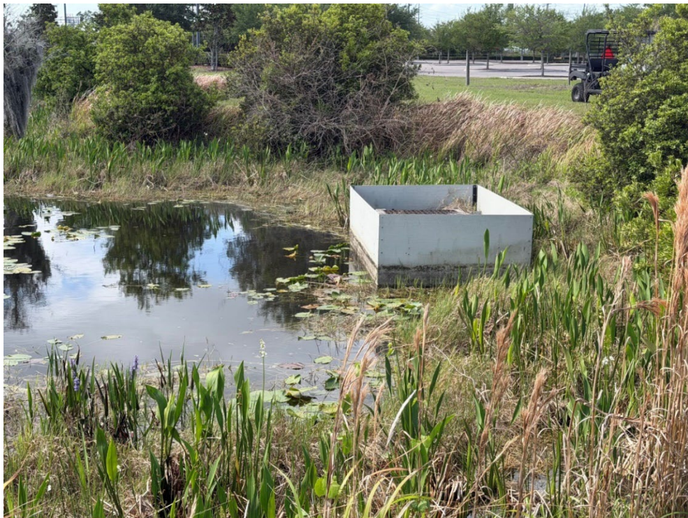
Photo 61.3 – Outfall Structure Containing Vegetation (New Photo – 2026 Assessment)
